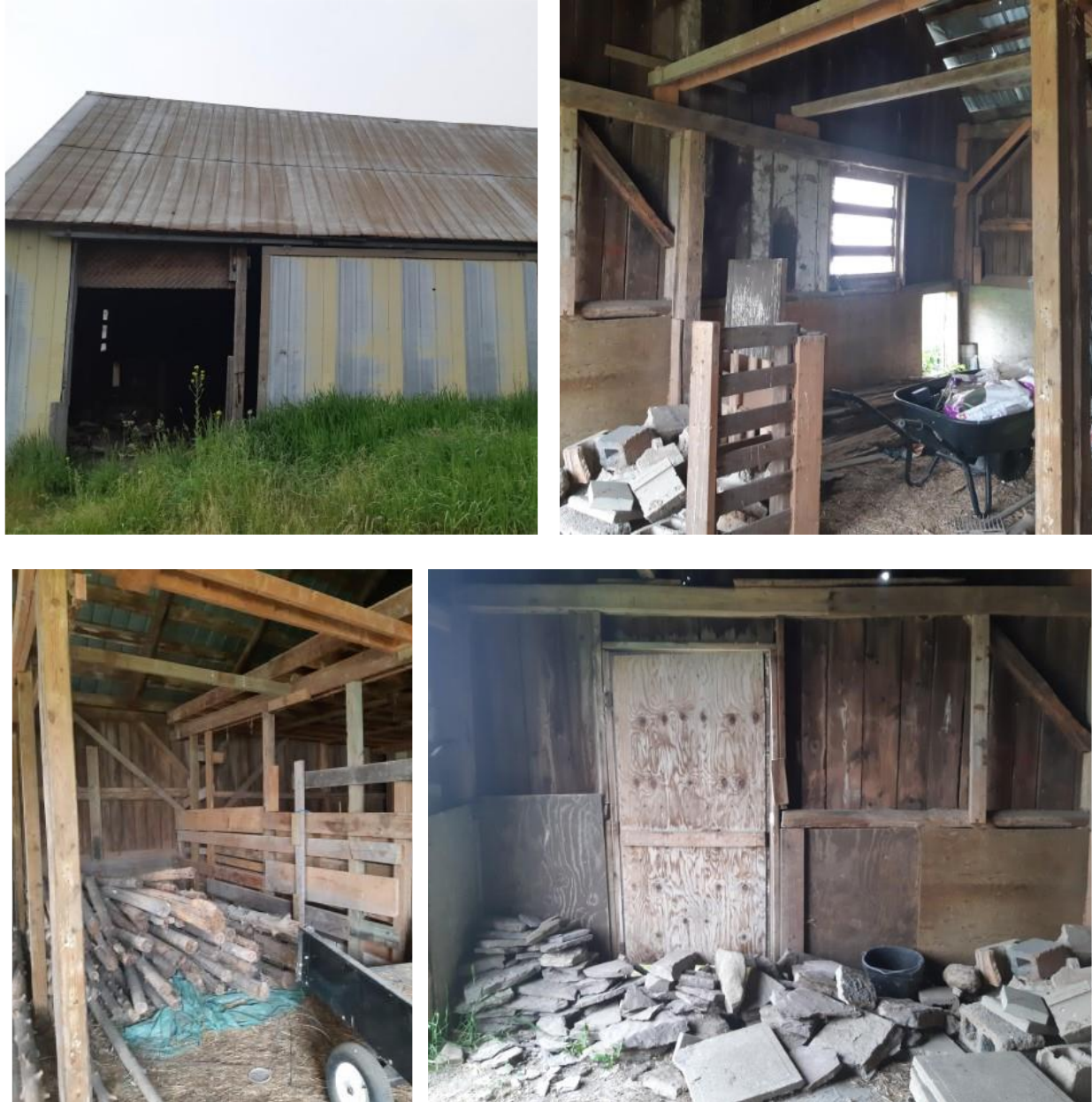
Figure 2: The exterior and interior of the vacant barn on the Subject Site (Novatech, June 2023).
