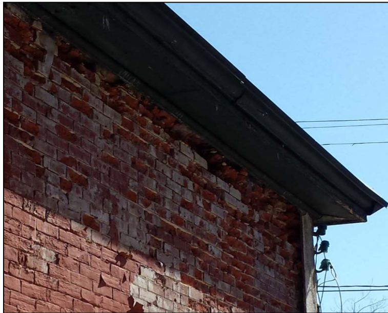
Image 2: Spalling of Brick Veneer Fascia on South Wall of 201 Wilbrod St.
