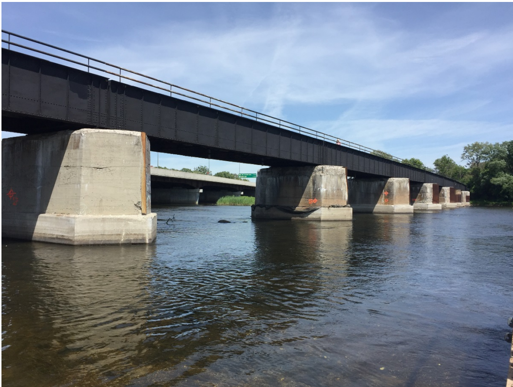
Photo 42 – South elevation of the exterior girders webs; coating in generally good condition.
