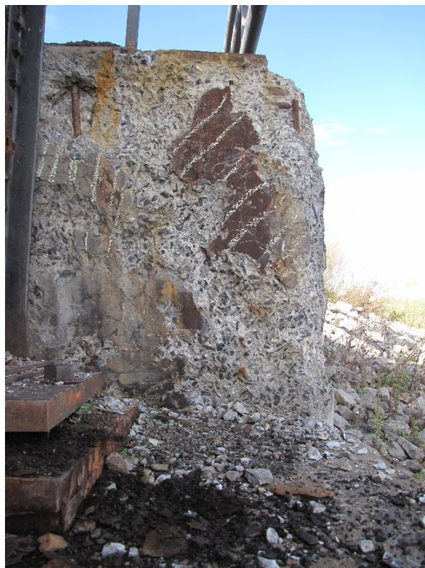
Photo 53 – Severe to very severe disintegration and delamination with exposed corroded rebar on the north end of the ballast wall.
