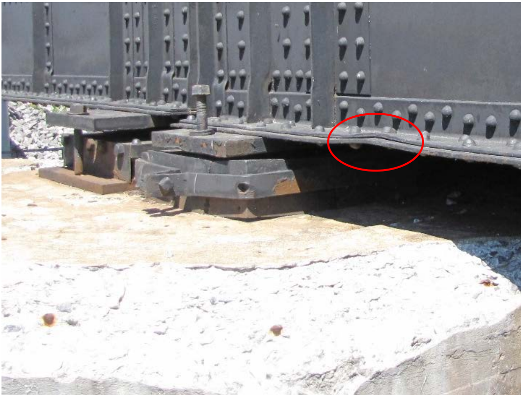
Photo 46 – Southeast bearing on Pier 7 is cracked and was previously temporarily repaired with a clamping device. Note the deformation on the bottom flange of the south girder.
