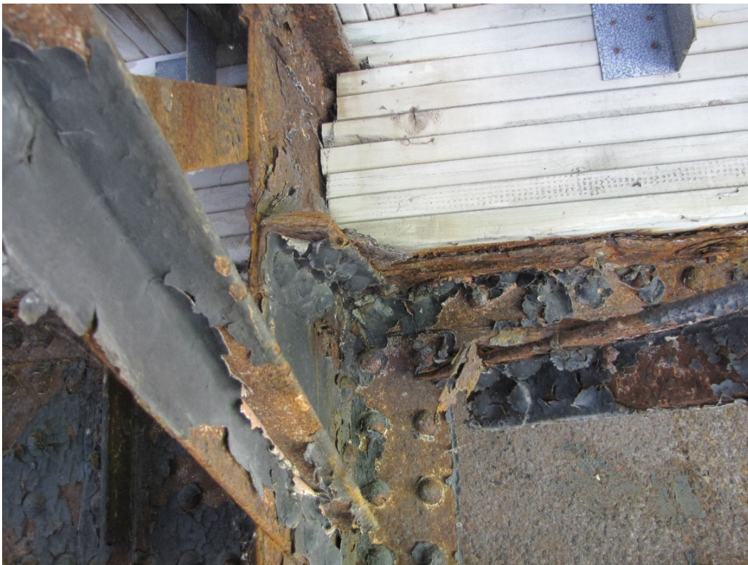
Photo 40 – Very severe corrosion on the horizontal gusset plate and lateral brace at the cross-frame in the bay just west of Pier 6, resulting in detachment of the lateral brace.
