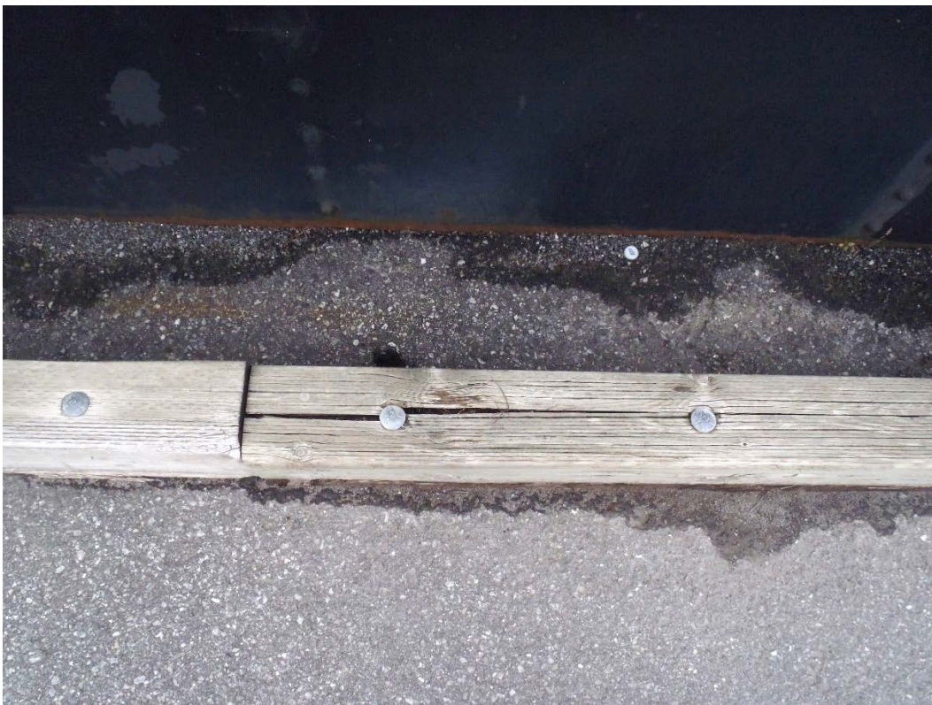
Photo 14 – Light to severe longitudinal splits in the curb from the bolts. Typical localized light weathering is also visible in the top and interior face of curb.
