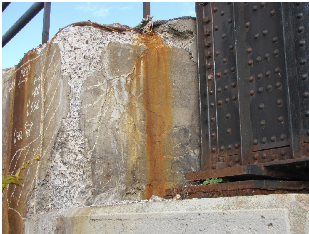
Photo 54 – Severe to very severe disintegration and delaminations with exposed corroded rebar at the south end of the ballast wall and southwest wingwall.
