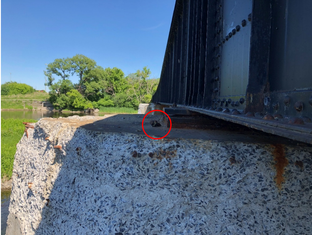
Photo 47 – Northwest bearing anchor bolt on Pier 4 has sheared off. Note the extensive concrete disintegration with exposed corroded reinforcing steel at the top of the pier shaft and bearing seat.
