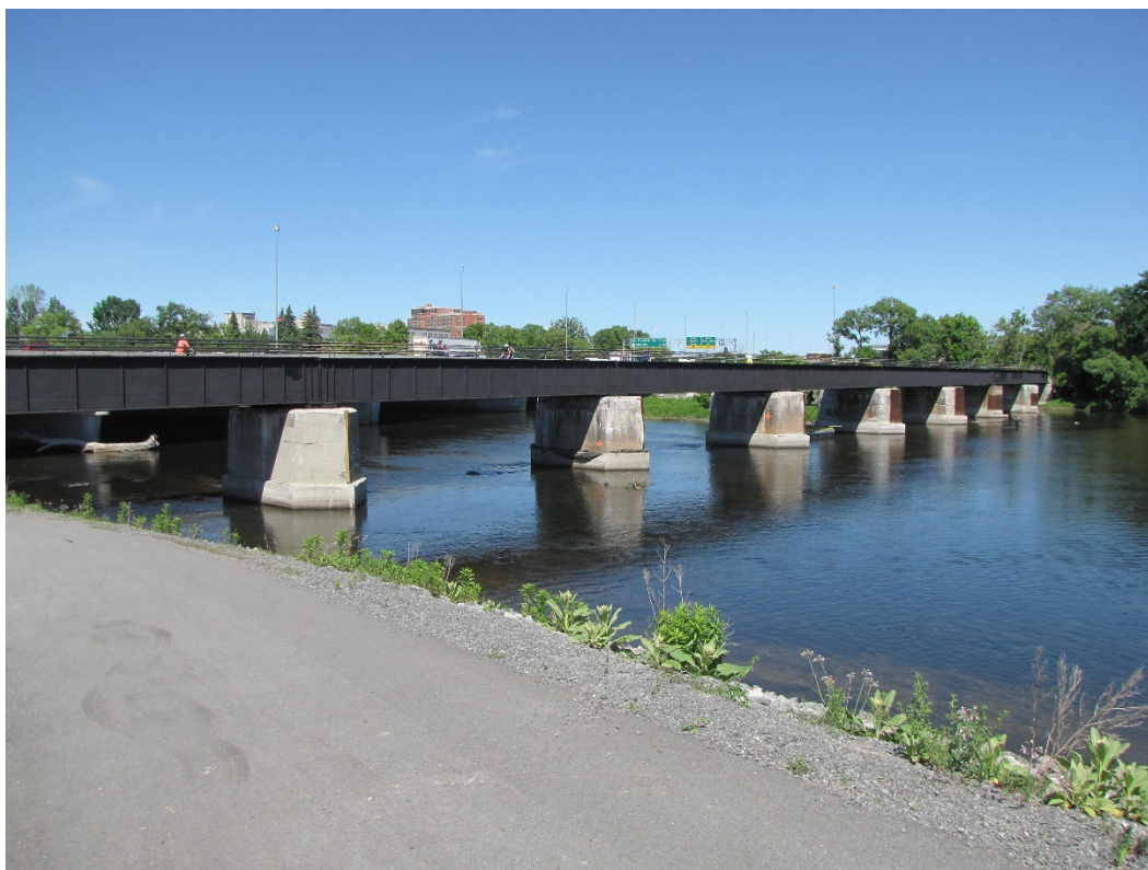
Photo 2 – South elevation. Note Rideau River Western Pathway (foreground), which passes below Span 8.
