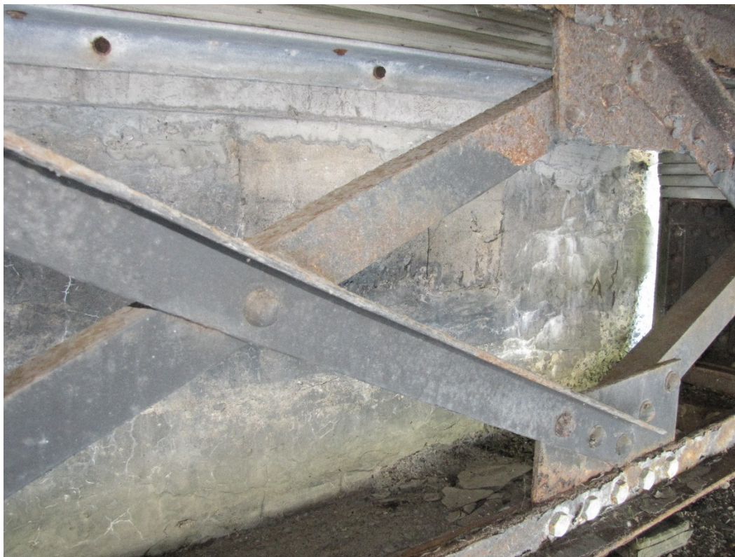
Photo 57 – Hairline to narrow wet and efflorescence stained map cracking in the east ballast wall.
