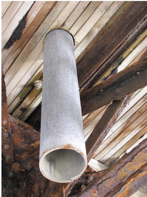
Photo 20 – Typical good condition of the deck drain downsouts with light corrosion on ends.
