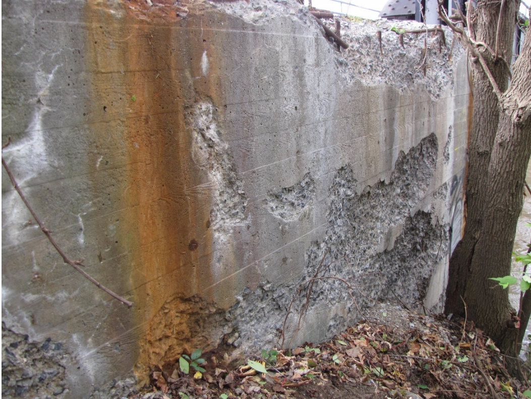
Photo 59 – Extensive areas of medium to very severe disintegration with exposed corroded rebar and hairline to narrow wet and efflorescence stained map cracking on the northeast wingwall.
