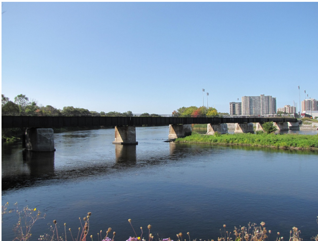
Photo 1 – North elevation of the Old Railway Rideau River Pedestrian Bridge. Note low-lying island downstream of Pier 5 and University of Ottawa (Lees Campus) located on west side of the river (background).
