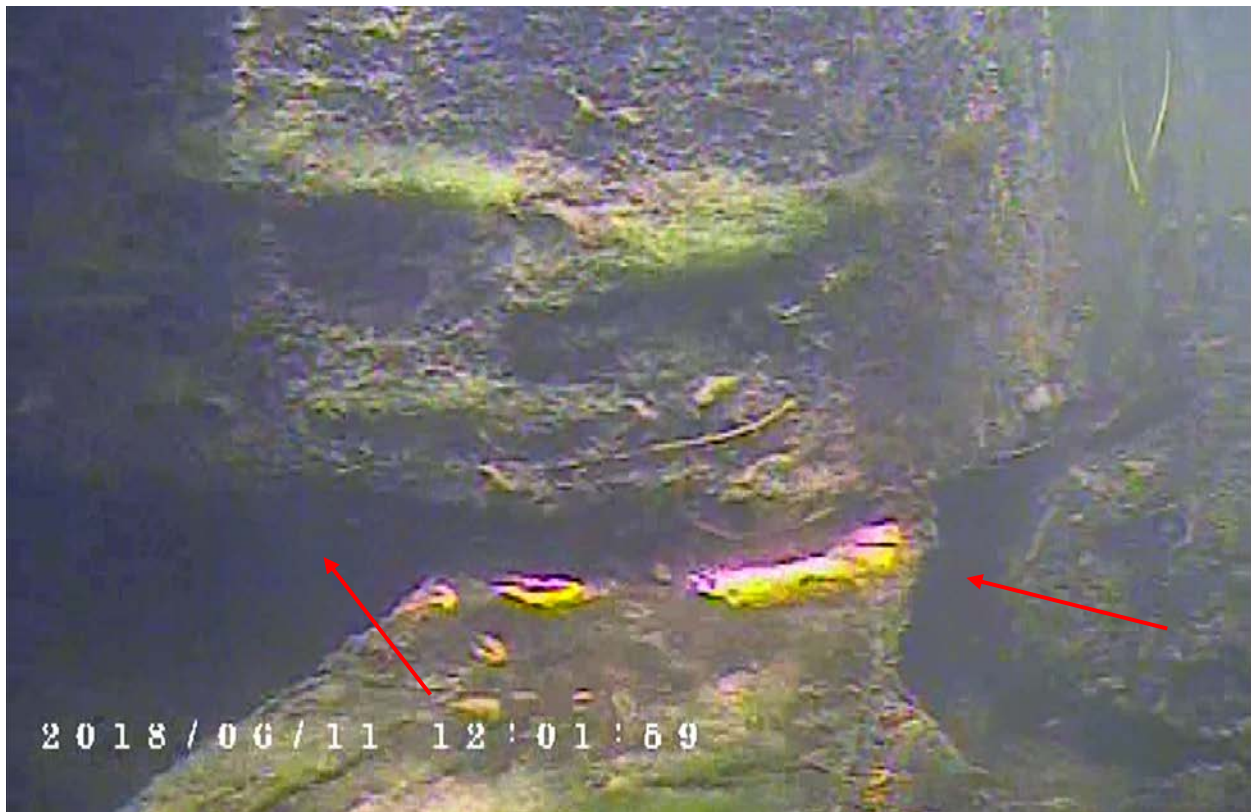
Photo 70 – Pier 6. South end of the footing is undermined by approximately 450 mm on each face.
