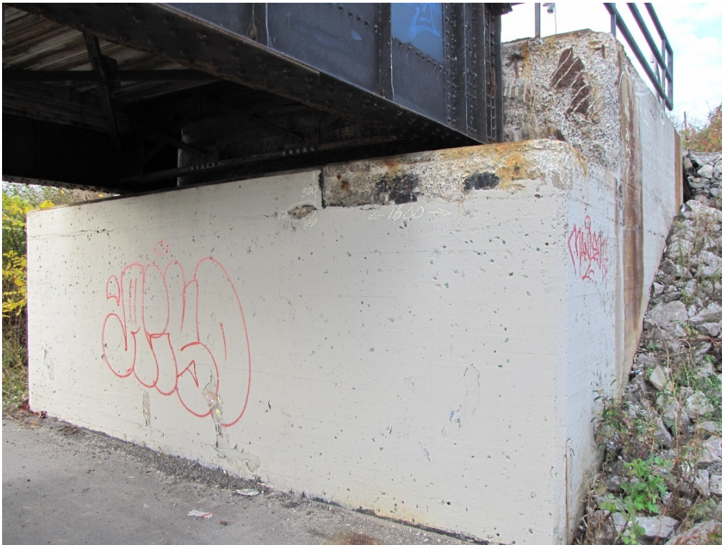
Photo 52 – Localized area of very severe disintegration in the west abutment wall and very severe disintegration and delamination with exposed corroded rebar on the north end of the ballast wall.
