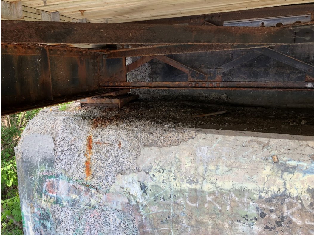
Photo 49 – Very severe disintegration at the top of the east abutment wall and bearing seat at the north end.
