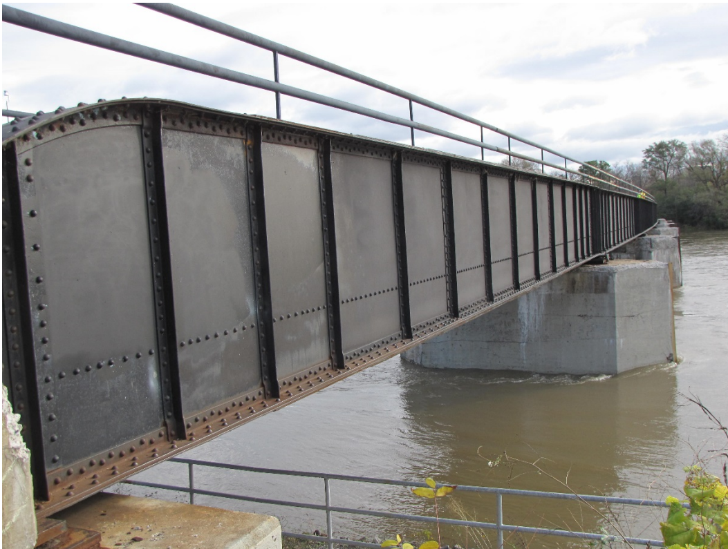
Photo 26 – Localized light corrosion on the exterior girder top of bottom flange and below the top flange.
