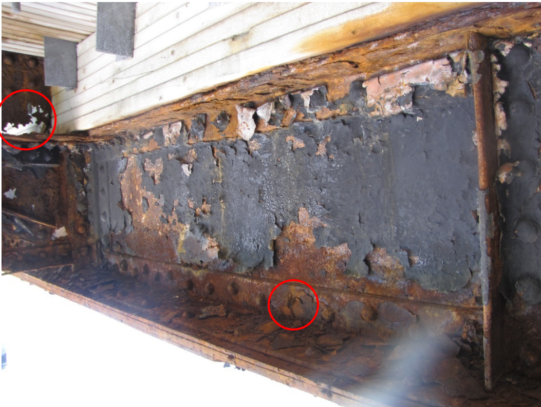
Photo 30 – Typical condition on the interior of the girder below deck. Medium to severe corrosion on the shelf angle below the ledger and bottom flange. Very severe corrosion and perforations in the vertical gusset plate. Corrosion with up to 100% section loss on rivet heads. Typical coating failure with widespread peeling paint.
