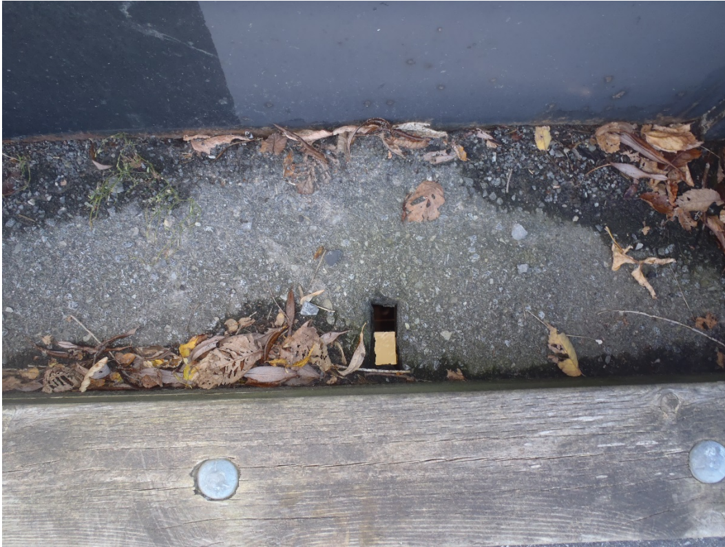
Photo 21 – Rectangular deck drainage openings located every 2 m on each side of deck. Note the medium to severe ravelling and wet staining of the asphalt along the girder web.
