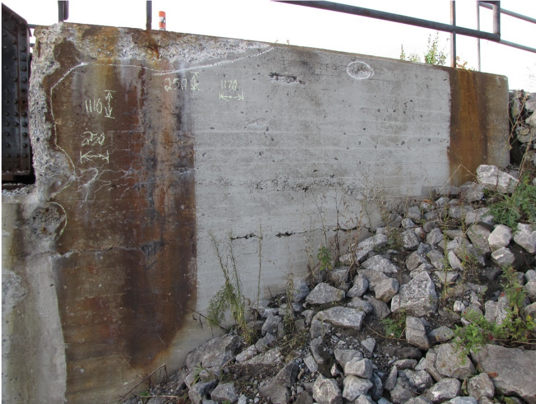
Photo 61 – Medium to very severe disintegration and delamination with exposed corroded rebar on the northwest wingwall. Localized area of efflorescence stained hairline to narrow map cracking.
