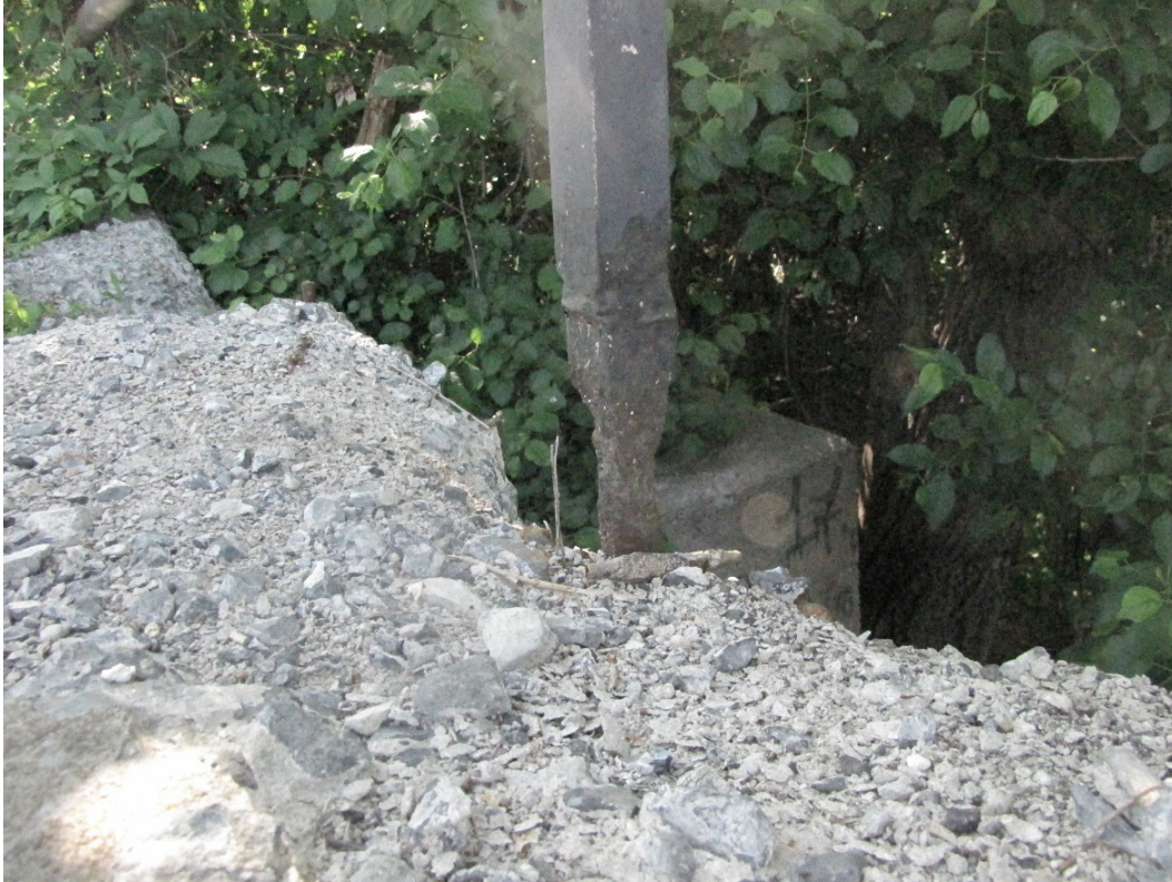
Photo 25 – Very severe corrosion with approximately 75% section loss at the base of a railing post on the southeast wingwall.
