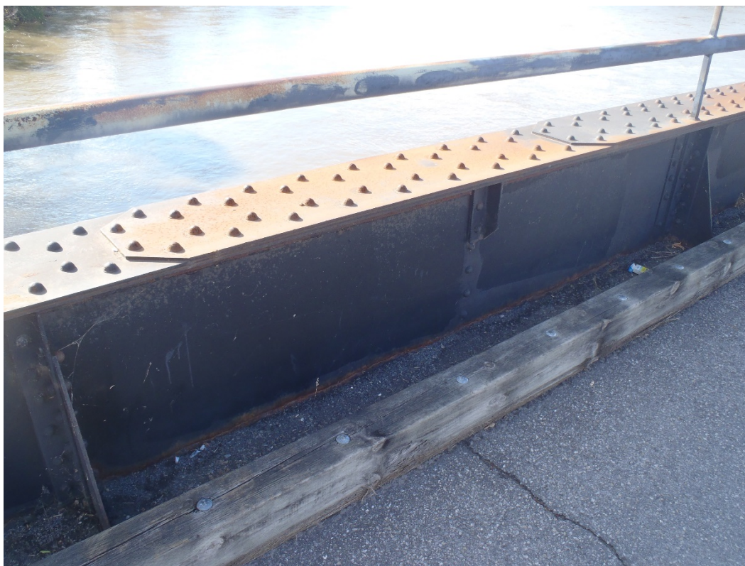
Photo 27 – Localized light corrosion on the top flange of the girder. Typical light to medium corrosion on the girder web and knee braces (i.e. vertical gusset plates) along the top of the asphalt wearing surface.
