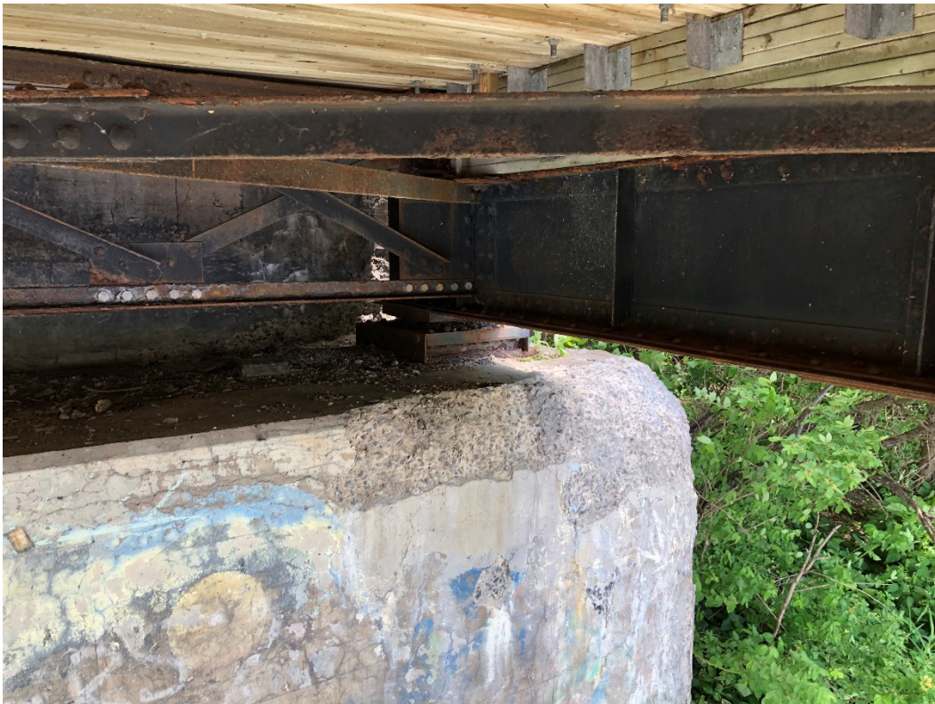
Photo 50 – Very severe disintegration at the top of the east abutment wall and bearing seat at the south end.
