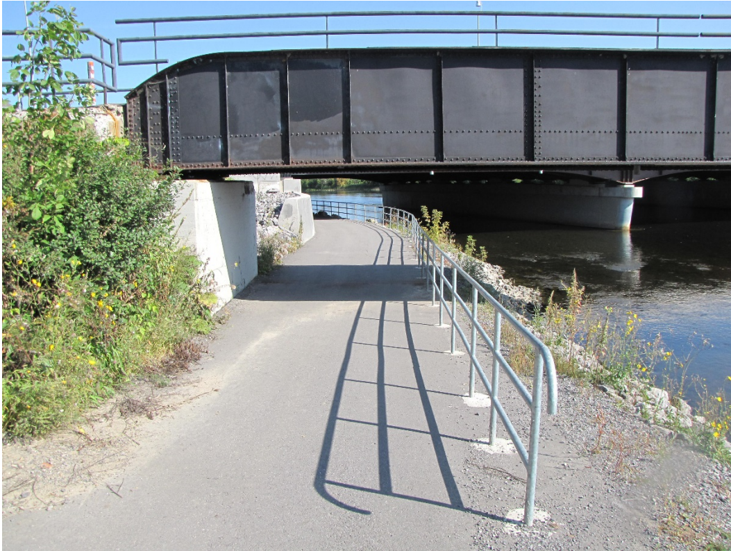
Photo 5 –South elevation. Rideau River Western Pathway passing in front of west abutment below Span 8; vertical clearance of 2.5 m. Note Highway 417 (Queensway) Hurdman Bridge pier in background.
