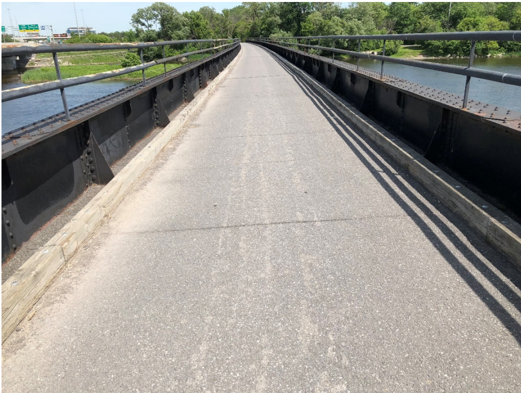
Photo 6 – Typical condition of asphalt wearing surface on the deck top, looking east. Note the light to severe isolated unsealed transverse cracks and light raveling throughout, with medium raveling on exterior of timber curbs.
