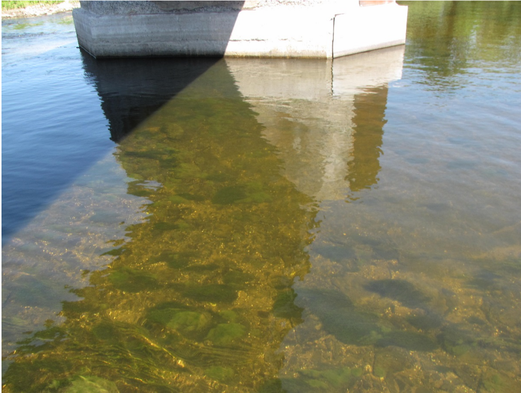
Photo 75 – Typical shallow water depth across the waterway between piers. Riverbed consisting of bedrock or with a shallow layer of silt and sand on bedrock.
