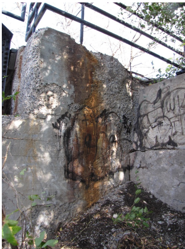
Photo 58 – Extensive areas of medium to very severe disintegration with exposed corroded rebar, delaminations, and hairline to narrow wet and efflorescence stained map cracking on the southeast wingwall.
