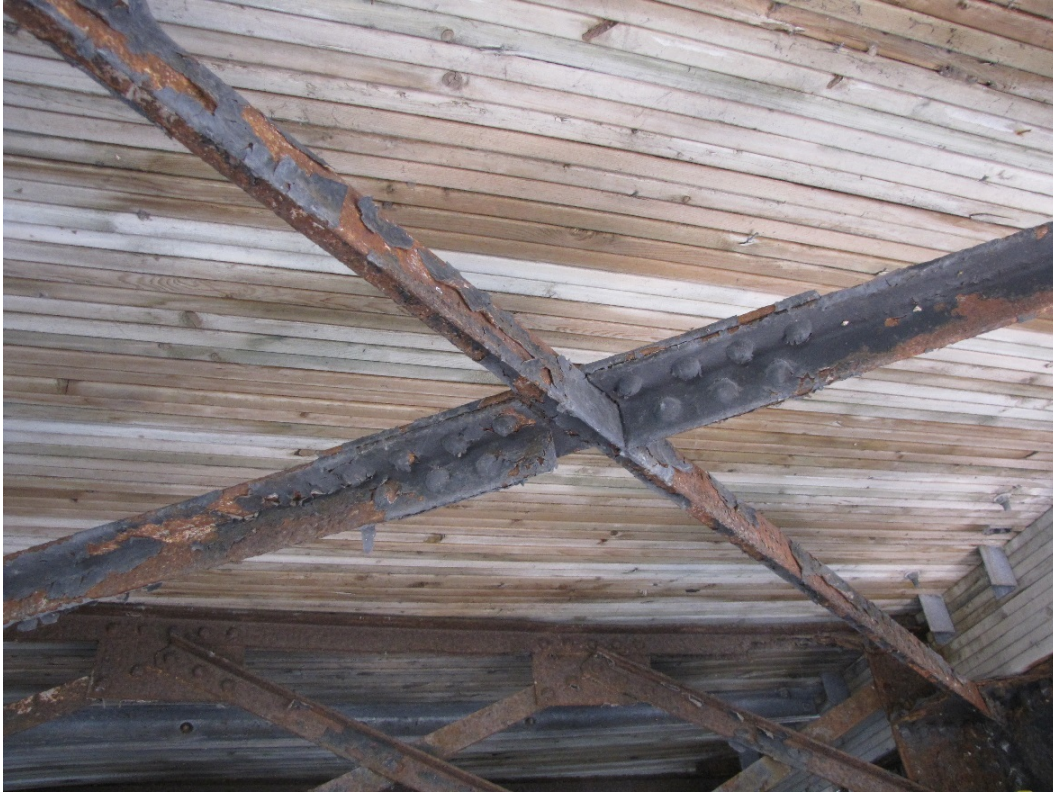
Photo 41 – Typical condition of the lateral bracing. Note the widespread coating failure and light to medium corrosion throughout.
