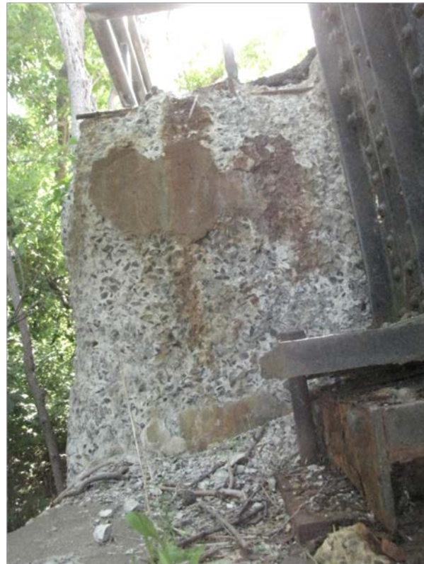
Photo 56 – Severe to very disintegration with exposed corroded rebar at the north end of the east ballast wall.
