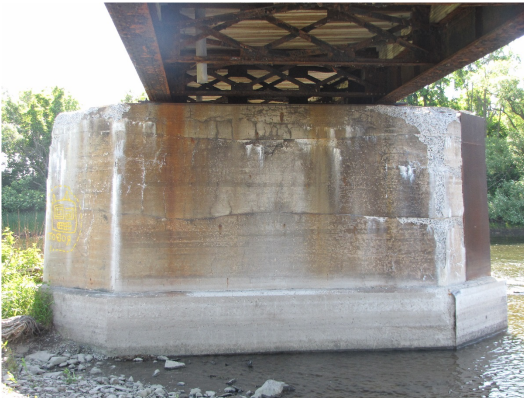
Photo 64 – Pier 3, west elevation. Severe to very severe disintegration with exposed corroded rebar at the bearing seat, isolated cracks and map cracking with wet or efflorescence staining, and wide horizontal construction joints.
