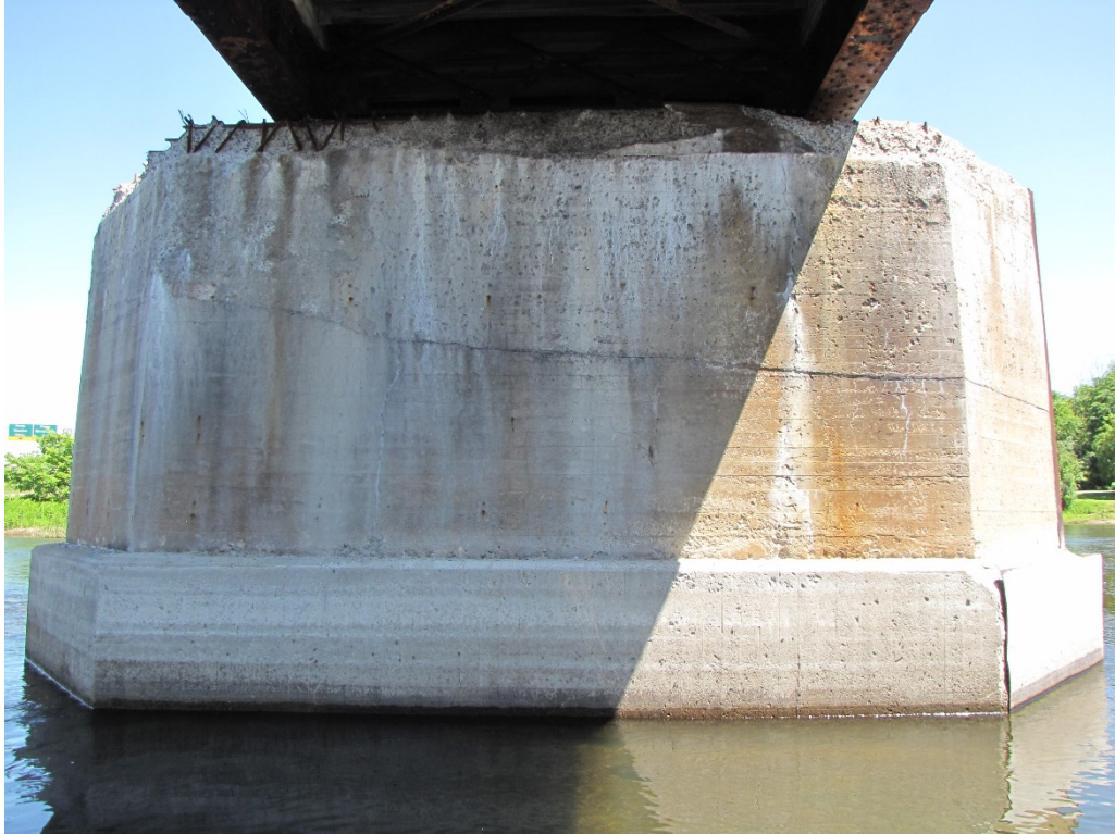
Photo 67 – Pier 5, west elevation. Extensive very severe disintegration with exposed corroded rebar at the bearing seat and wide horizontal construction joint.
