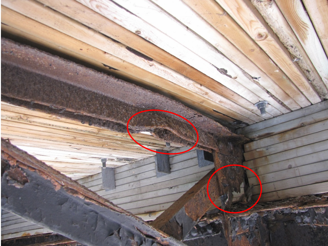
Photo 35 – Cross-frame 2 bays west of Pier 5. Perforation full width of the vertical gusset plate and severe deformation of the top brace member.
