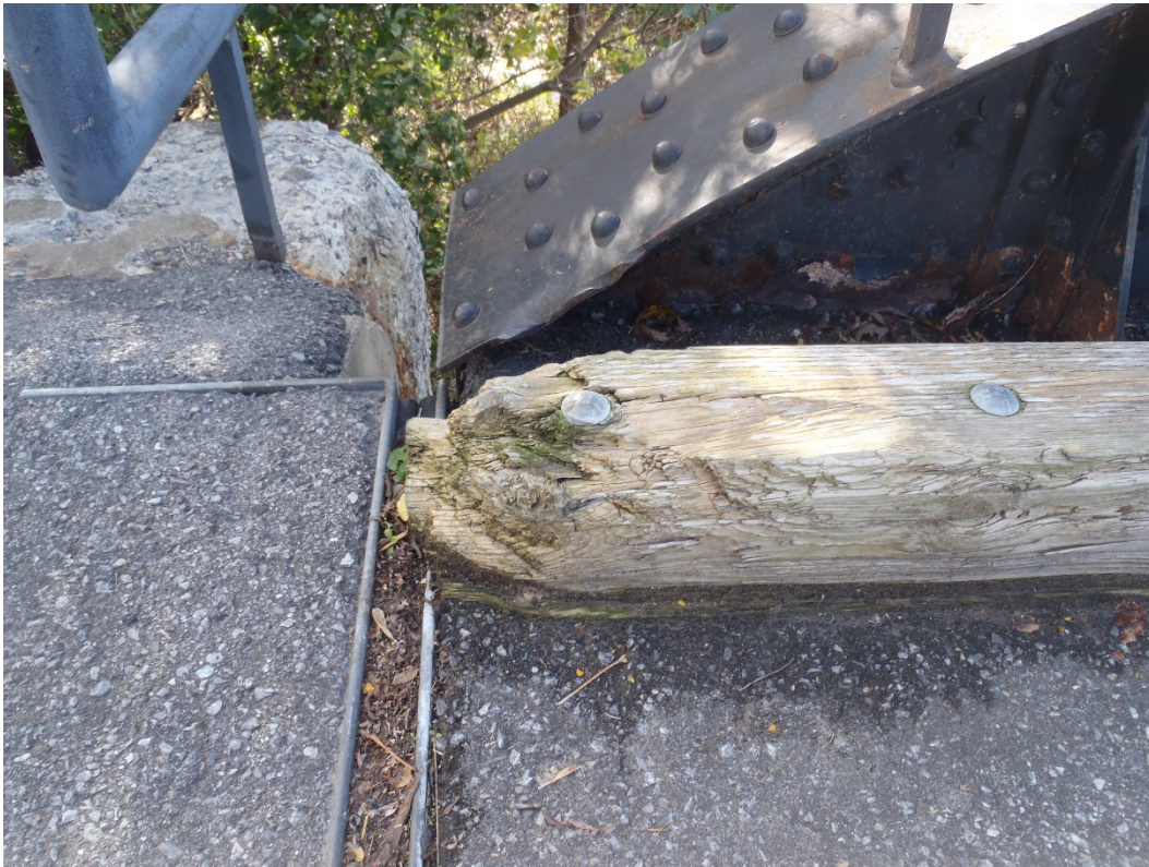
Photo 13 – Impact damage to the east end of the south timber curb.
