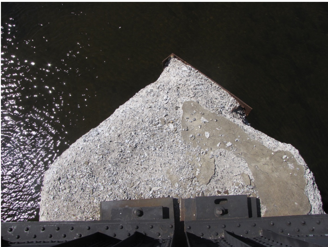
Photo 66 – Pier 4, south end. Severe to very severe disintegration and delamination on the bearing seat up to the bearings.
