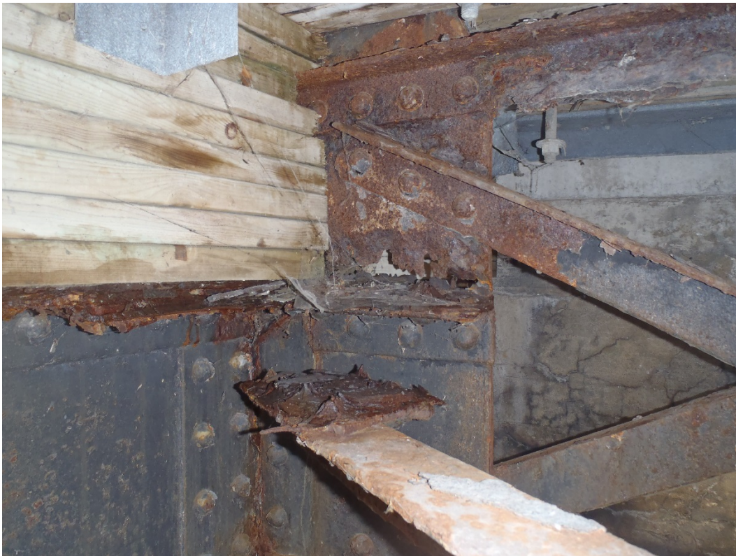
Photo 38 – Very severe corrosion with complete perforation across the vertical gusset plate and detachment of the lateral brace from the horizontal gusset plate at the south end of the west abutment cross-frame.
