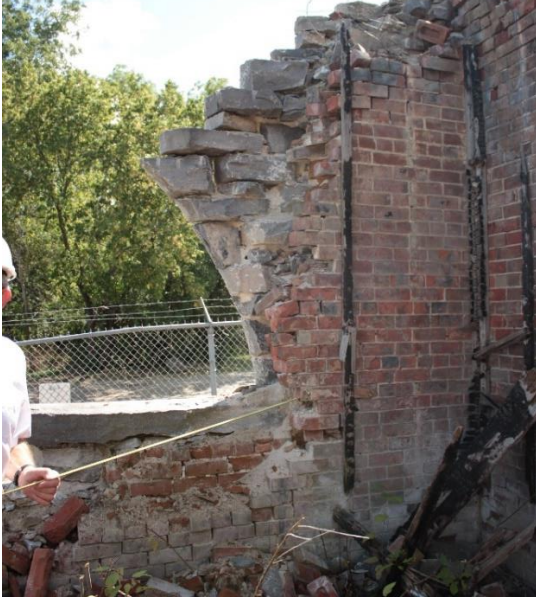
Figure 16: Collapsed east wing arch on south wall [JCAL 2021]
