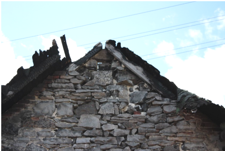
Figure 20: Void joints and displaced stones at gable peak [JCAL 2021]
