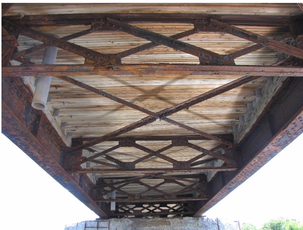
Photo 10 - Underside of Span 7, looking east. Areas of wet staining throughout the soffit of the laminated timber deck. Note water was observed penetrating through the laminated timber deck during the inspection, when raining.
