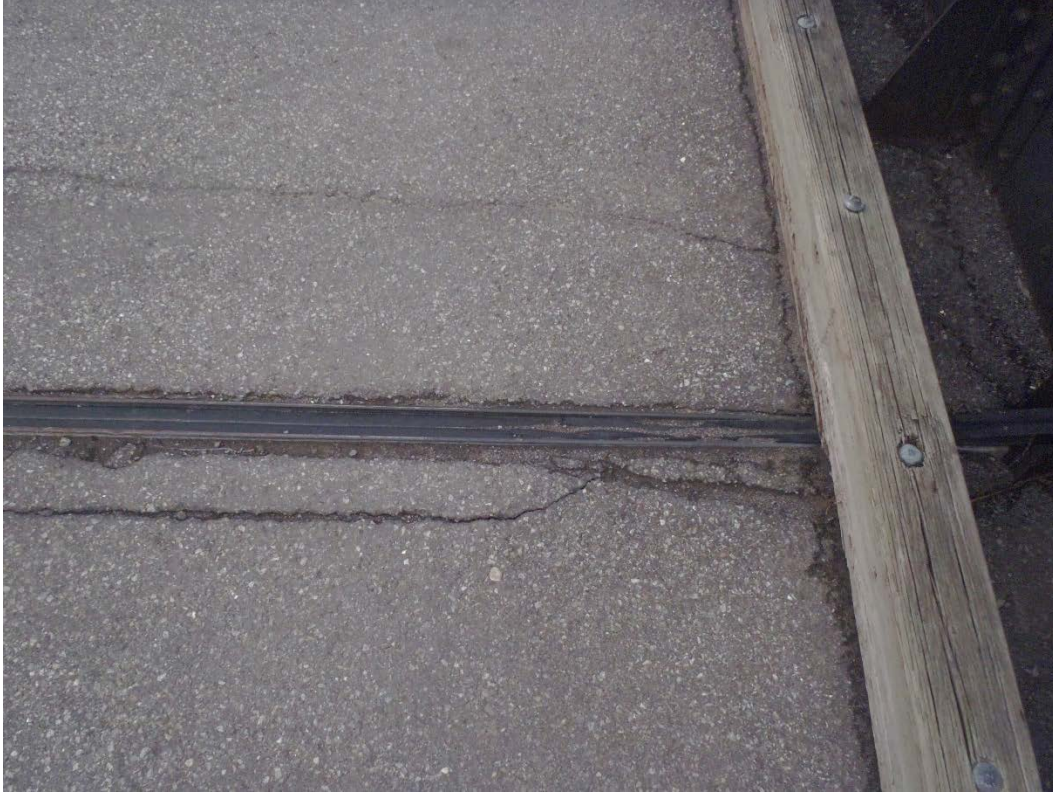
Photo 15 – Broken end of compression seal at Pier 2.
