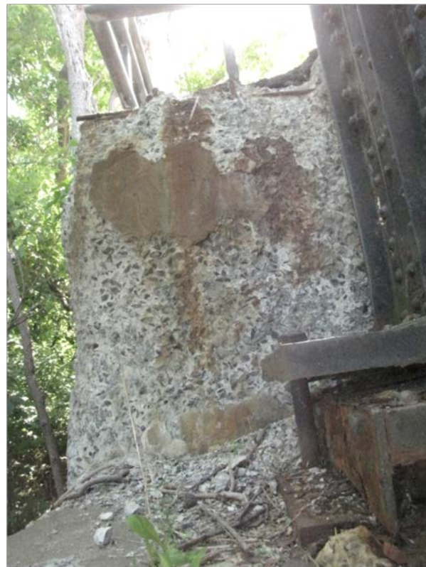
Photo 56 – Severe to very disintegration with exposed corroded rebar at the north end of the east ballast wall.
