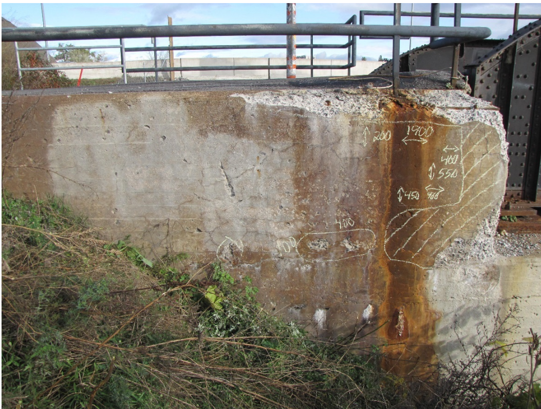
Photo 60 – Light to very severe disintegration and spalls with exposed corroded rebar and hairline to narrow wet and efflorescence stained map cracking on the southwest wingwall. Very severe delamination adjacent to the ballast wall.
