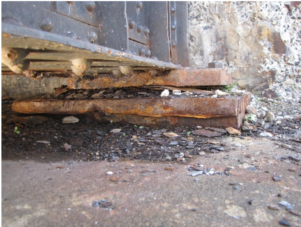
Photo 44 - Medium to severe corrosion on the north fixed bearing of the west abutment.
