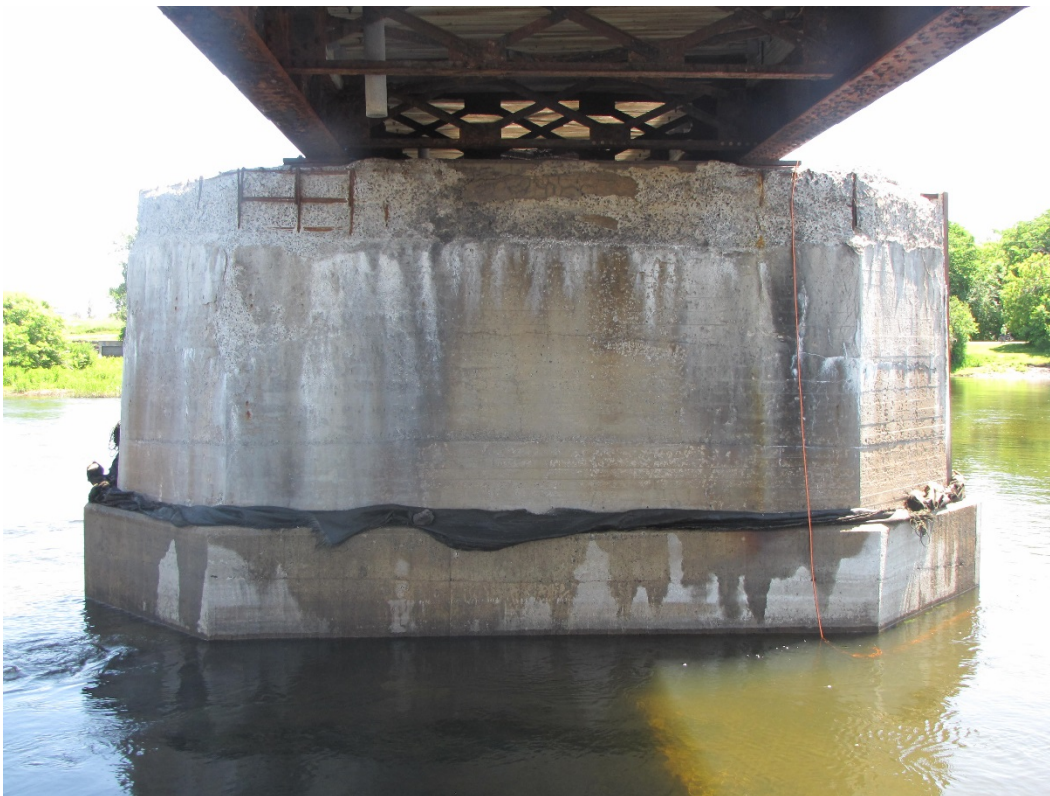
Photo 68 – Pier 6, west elevation. Extensive very severe disintegration with exposed corroded rebar, delaminations and efflorescence staining at the bearing seat, and map cracking with efflorescence.
