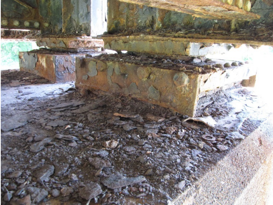
Photo 45 – Pier 2 south bearings. Widespread coating failure, medium to severe corrosion and significant accumulation of debris on top of the bearings and bearing seat.
