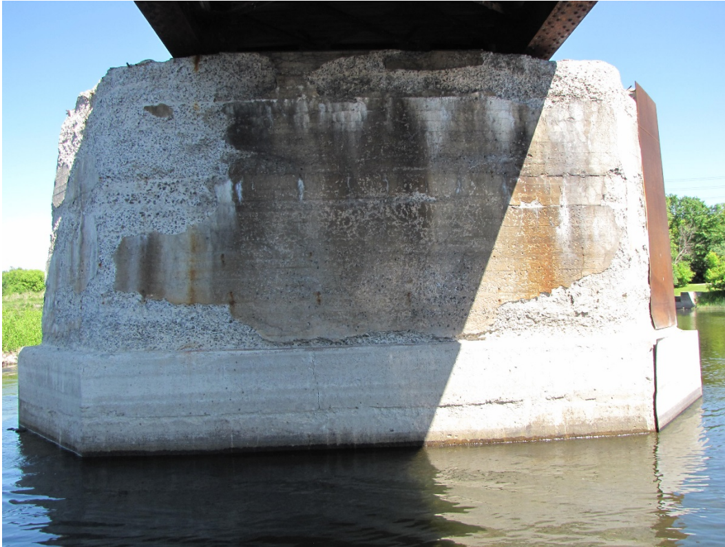
Photo 65 – Pier 4, west elevation. Severe to very severe disintegration with exposed corroded rebar throughout the face of the pier, wet and efflorescence staining, and localized rust staining.
