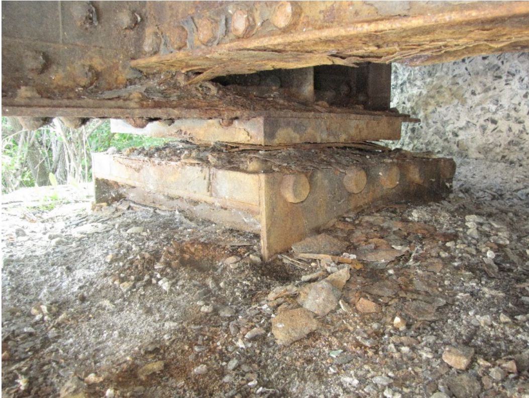
Photo 43 - Light to severe corrosion on the north expansion bearing of the east abutment. Note the significant accumulation of corroded steel and disintegrated concrete on the bearing and bearing seat.
