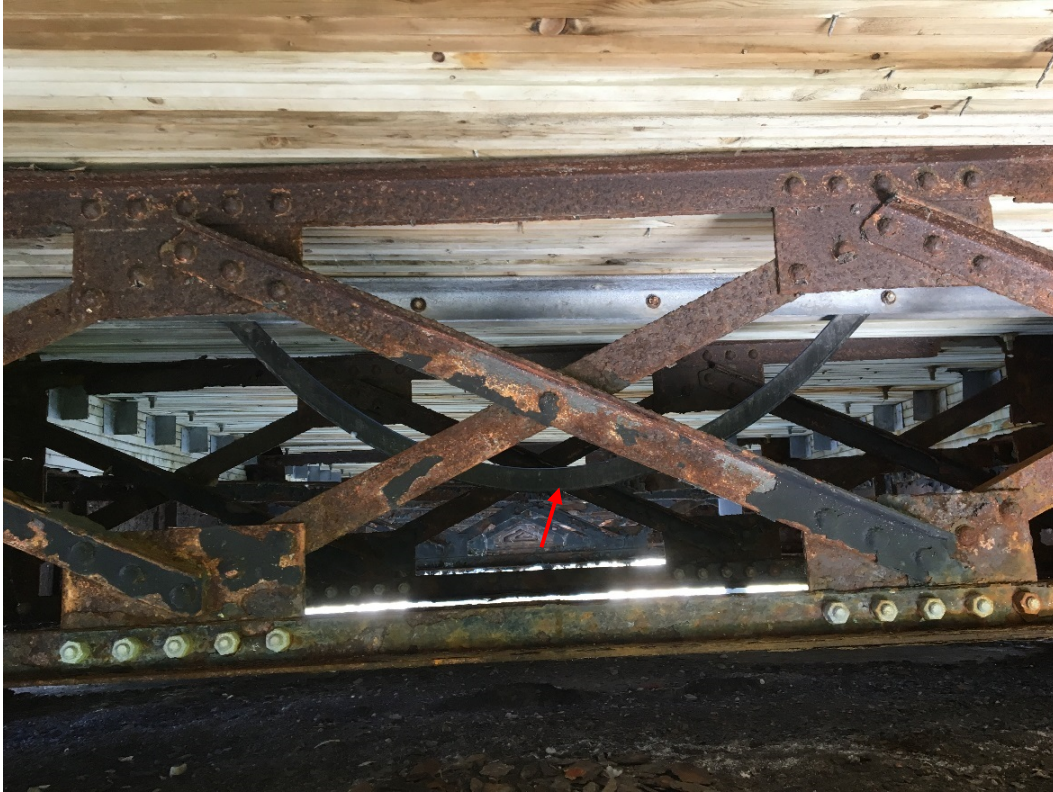
Photo 17 – Significant section of debonded expansion joint compression seal sagging below deck at Pier 4. Light to medium corrosion on expansion joint angle bolts.
