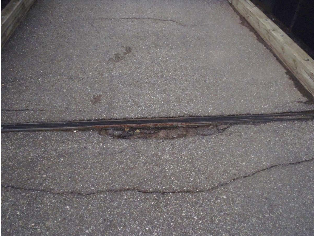
Photo 7 – Light to severe isolated unsealed transverse cracks and asphalt break-up with a pothole at the expansion joint at Pier 6.
