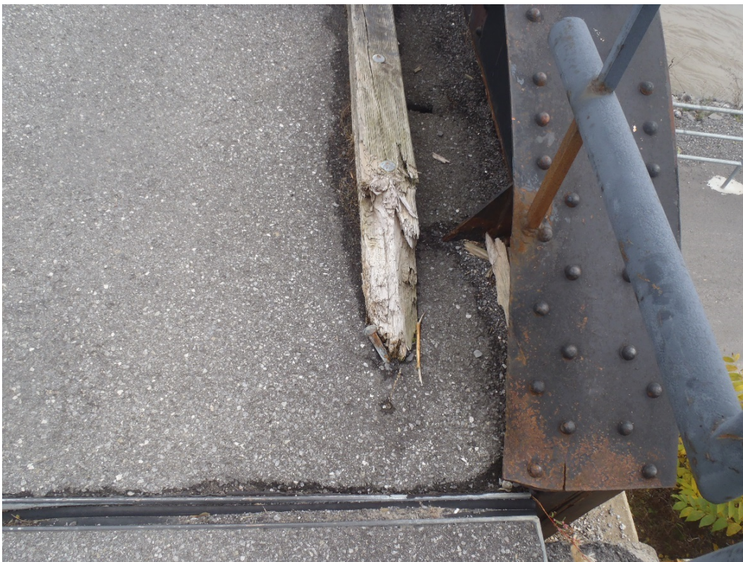
Photo 12 – Very severe impact damage to the west end of the south timber curb. Note the impact damage with cracking and light corrosion in the cover plate of the steel girder.
