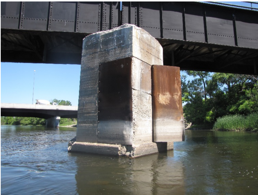
Photo 62 – Pier 1 steel nosing plate on southeast face is detached and folded back. Note lack of a steel nosing angle or plate on the upstream nosing of the footing with a very severe spall.
