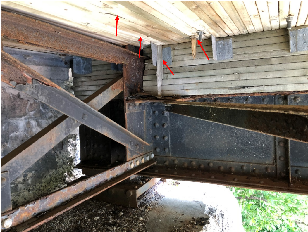
Photo 11 – Light to medium checks in the soffit and ledger and a severe split which has splintered a board in the soffit at the curb bolt. There is a piece of splintered curb timber lodged in the rectangular deck drain at the east abutment.
