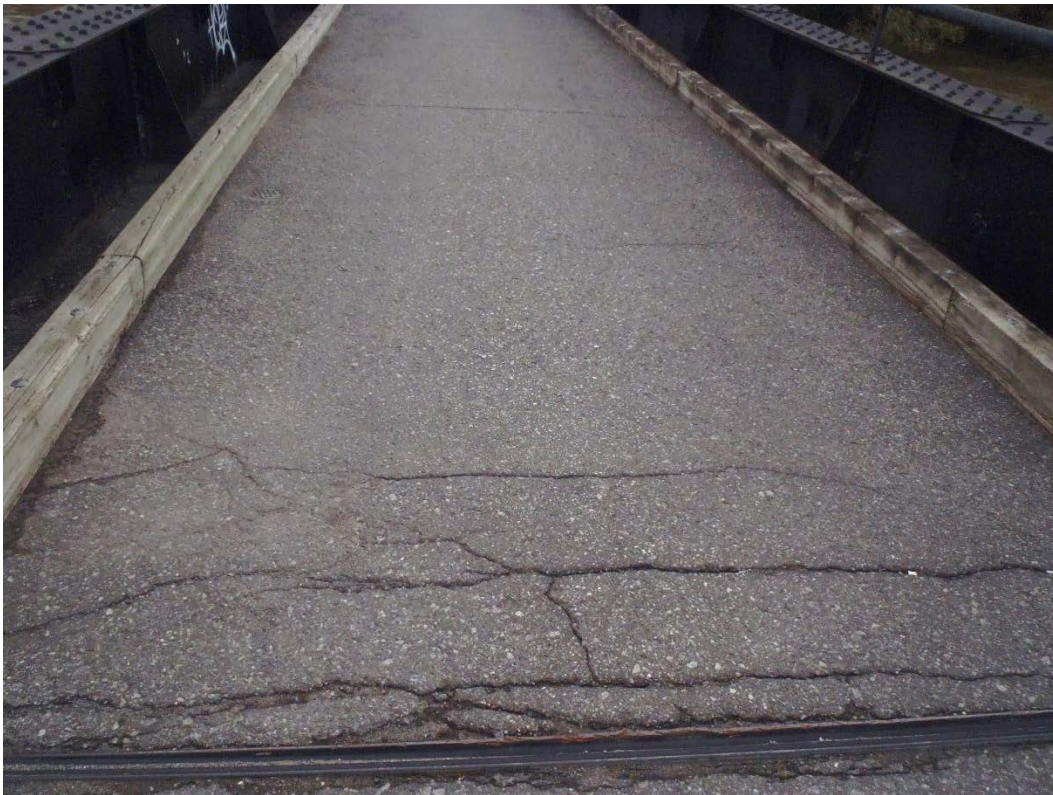
Photo 8 – Light to severe unsealed progressive edge cracks and isolated cracks at the expansion joint at Pier 3.
