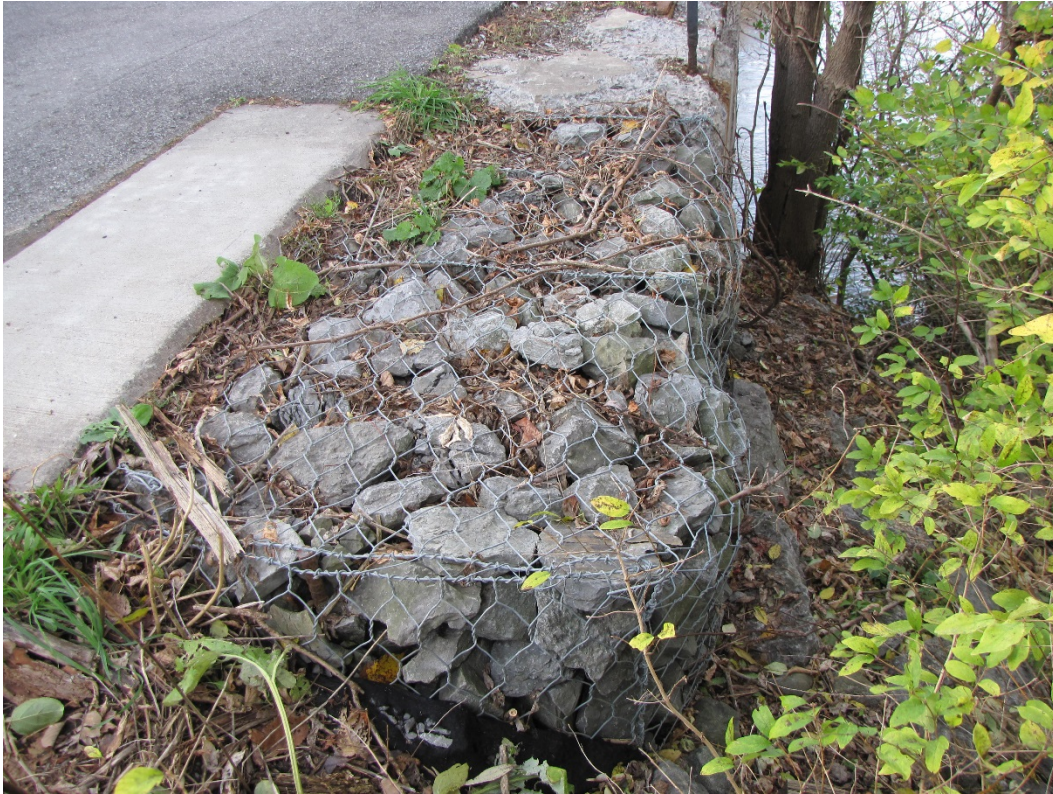
Photo 77 – Gabion basket retaining wall located at the end of the northeast wingwall with slight bulging.
