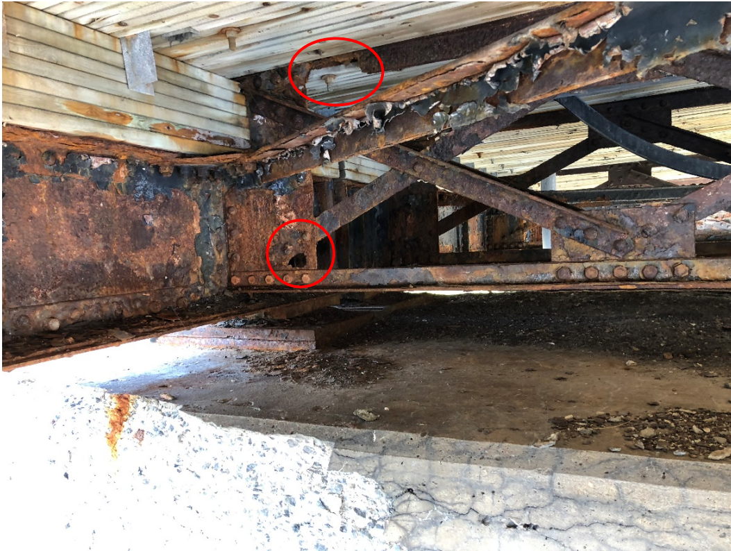
Photo 33 – Cross-frame at Pier 4 complete section loss on the top brace and perforation in the vertical gusset plate.
