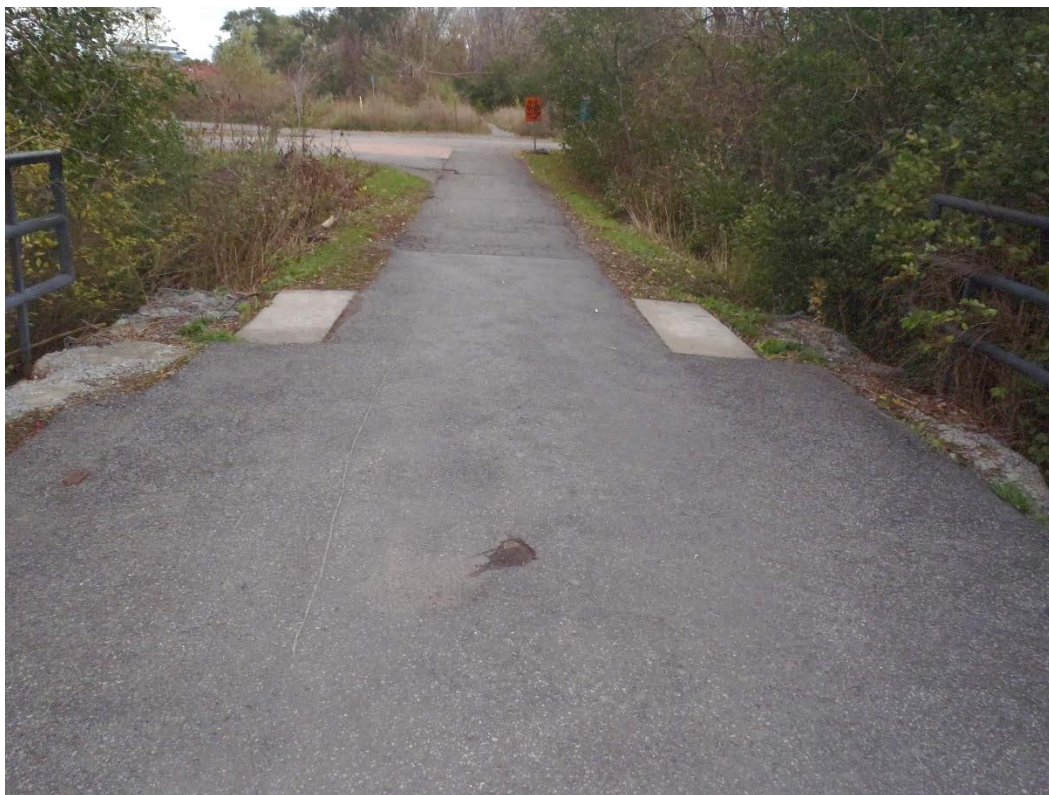
Photo 9 -Light to medium ravelling typical throughout the east approach wearing surface.
