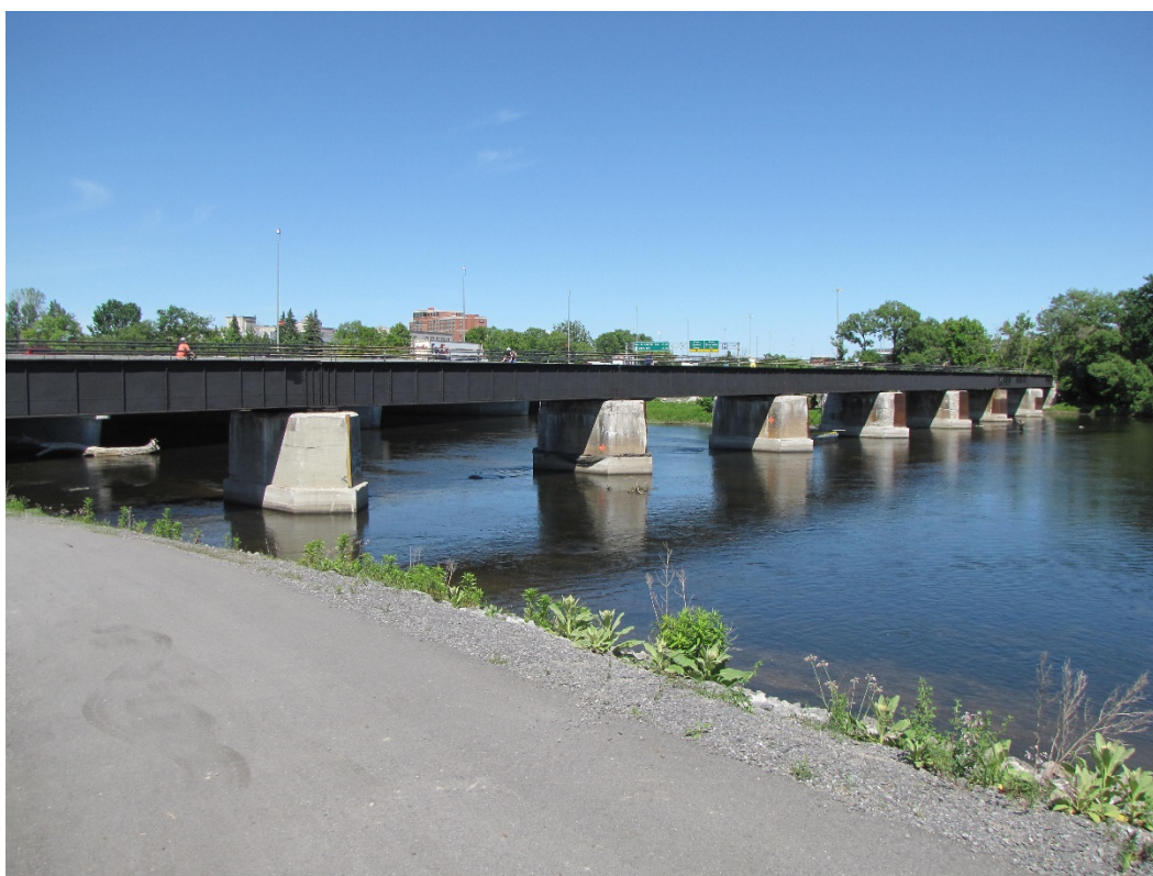
Photo 2 – South elevation. Note Rideau River Western Pathway (foreground), which passes below Span 8.
