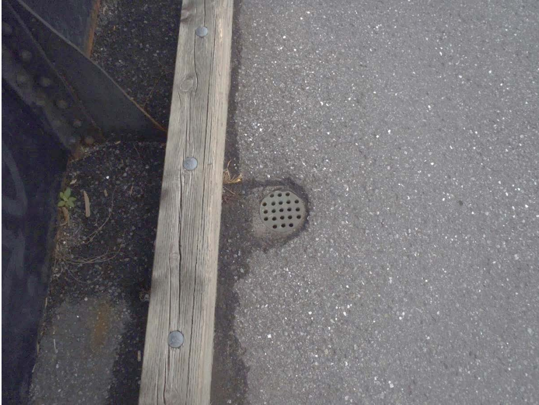
Photo 19 – Medium to severe raveling between the exterior face of the timber curb and girder web. Note typical good condition of deck drain gratings.
