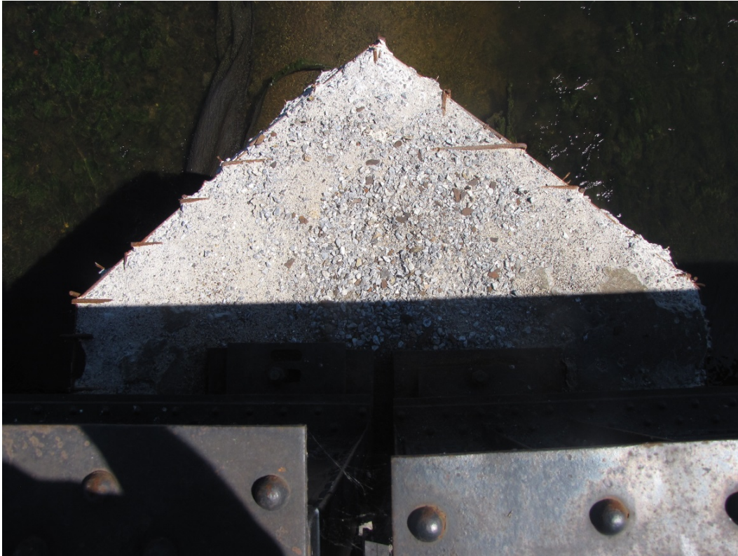
Photo 69 – Pier 6, north end. Very severe disintegration with exposed corroded reinforcing steel on the bearing seat up to the bearings.
