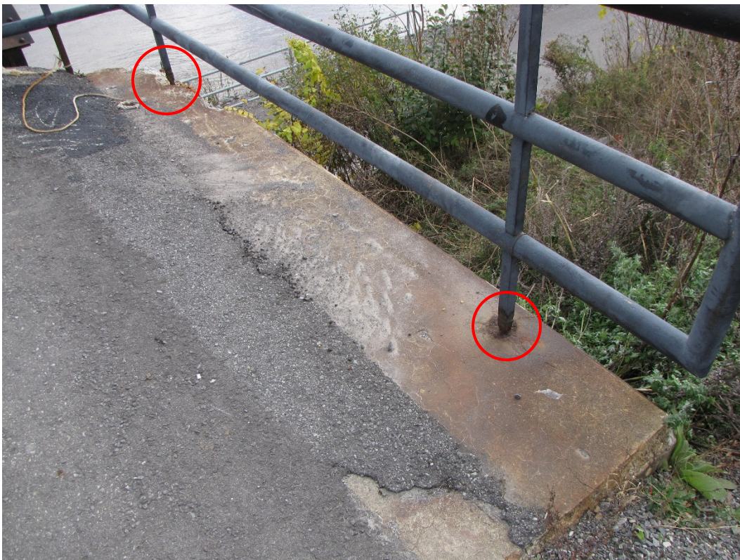
Photo 24 – Severe to very severe corrosion at the base of the approach railing posts embedded into the top of the concrete wingwalls.
