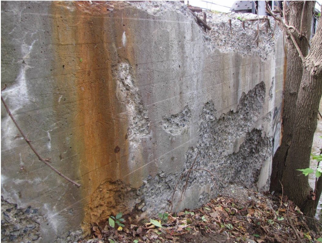
Photo 59 – Extensive areas of medium to very severe disintegration with exposed corroded rebar and hairline to narrow wet and efflorescence stained map cracking on the northeast wingwall.
