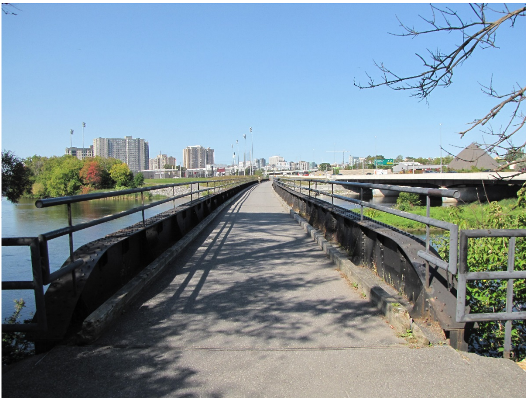
Photo 4 – East approach, looking west across top of deck. Impact damage to ends of timber curbs. Note horizontal curved alignment of the structure towards the north.
