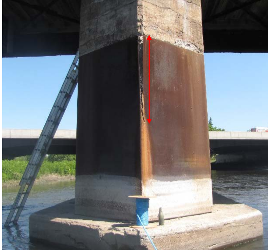
Photo 63 – Pier 2 steel nosing plate is cracked and separated, extending from the top to midway down the center of the plate. Note lack of a steel nosing angle or plate on the upstream nosing of the footing with a very severe spall.
