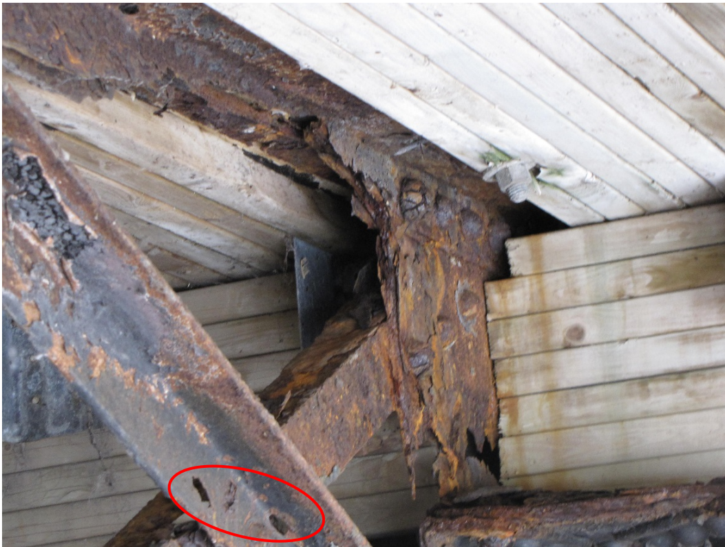
Photo 36 – Severe to very severe corrosion and localized or complete perforations in the diagonal brace, top brace, and vertical gusset plate at the north end of the west abutment cross-frame.
