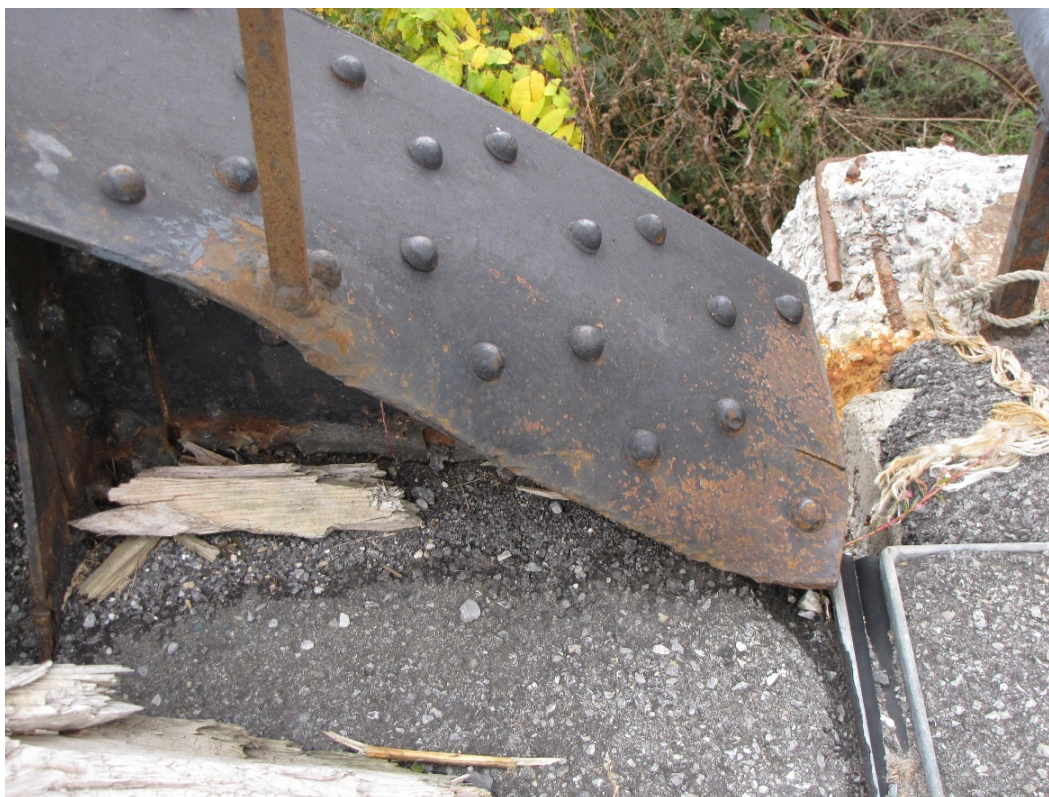
Photo 28 – Impact damage to the top of flange and light corrosion at the west end of the south girder.
