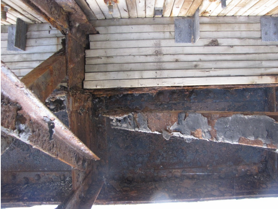
Photo 39 – Complete detachment of the lateral brace from the horizontal gusset plate at the cross-frame in the bay just east of Pier 6.
