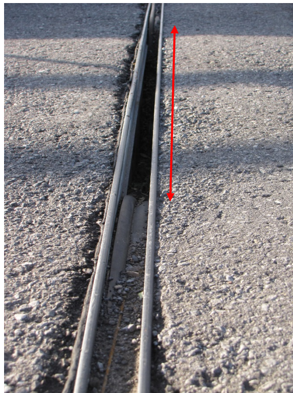
Photo 18 – Failed expansion joint compression seal is sagging below at the west abutment. Also note the asphalt break-up at the expansion joint angles.
