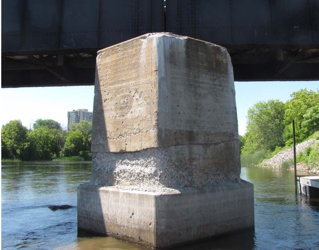
Photo 71 – Pier 7, north elevation. Severe to very severe disintegration below the horizontal construction joint and at the bearing seat.
