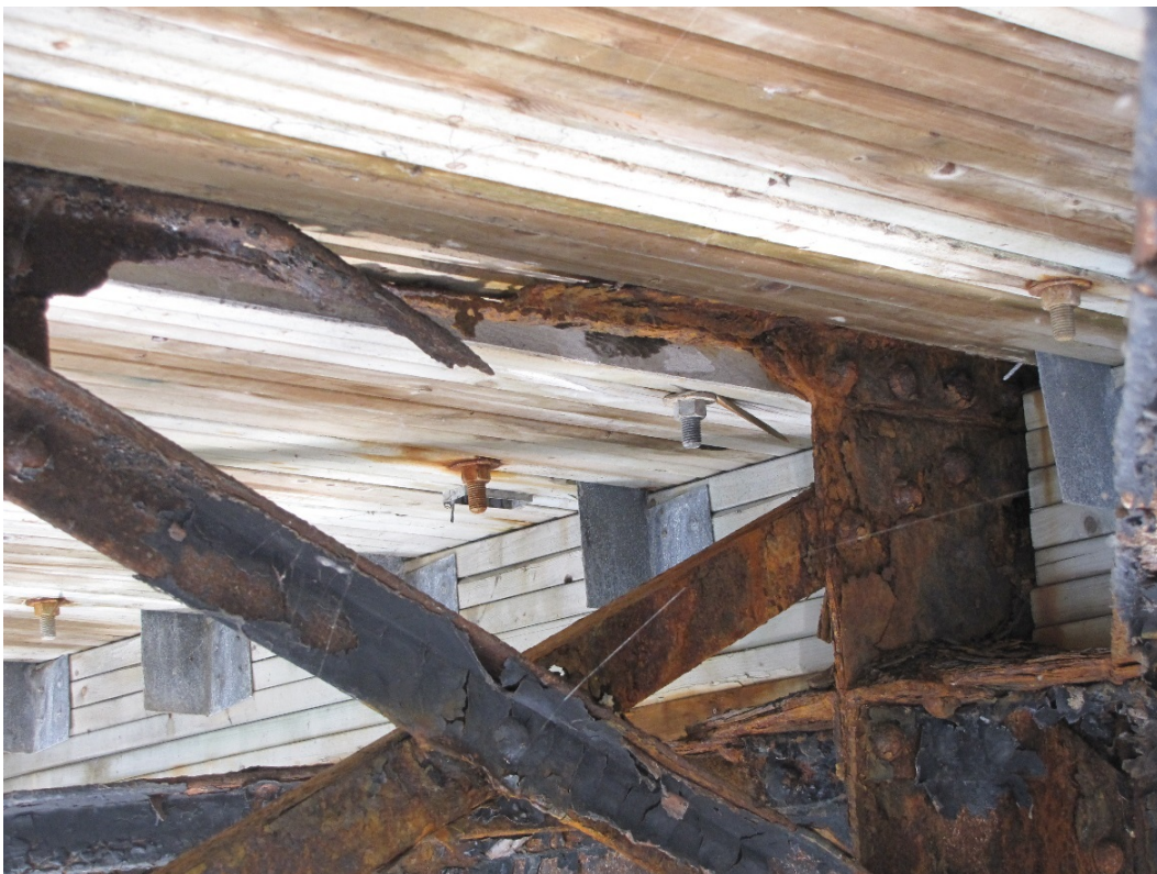
Photo 34 – Cross-frame in the bay just east of Pier 6 has 100% section loss in the top brace.
