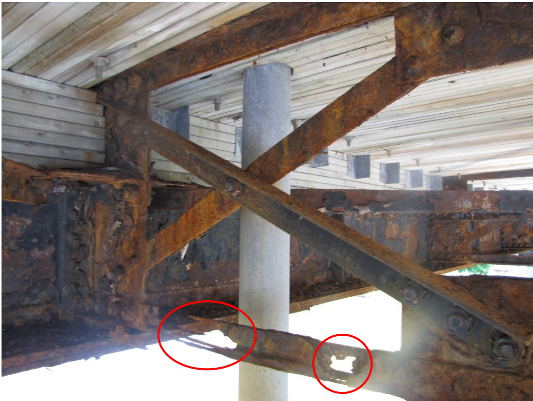
Photo 32 - Cross-frame 3 bays east of Pier 2 has 100% section loss in the bottom brace.
