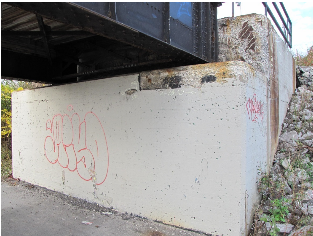
Photo 52 – Localized area of very severe disintegration in the west abutment wall and very severe disintegration and delamination with exposed corroded rebar on the north end of the ballast wall.
