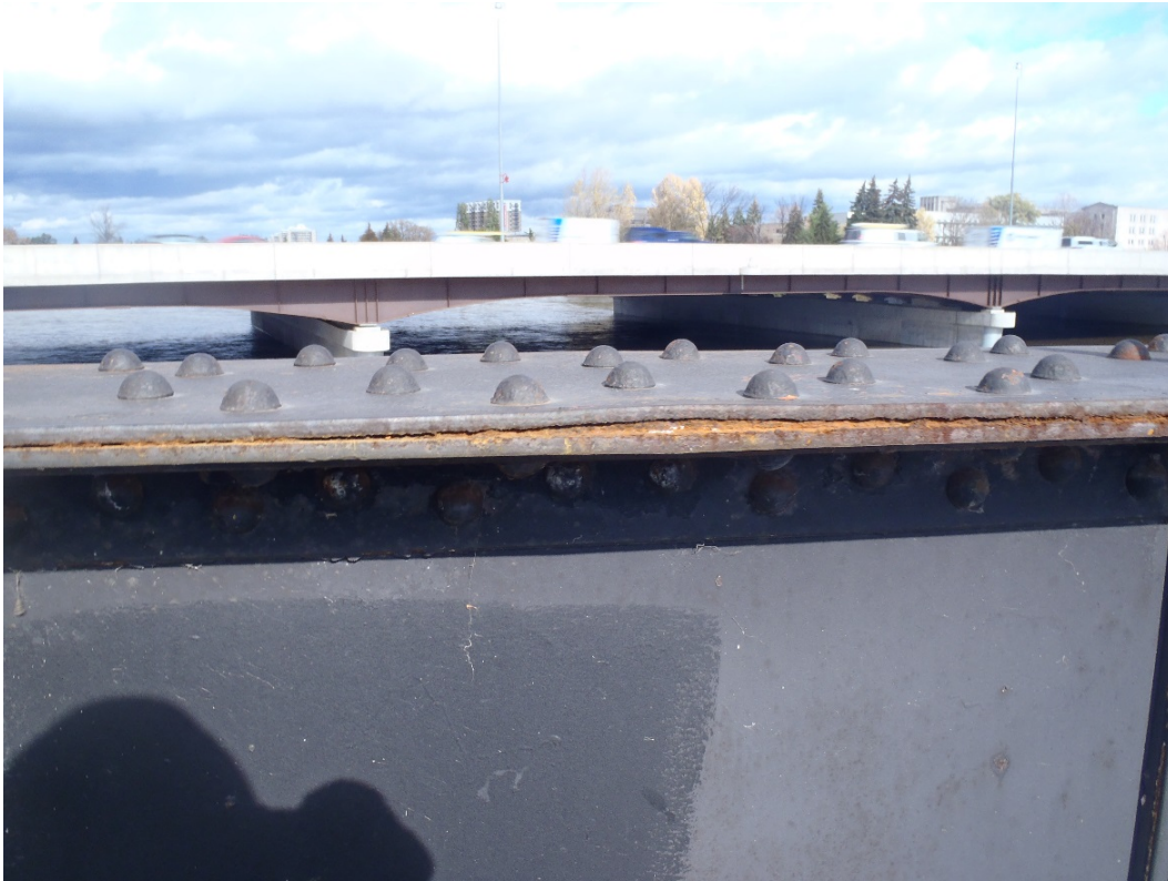
Photo 29 – Light to medium corrosion with rust jacking between cover plates on the top flange of the north girder.
