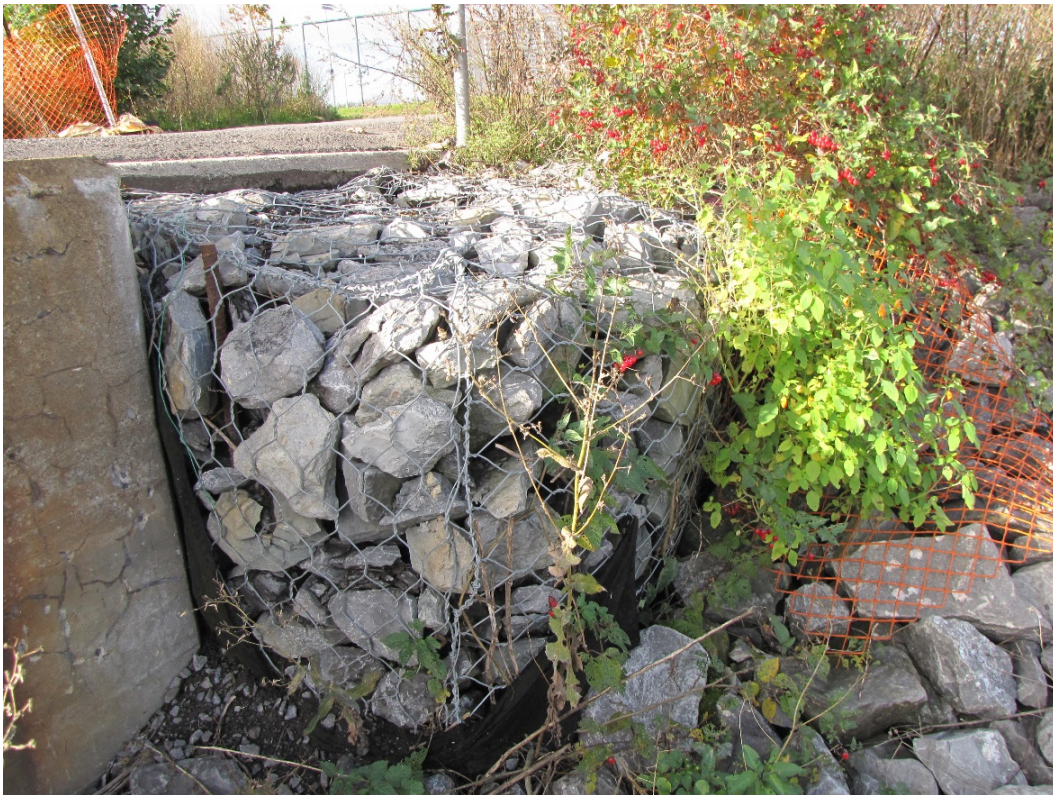
Photo 76 – Gabion basket retaining wall located at the end of the northwest wingwall is in good condition.
