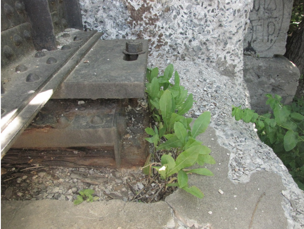
Photo 51 – Very severe disintegration on the ballast wall and adjacent to the south expansion bearing at the east abutment. Note vegetation growth in bearing seat.
