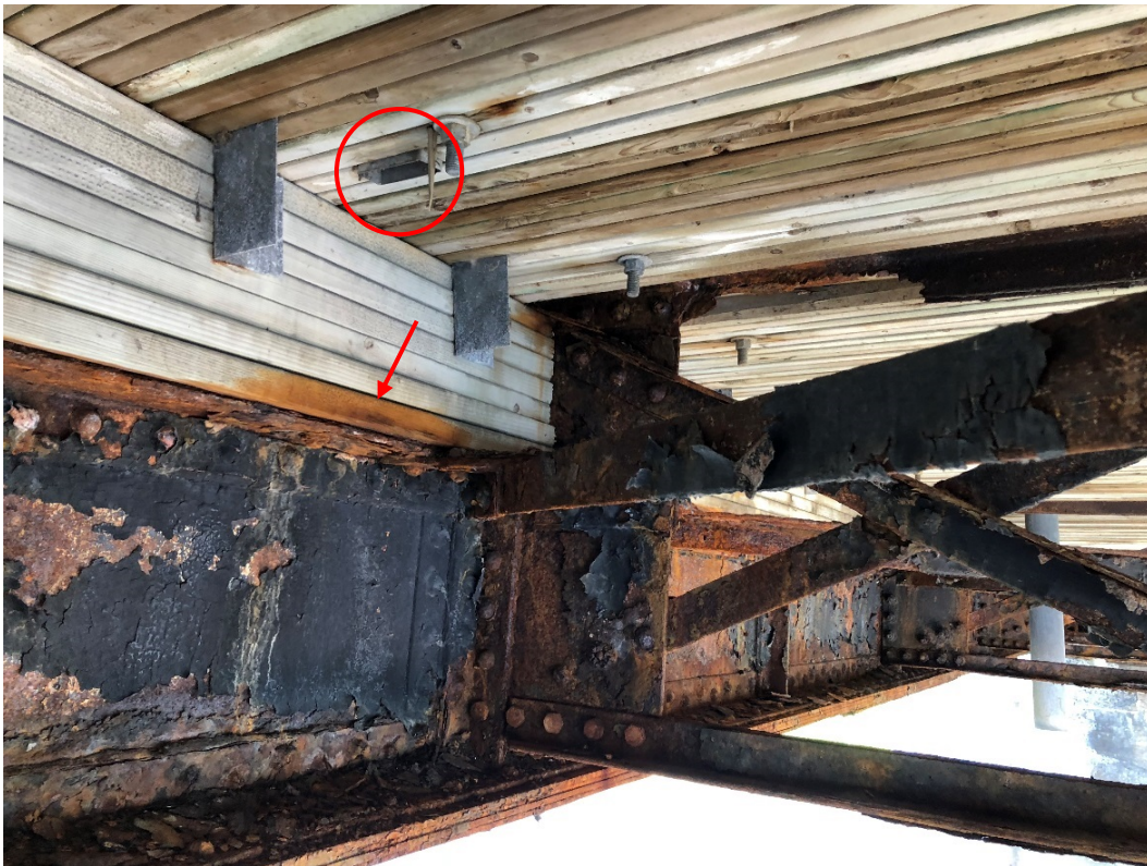
Photo 22 – Rectangular deck drainage opening with no downspout. Note the corrosion staining on the timber ledger and severe corrosion on shelf angle below caused by deck runoff outlet directly onto structure components below.
