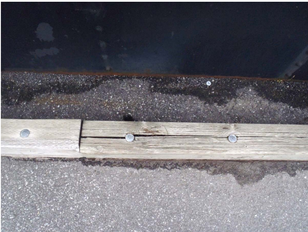
Photo 14 – Light to severe longitudinal splits in the curb from the bolts. Typical localized light weathering is also visible in the top and interior face of curb.
