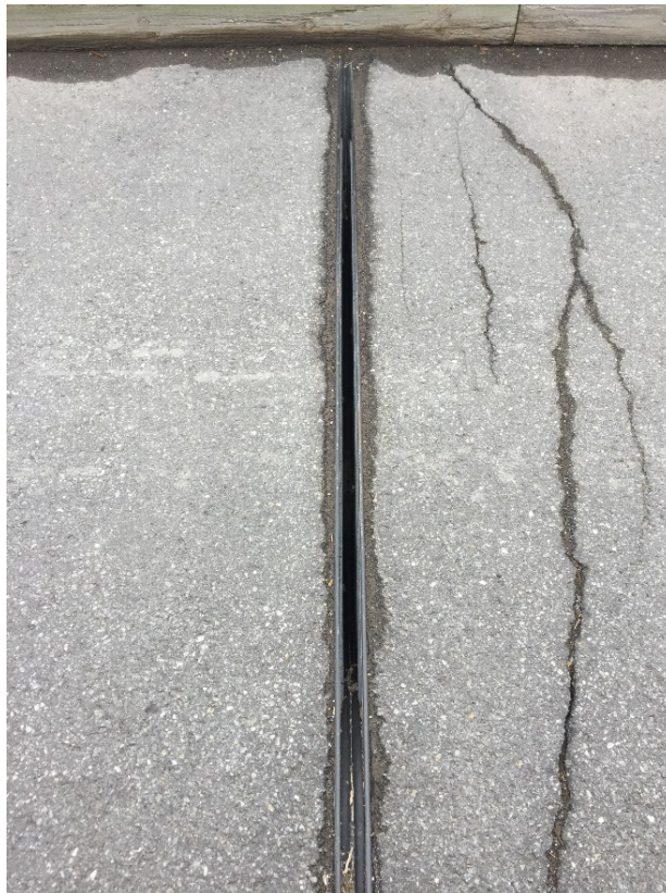
Photo 16 – Failed section expansion joint compression seal sagging below deck at Pier 4.
