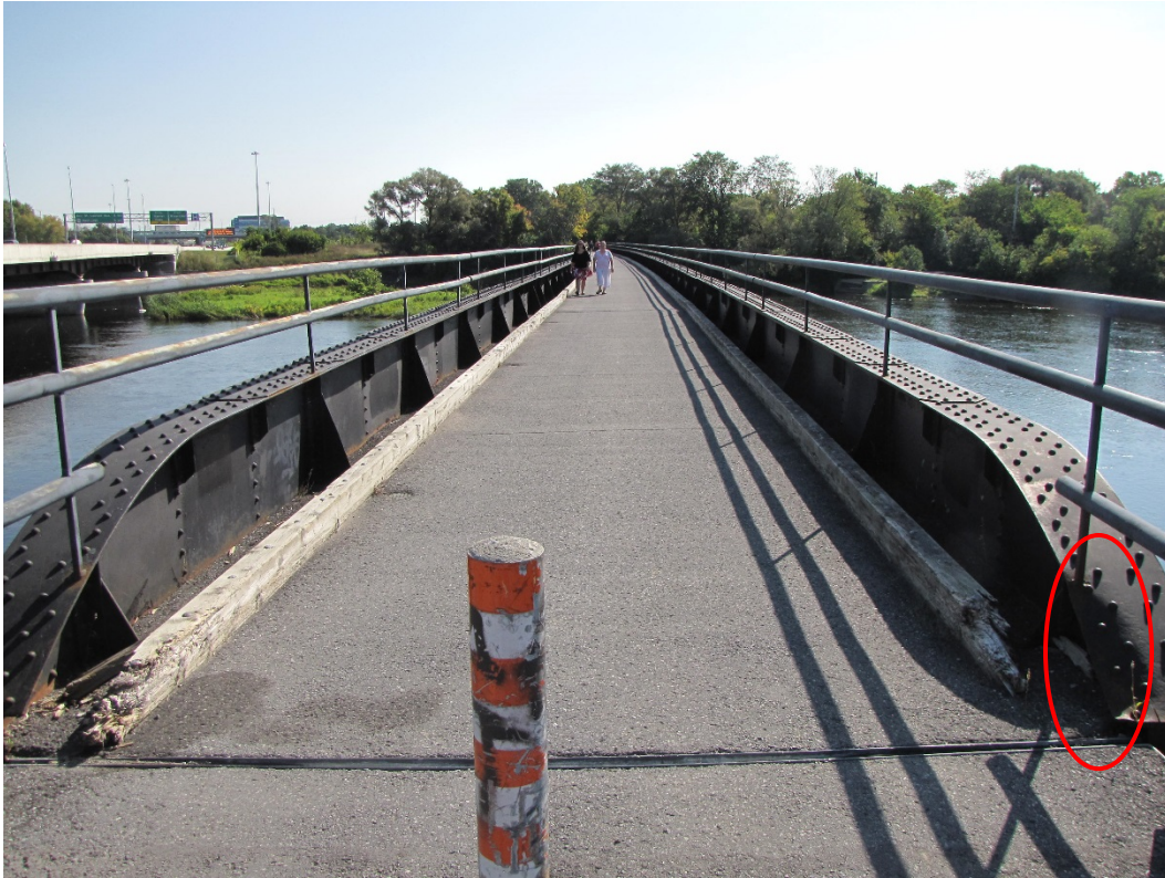
Photo 3 – West approach, looking east across top of deck. Impact damage to ends of timber curbs and top flange cover plate of south girder. Note transverse downslope of deck towards north and deck drains along interior of timber curb.
