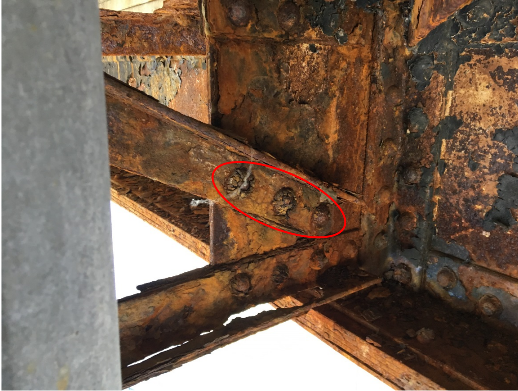
Photo 37 – Severe to very severe corrosion on the rivet heads a diagonal brace and very severe corrosion with perforation in the bottom brace.
