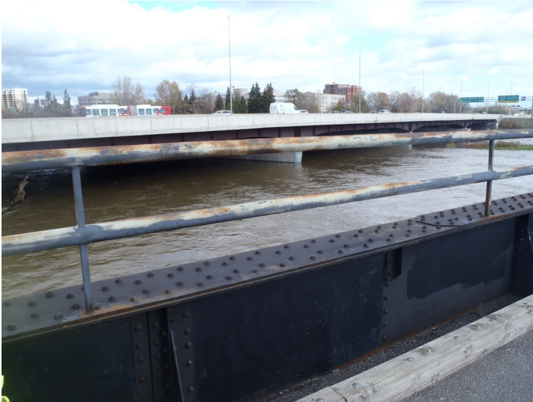
Photo 23 – Localized light corrosion throughout both steel rails and steel pickets on the steel pipe railings due to deterioration of the coating system.
