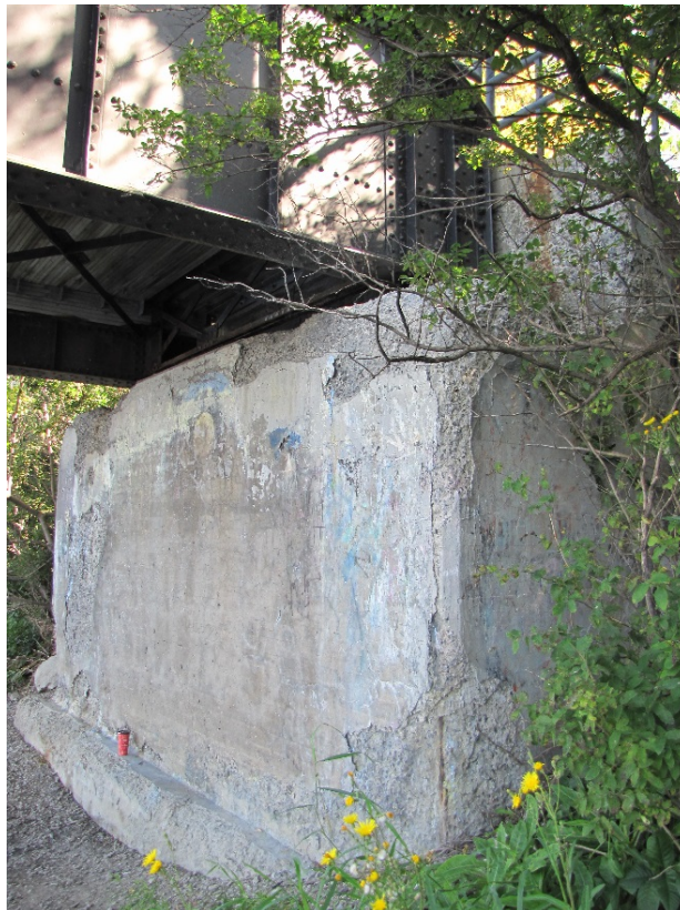
Photo 48 – East abutment. very severe disintegration throughout with spalls, delaminations and exposed corroded rebar on the abutment wall and footing.
