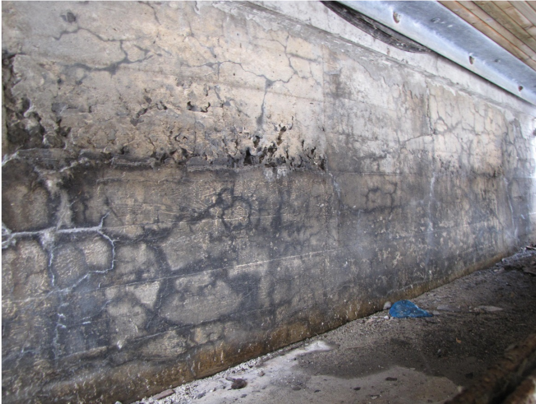
Photo 55 – Wet and efflorescence stained hairline to narrow map cracking throughout, wet staining and medium honeycombing in the west abutment wall.
