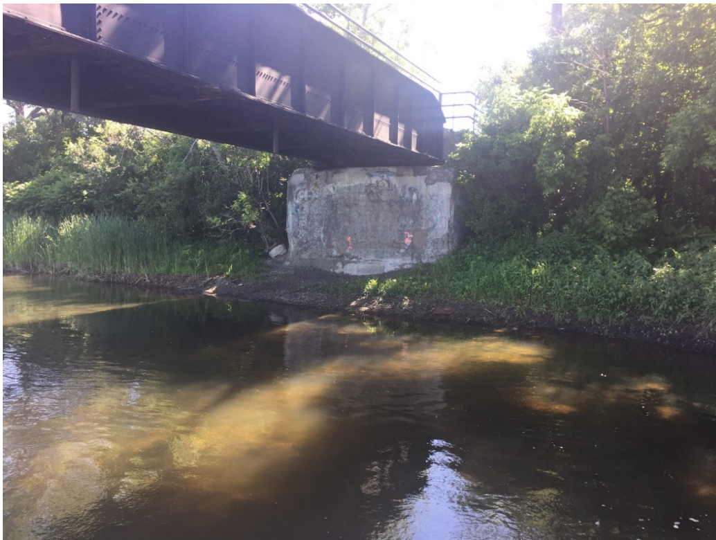
Photo 72 – Embankment in front of the east abutment in fair condition due to erosion of embankment material. Southeast and northeast embankments well vegetated, but steep.
