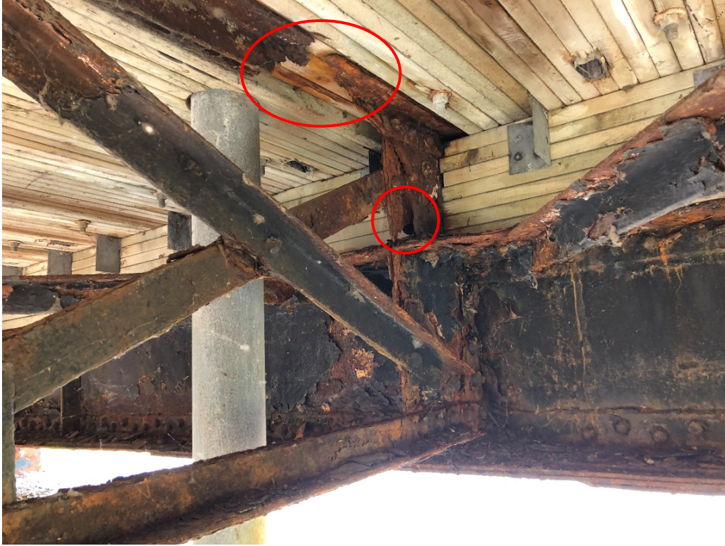
Photo 31 - 100% section loss in the top brace and vertical gusset plate of the cross-frame 2 bays east of Pier 1.
