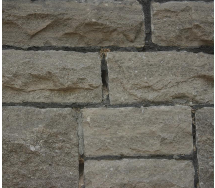
Figure 12: Mortar condition on exterior wythe of north wall [JCAL 2021]
