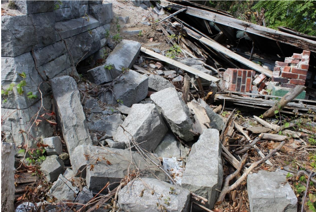
Figure 13: Remaining features of east wall, including brick piers, stone steps, and basement [JCAL 2021]
