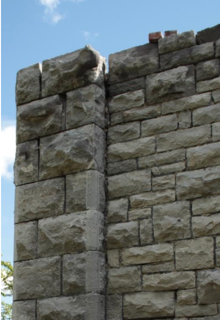
Figure 11: Detached northeast corner [JCAL 2021]
