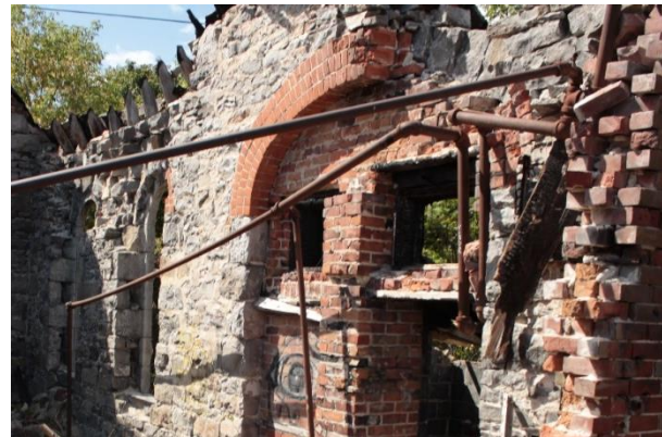
Figure 8: Collapsed inner wythe above archway [JCAL 2021]
