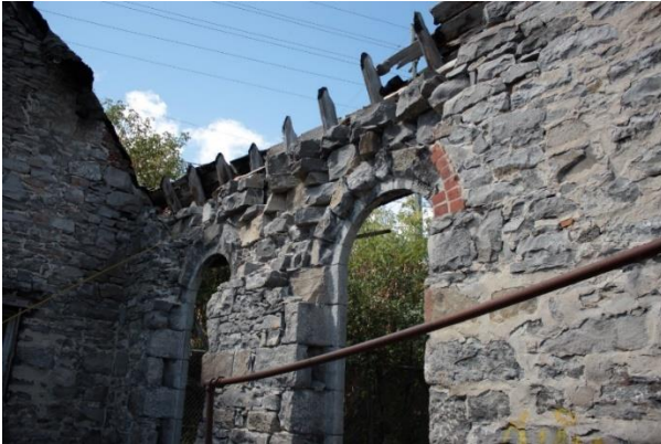
Figure 7: Collapsed inner wythe above arched windows [JCAL 2021]
