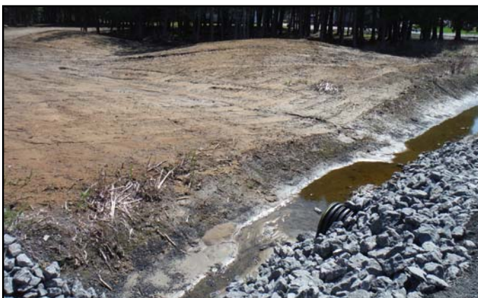
Extensive sediment deposition observed on Joannise Road
