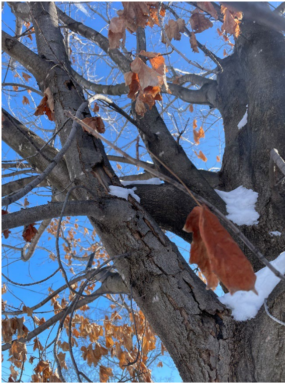
Figure 3: Tree 1 - dead wood/decay in junction of main stem
