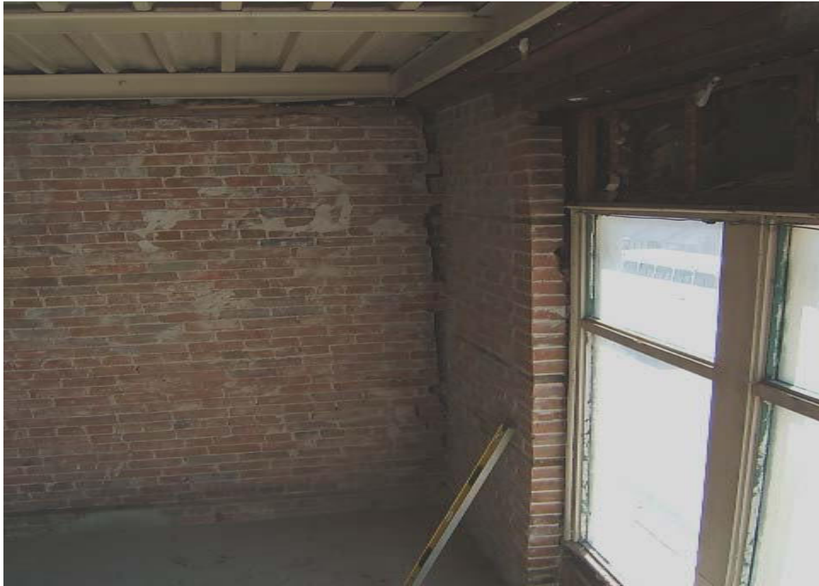
Figure 8: Previously Existing Condition Outlining Movement of West Wall
