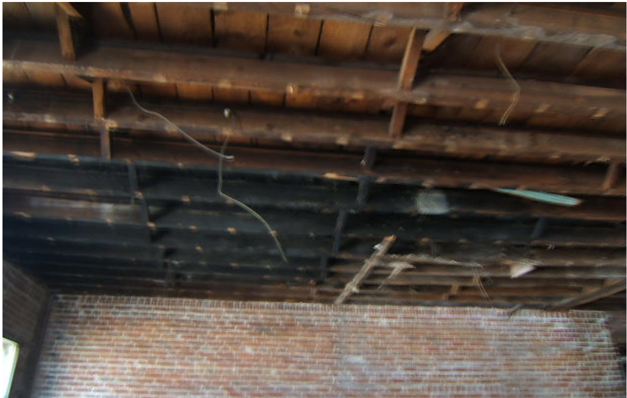
Figure 4: Previously Existing Condition Flooring System and Fire Damage
