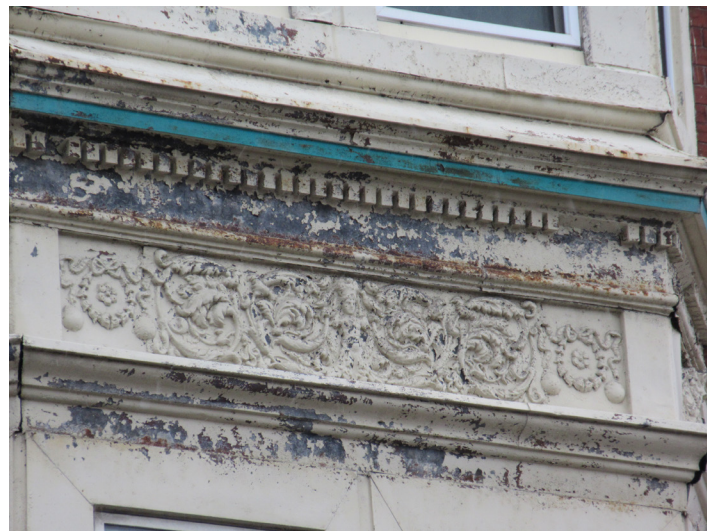
Bay Window Metal Work Relief Details to be Restored
