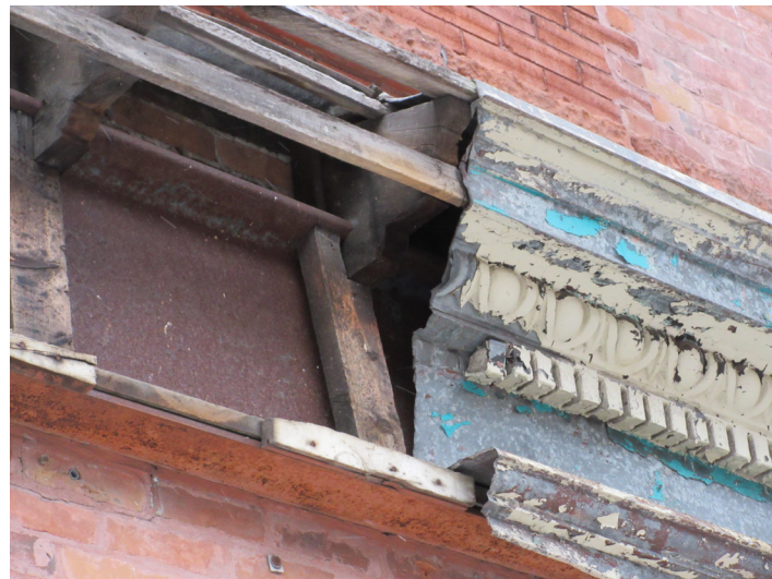
Low Level Cornice to be Replicated
