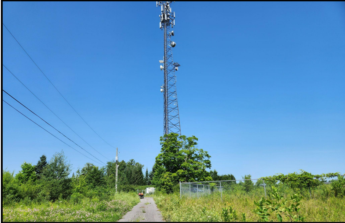
3. Cell tower located in the northeast corner of Part 3, east of the pond in image 1 and west of the Park N' Ride in image 2.
