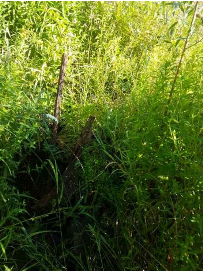
13-Culvert 1+350 - Upstream end ~1000mm CSP poor condition.jpeg
