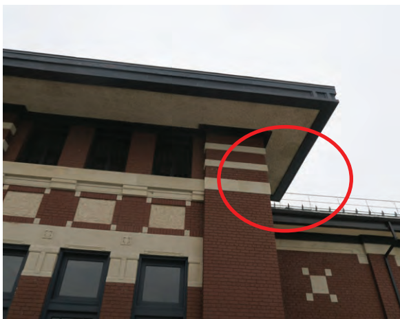
Sagging corner of the flat roof on the southeast corner of the entrance hall (ERA 2023)
