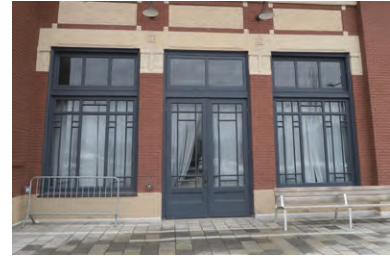
Dry and cracking wood doors on the south elevation of the entrance hall (ERA 2023)
