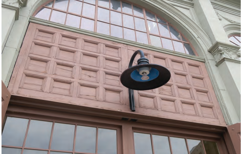
Original panelled transom over west entrance main doors. Note dry/split wood in panels (ERA 2023)
