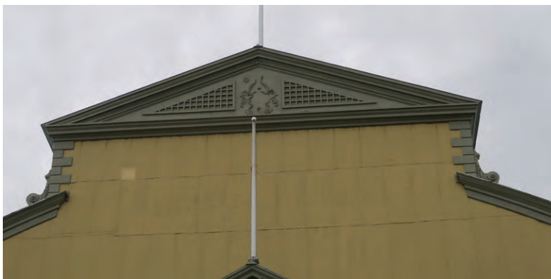
Dented metal panels edges and patches of repair above the east entrance pavilion (ERA 2023)
