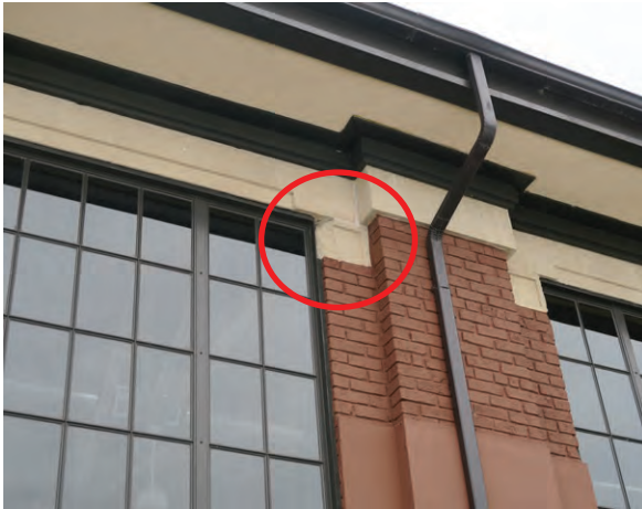
Chipped stone detail on east elevation (ERA 2023)
