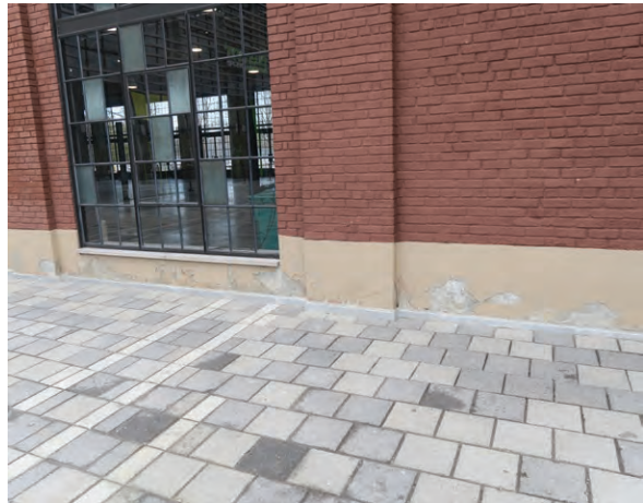
Delaminated material and paint flaking base on west elevation of exhibition hall (ERA 2023)
