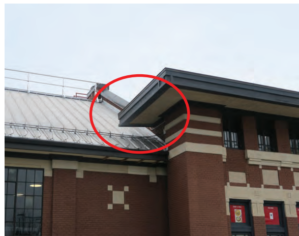
Sagging corner of the flat roof on the northwest corner of the entrance hall (ERA 2023)
