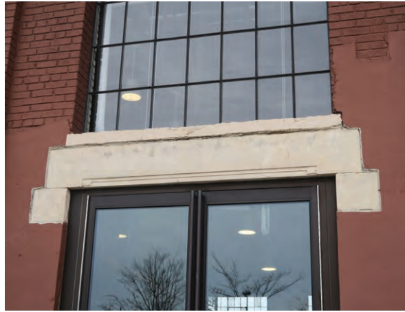
Delaminated and cracked stone sill and header on east elevation of exhibition hall (ERA 2023)
