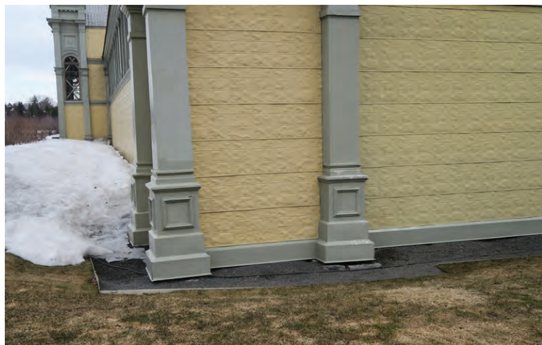
Northwest turret: damage sheet metal capital base (ERA 2023)
