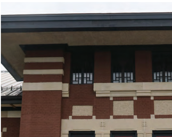
Missing stone window apron on west wing of the entrance hall (ERA 2023)
