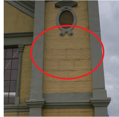
Rust present at perimeter of metal panels on northeast corner turret (ERA 2023)
