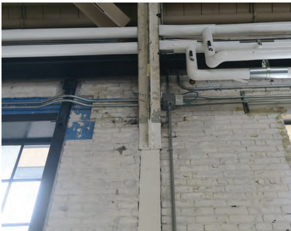
Deteriorating brick walls on the west wall of the exhibition hall at the truss (ERA 2023)
