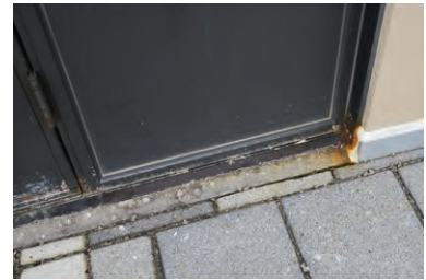
Rust damage on the bottom of the doors on the east elevation (ERA 2023)
