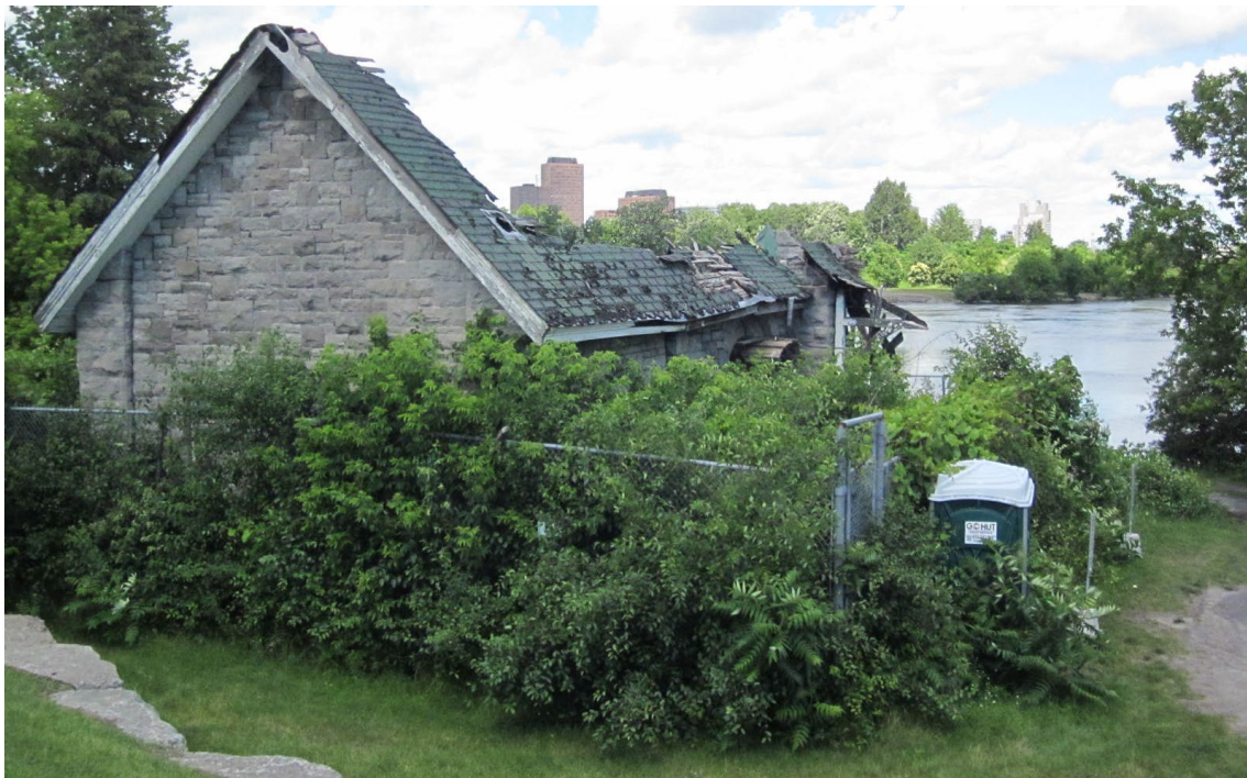
Existing conditions of the Hintonburg Pumping Station, as seen from Onigam Street (City of Ottawa, 2023).
