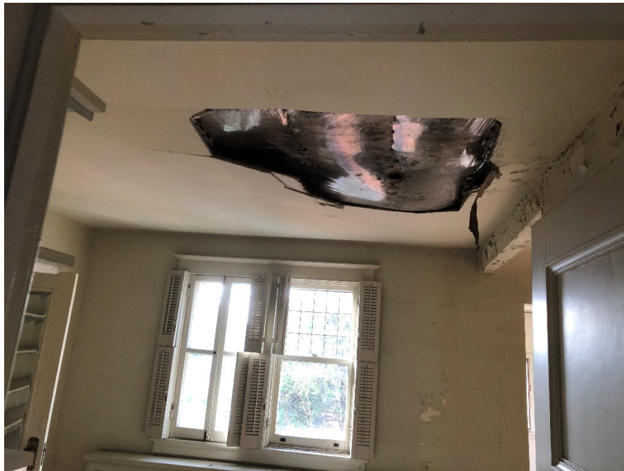
Photograph 2: Collapsed ceiling on second floor of 1112 Maple Road.
