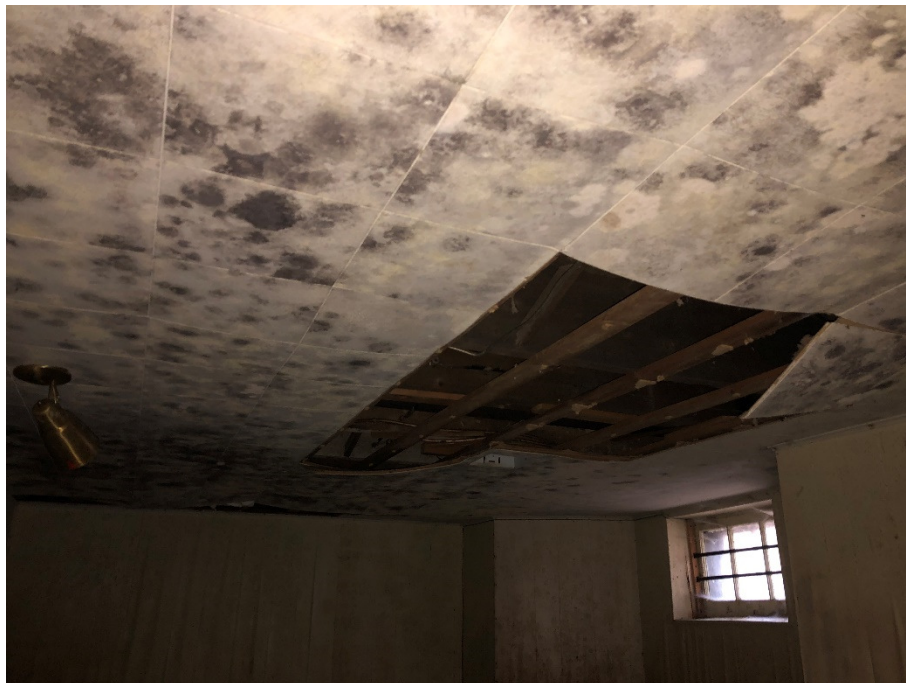
Photograph 6: Basement office of 1112 Lisgar Road showing extensive mould growth from moisture intrusion occurring on floors above.
