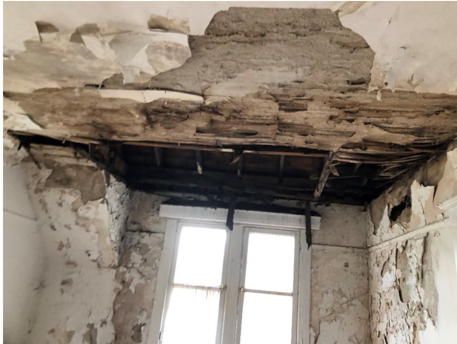
Photograph 9: Collapsed ceiling on ground floor of 1 Maple Lane due to moisture intrusion.
