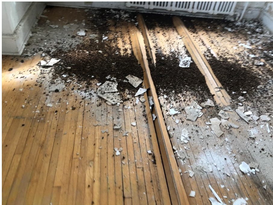
Photograph 10: Ceiling material from ground floor ceiling of 1 Maple Lane. Signs of significant water intrusion is shown from buckling hardwood flooring material.
