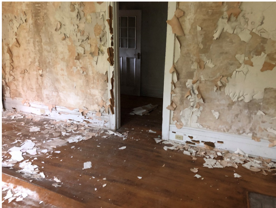
Photograph 8: Deteriorating walls on ground floor of 1 Maple Lane due to prolonged moisture intrusion.
