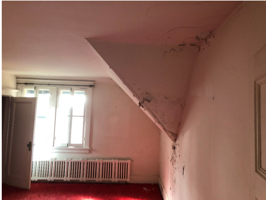
Photograph 5: Deteriorating ceiling and wall material from moisture intrusion on third floor of 1112 Lisard Road.
