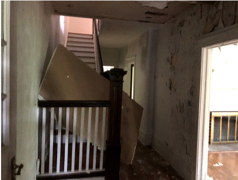
Photograph 7: Collapsed ceiling material on ground floor of 1 Maple Lane.
