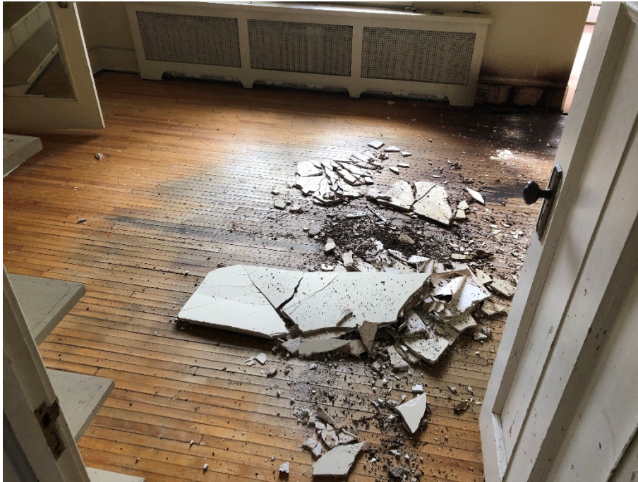
Photograph 3: Ceiling material from collapsed ceiling on second floor. Showing signs of moisture staining indicated cause of failure was from moisture intrusion.
