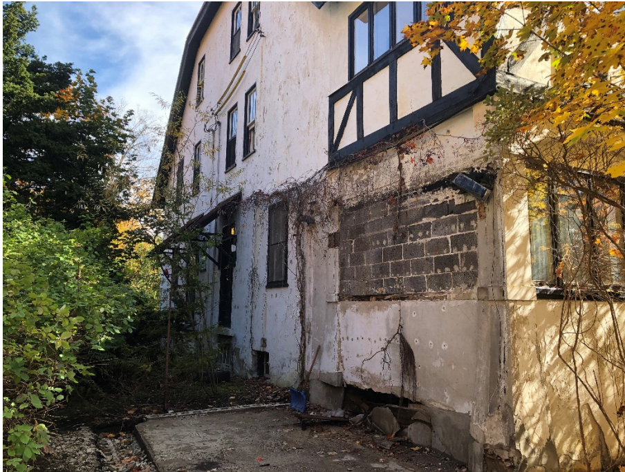
Photograph 1: Deteriorating façade on the north façade of 1112 Lisgar road.
