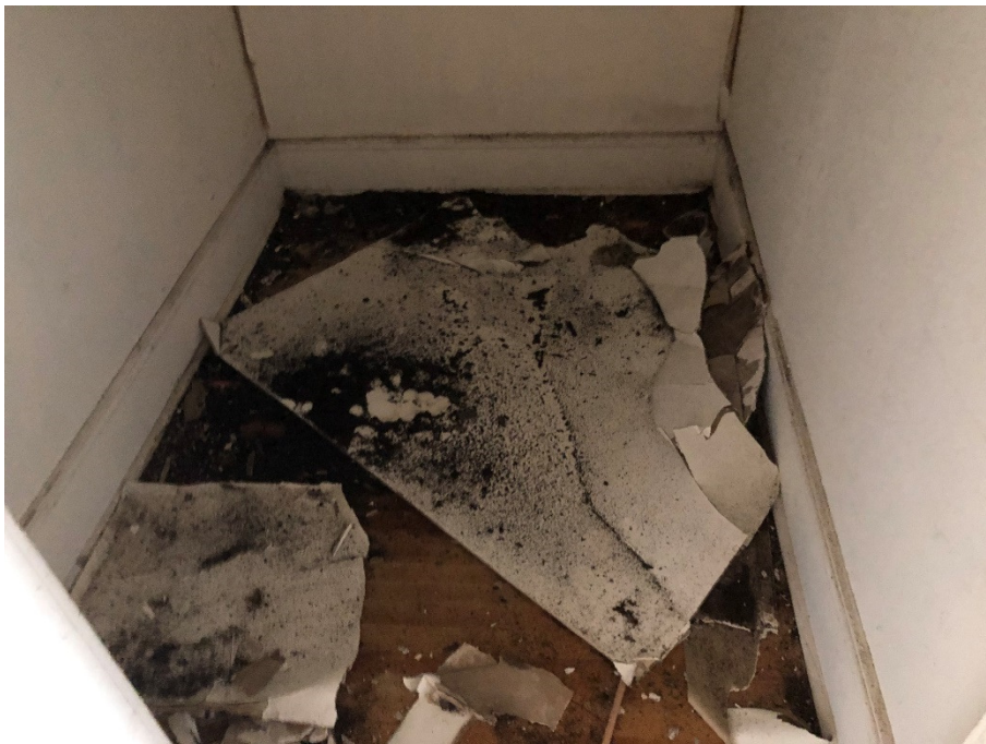
Photograph 4: Additional collapsed ceiling material within closet on third floor of 1112 Lisgar Road.
