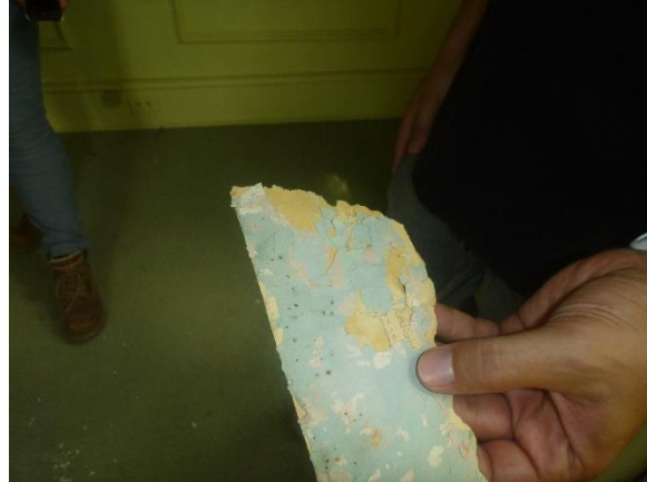
Photo 20: Mold noted on underside of ground floor ceiling wallpaper [JCAL 2021]
