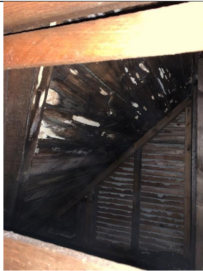
Photo 12: Roof water damage and mold within valley [JCAL 2021]
