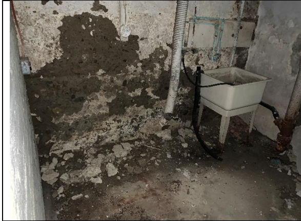
Photo 7: Concrete foundation damage and salt deposits [JCAL 2021]
