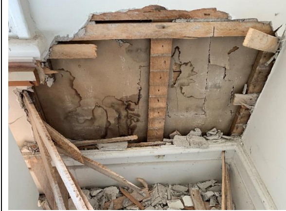
Photo 19: Ground floor wall opening- water damage and mold noted [JCAL 2021]
