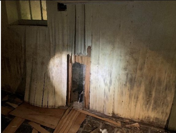
Photo 21: Typical extent of mold throughout basement [JCAL 2021]
