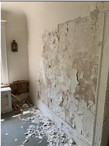
Photo 17: Ground floor west room water damage on interior wall [JCAL 2021]
