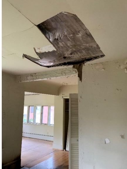
Photo 16: Second floor damage to ceiling finishes [JCAL 2021]
