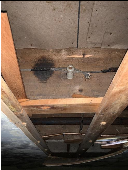
Photo 23: Mold noted on ground floor structure [JCAL 2021]
