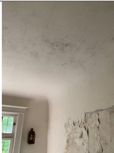
Photo 18: Ground floor west room mold on ceiling finishes [JCAL 2021]
