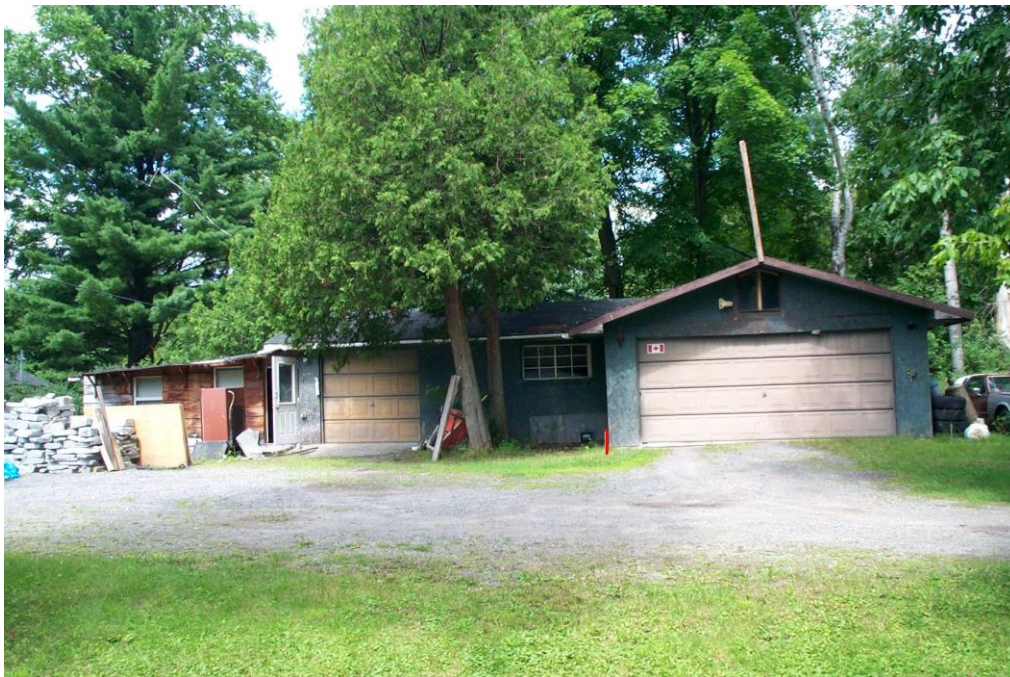
Figure 10 4120i Existing garage to be replaced, new garage SW corner at red stake.
