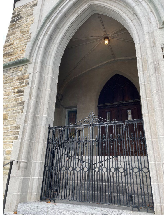
Ornamental Wrought Iron Gates at the Entrance Vestibule. Source: City of Ottawa
