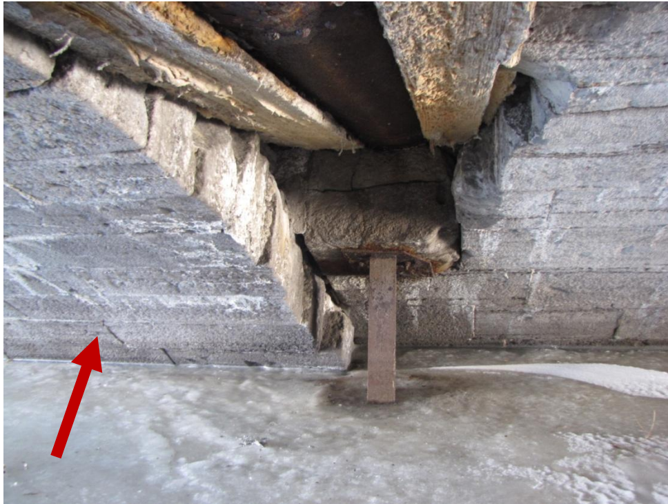
Figure 26: View (looking north) of the water pipe running along the arch added on the east side of the Old Booth Street Bridge. The stone arch of the original bridge is visible on the left side (arrow). Source: Parsons, March 2019.
