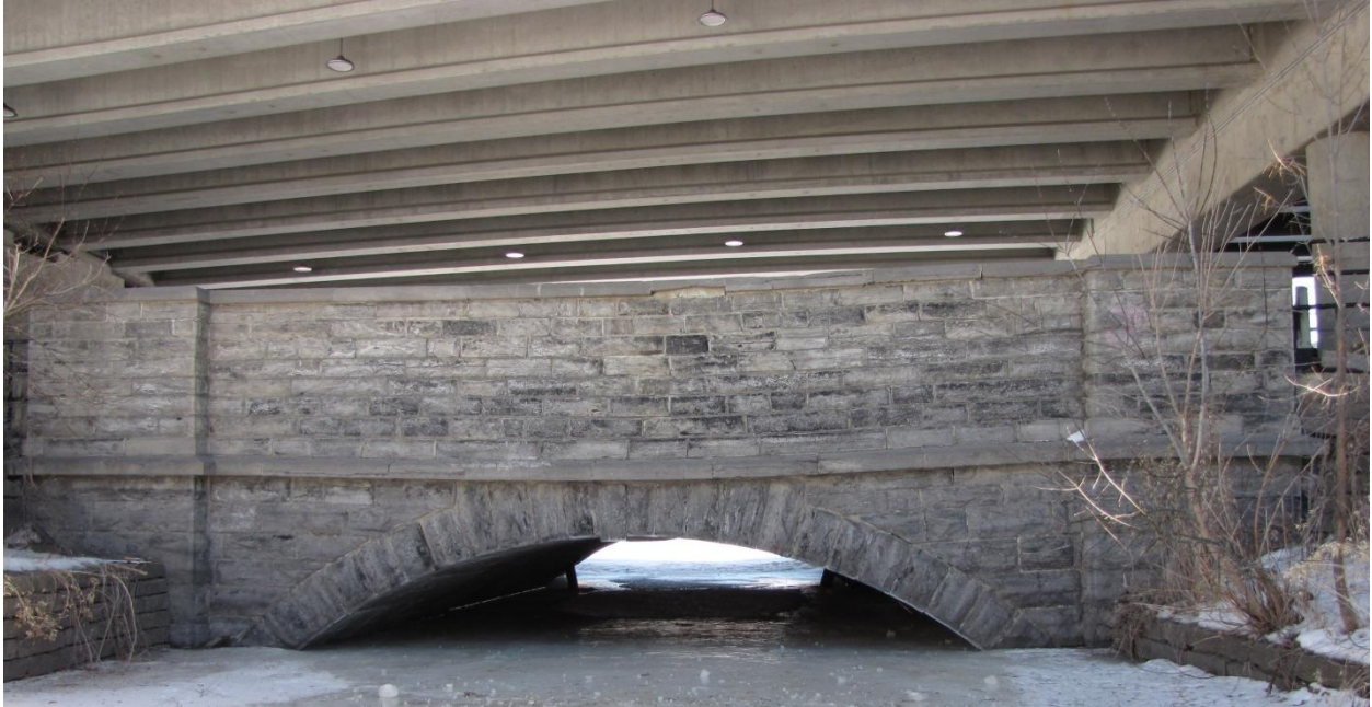
Figure 1: West arch and parapet of the Old Booth Street Bridge, March 2019. Source: Parsons.
