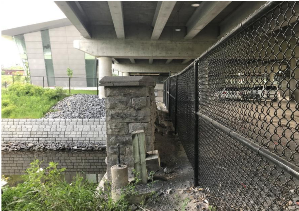
Figure 25: Looking south towards the east parapet of the Old Booth Street Bridge, June 2019. Source: Contentworks.
