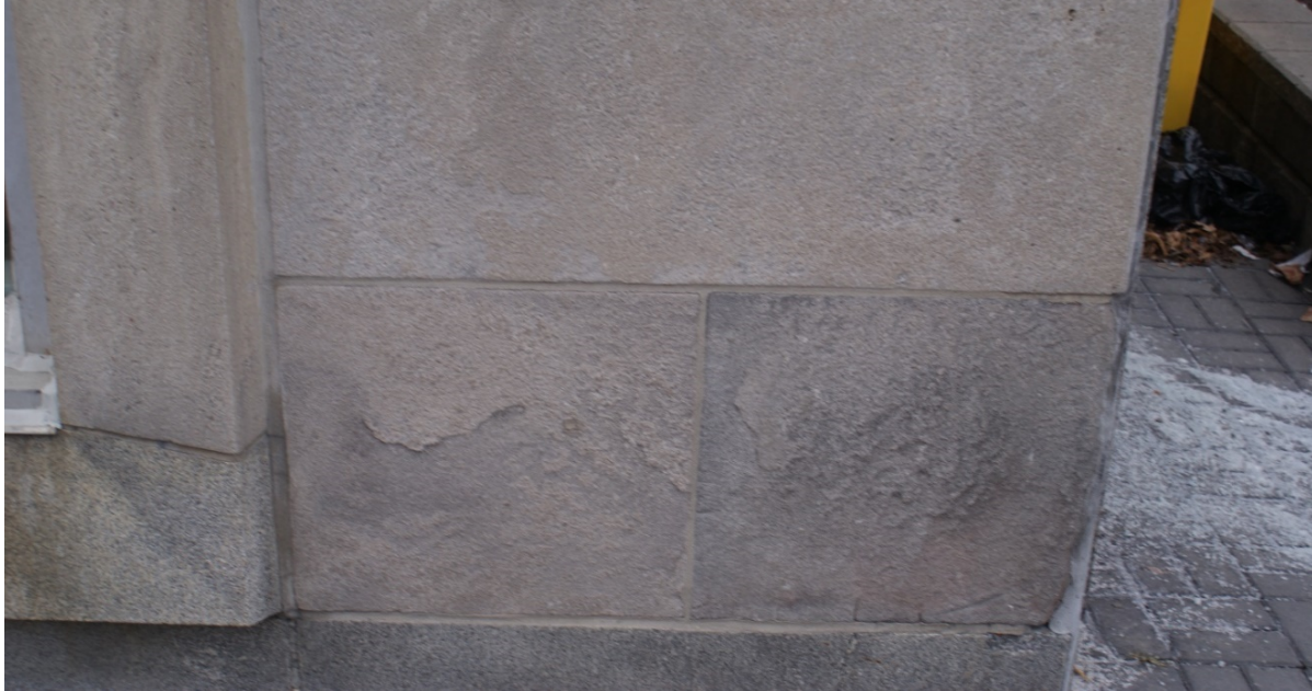
Figure 22: Detail view at the base of the wall at the south-west corner. The surface of the two Niagara limestone panels at the base of the wall are scaling due to de-icing salts. The granite plinth course is evident at the bottom of the photo. The Niagara limestone window surround is the vertical element to the left and a granite windowsill/surround below. Source: Commonwealth 2022.
