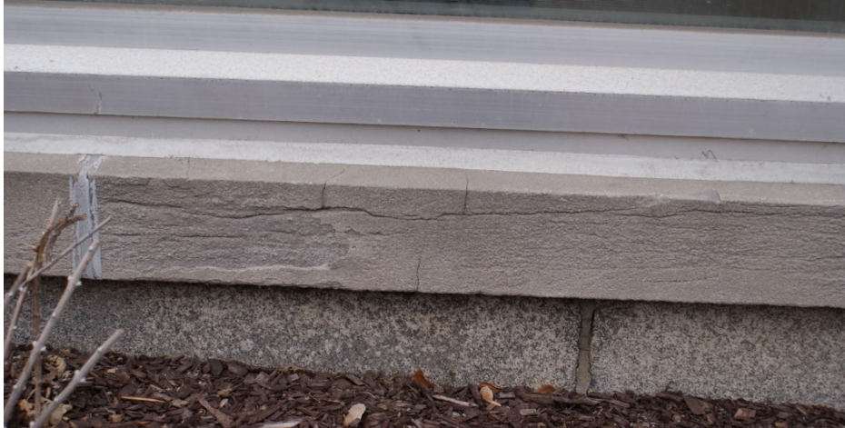
Figure 20: View of a deteriorated limestone windowsill and the granite plinth course below. The cleavage planes within the limestone sills are evident where the sawn surface has weathered. The cleavages planes follow the layers of deposition of the sedimentary rock. Source: Commonwealth 2022.
