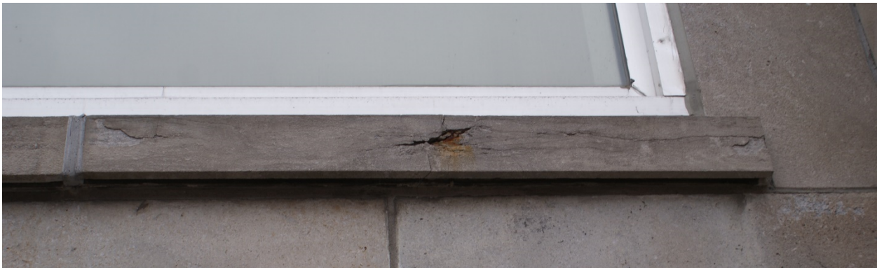
Figure 21: View of a deteriorated limestone windowsill. The cleavage planes within the limestone sills are evident where the sawn surface. The cleavages planes follow the layers of deposition of the sedimentary rock. Source: Commonwealth 2022.
