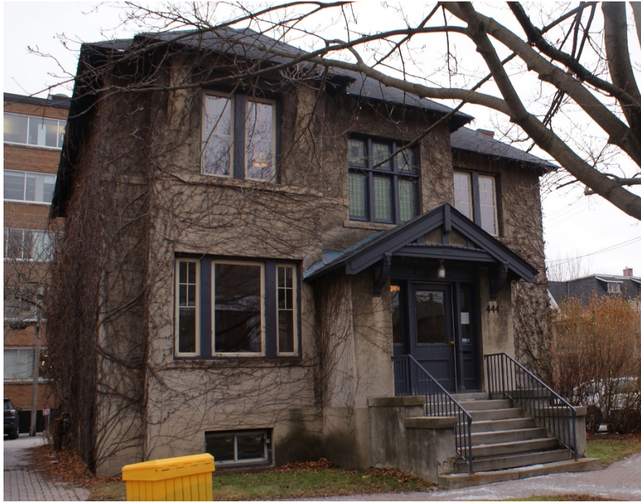
Figure 36: View of 444 MacLaren Street. The stuccoed exterior wall is covered in vines that should be removed before they have an adverse impact on the stucco finishes. Source: Commonwealth 2022
