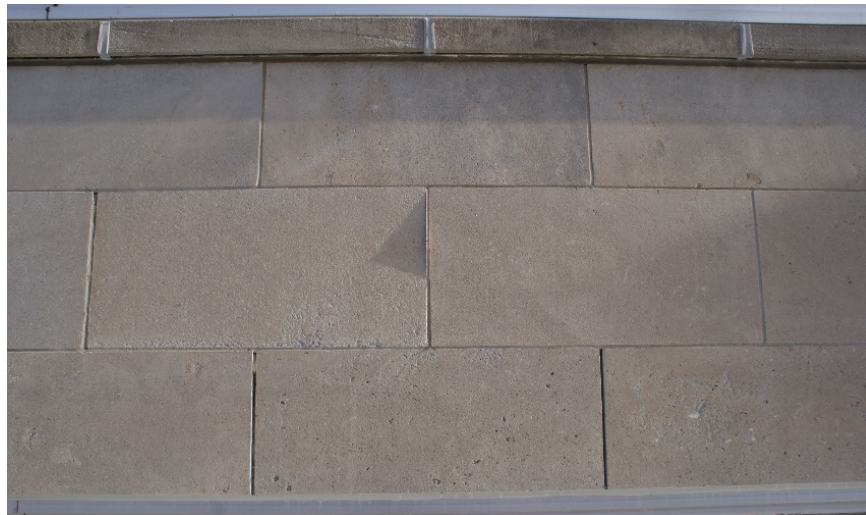
Figures 13: View of the Niagara limestone cladding above the Kent Street entrance. Note the variations in the material, coursing, and the windowsill course band the length of units corresponding with the cladding coursing. Mortar is missing from a number of joints. Source: Commonwealth 2023.
