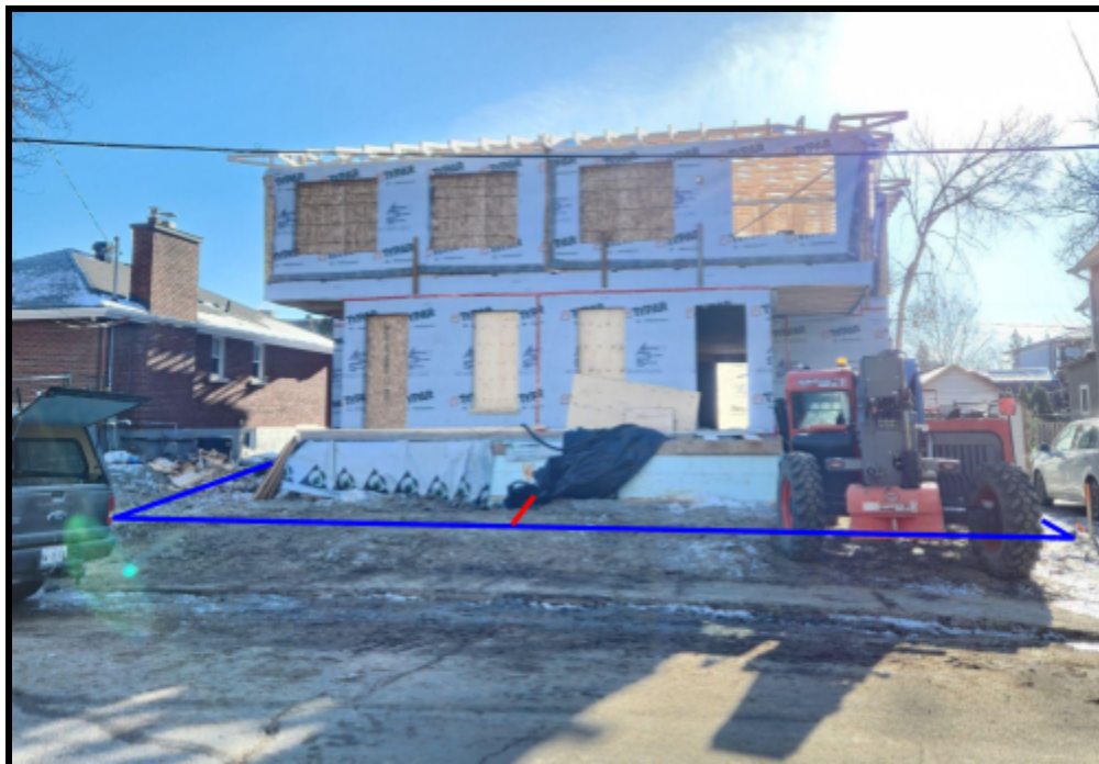
Image of the subject property under construction showing the lot boundary and proposed severance line.
