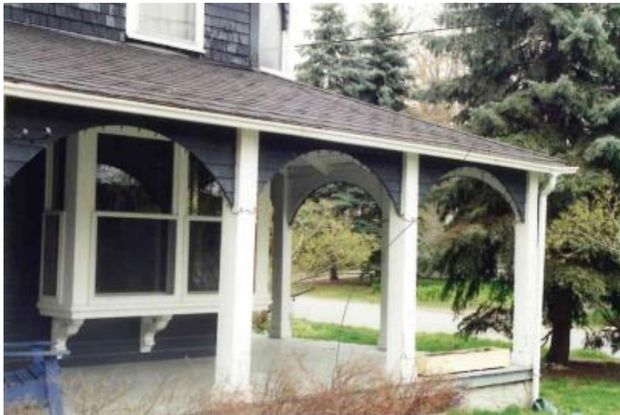
West façade arched spandrels and box bay window, Source: Tumak and Horwitz, Heritage Survey and Evaluation Form, 1996
