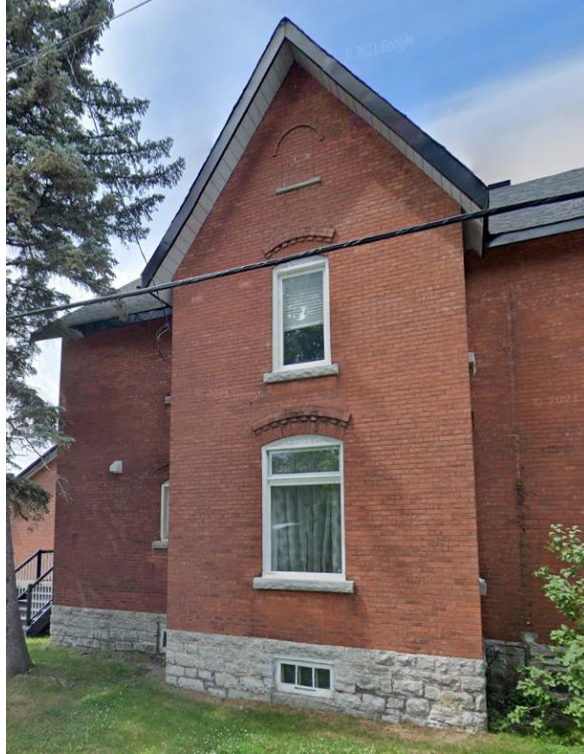
2764 Rowatt Street, east gable end, Source: Google Maps, 2021. Note: vertical stain on the wall correlates to likely water damage from a downspout seen in the 1961-65 photo
