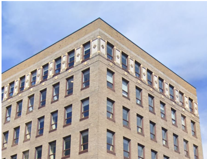
Brickwork detailing on top storey with top cornice removed, 2021. Google Maps , 2021.
