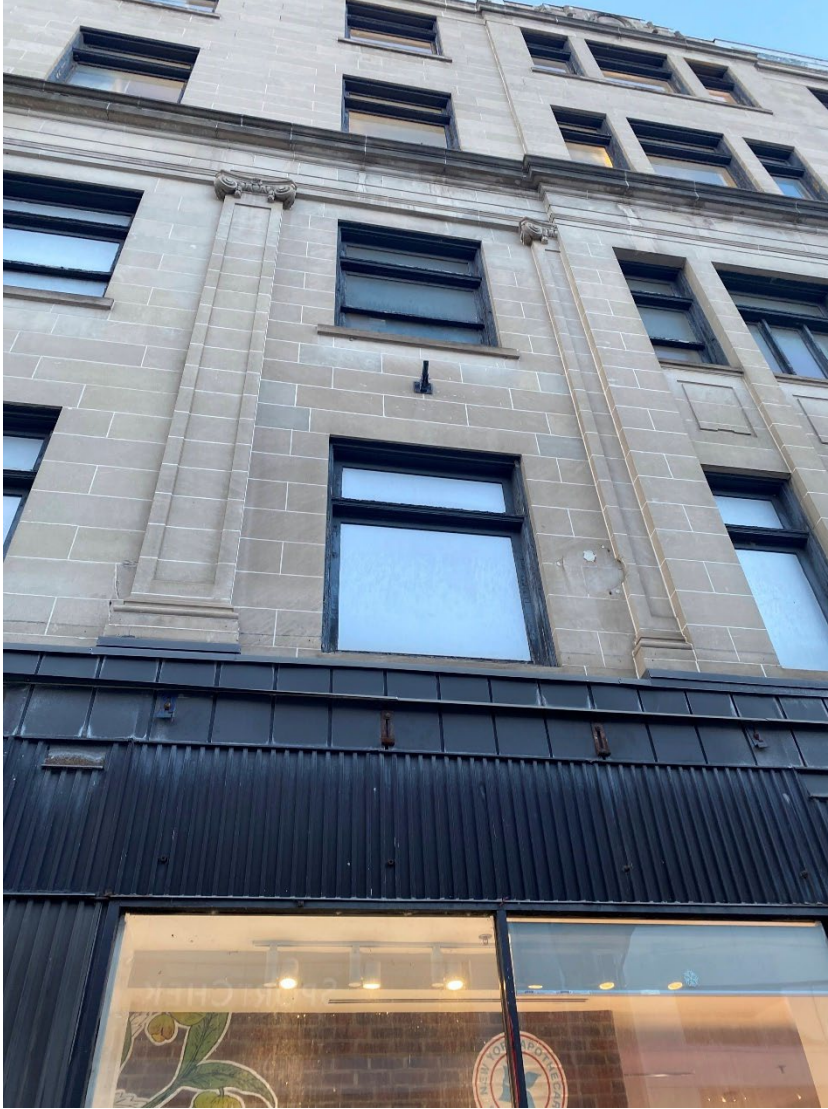
Close of up the stone pilasters and detailed capitals. City of Ottawa, 2024.
