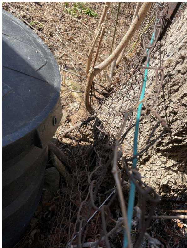
Figure 6: Base of Manitoba maple (tree 3) growing into metal fence and post
