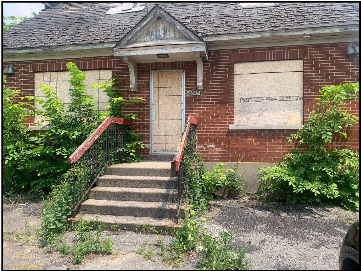
Image of the front facade of the existing building to be removed which was damaged by a fire in August 2021.
