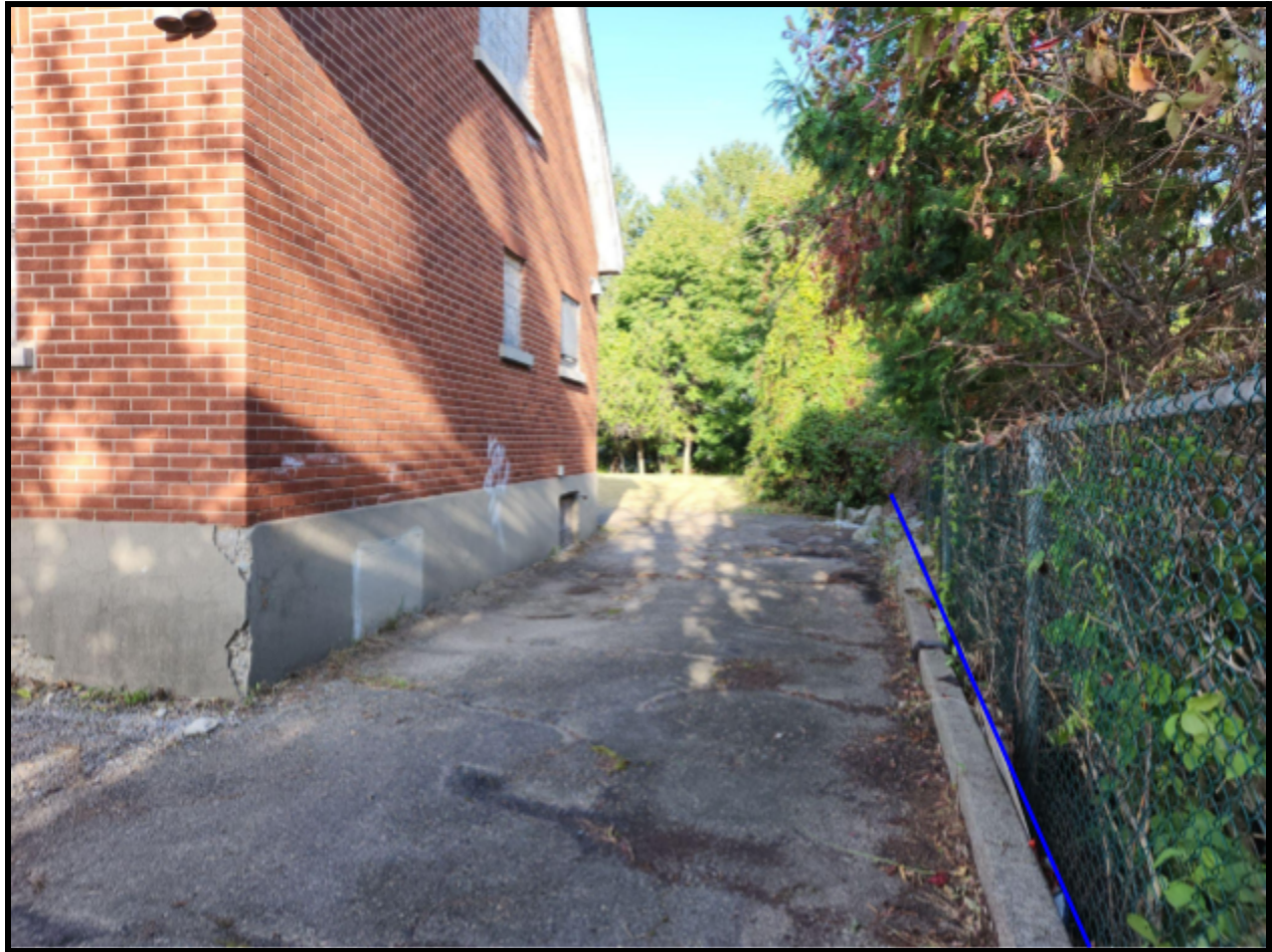
Image showing the existing south interior side yard conditions of the subject property and the existing driveway whose location is to be maintained.
