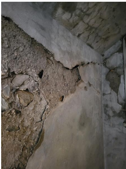
Foundation Wall Deterioration
