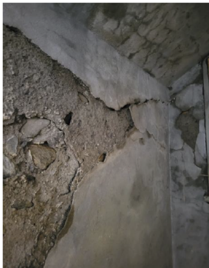
Foundation Wall Deterioration
