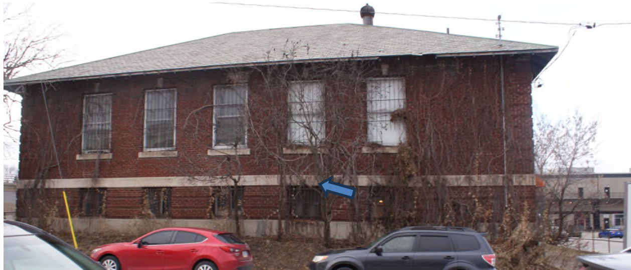
Figure 9: View of the east elevation. Note: The deflection/settlement in the string course extending from the second window from the right to the north-east corner (right corner). Stepped cracking is evident in the foundation, extending up to the windowsills through to the roof. The gauged brick forming the header above one window is missing, and brickwork at the north-east corner is displaced below the roof. Source: Commonwealth, December 2023.
