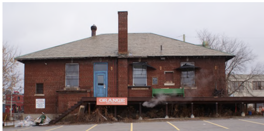
Figure 6: View of the west elevation. The architectural pre-cast stone string course and rusticated brick finish below extends to the small brick basement bump out. Source: Commonwealth, December 2023.
