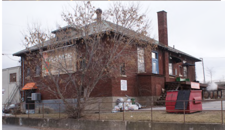
Figure 7: View looking southeast to the west and north façades. The retaining wall and tubular metal railing would appear to date to the early 1960s site development. Note the grassed area. Source: Commonwealth, December 2023.
