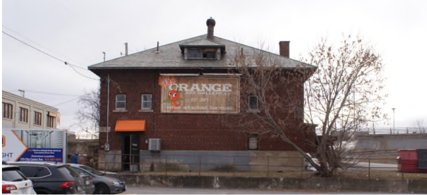
Figure 8: View of the north façade. Note the step cracking in the brickwork above the window at the north-east corner above the basement entrance. Note the grassed edge and tree. Source: Commonwealth, December 2023.
