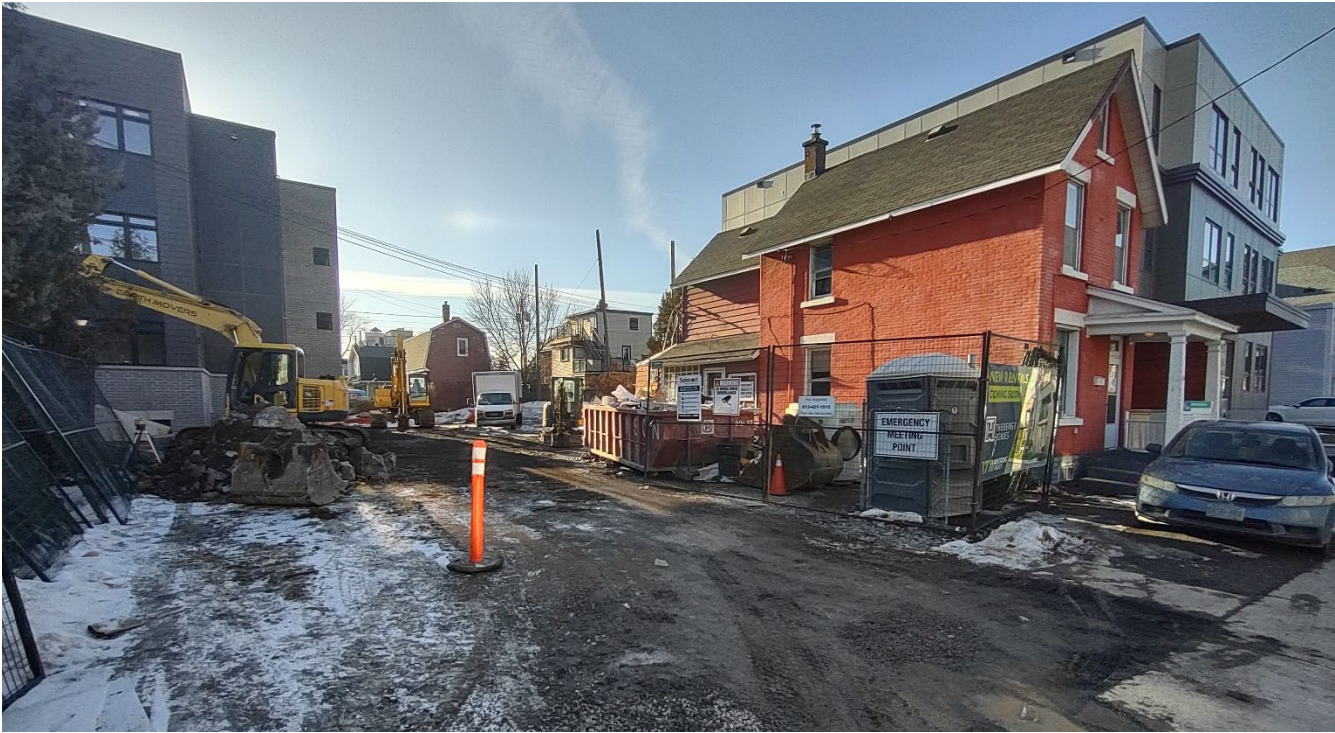
Figure 5. Looking northwest at the subject property where the proposed low-rise apartment dwelling is proposed to be constructed.
