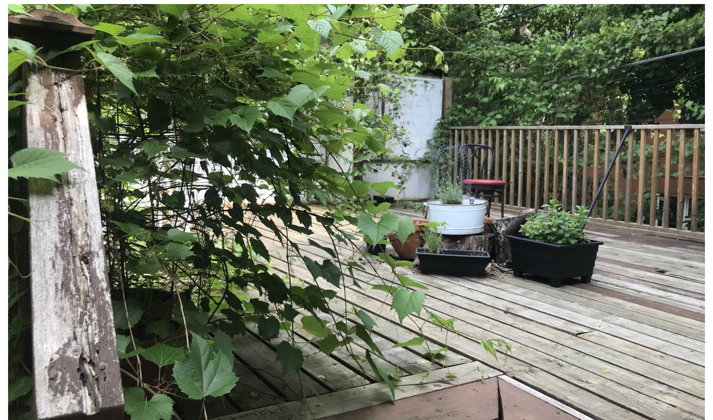
J) View of the existing roof top deck looking towards the North corner.
