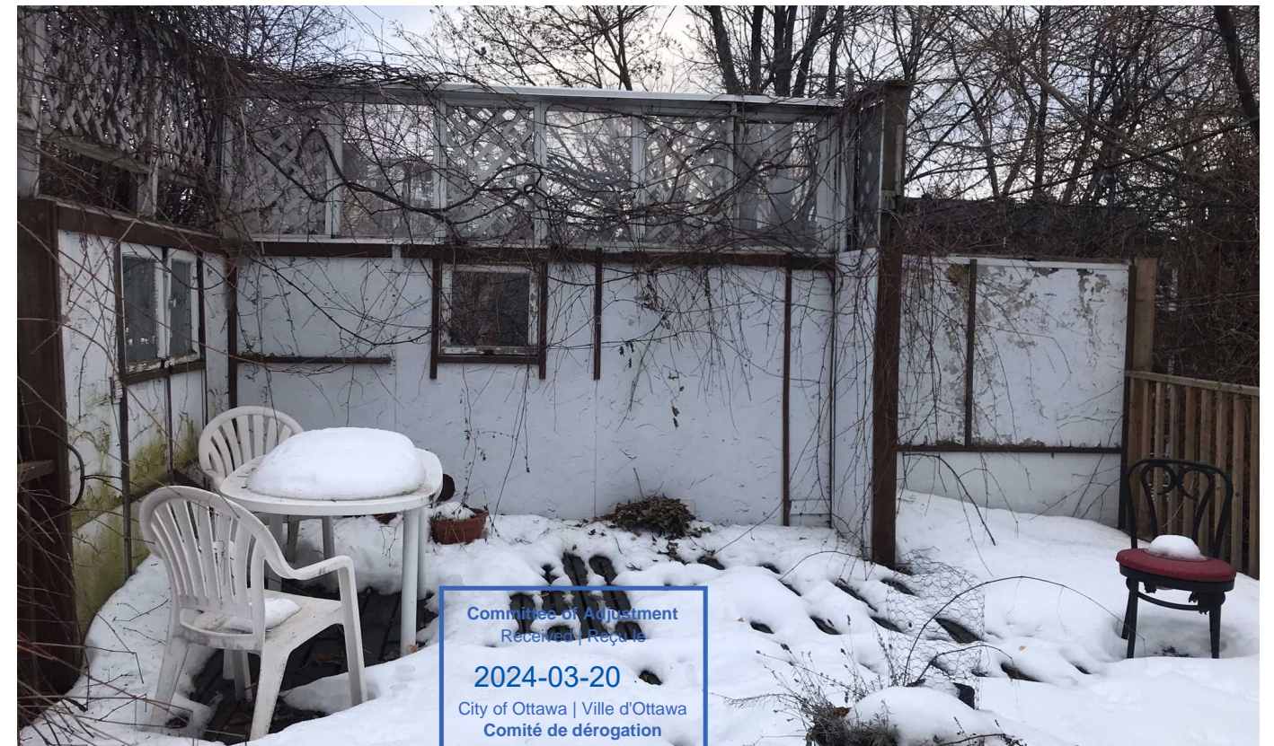
T) View of the roof top deck privacy screen at the North corner of the property.
