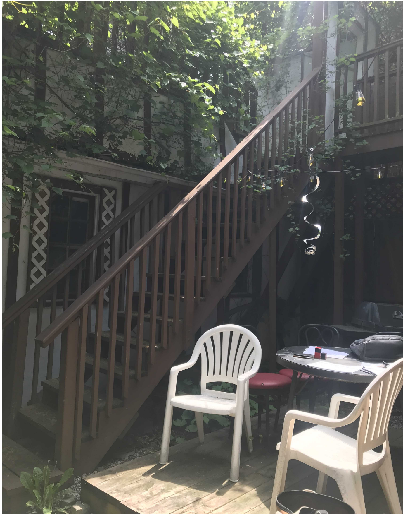
F) View of the exterior stairs to the roof top deck and elevated walkway.
