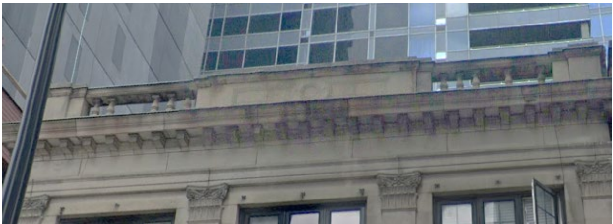
Balustrades and a parapet above the roofline at 217 Rideau Street. Google Maps , accessed 2024.
