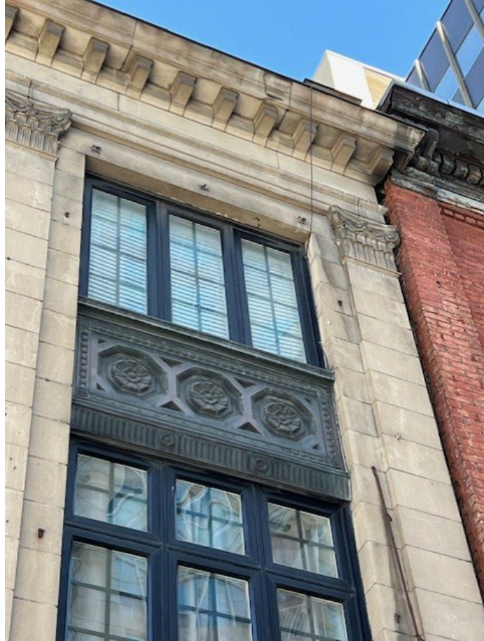
Detailing on 217 Rideau Street including a metal spandrel panel, ornate carved capitals, and dentilled cornice. City of Ottawa , 2024.
