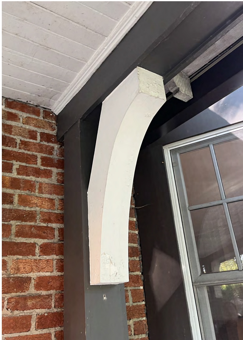
2 EXISTING PORCH DECORATIVE BRACKETS FOR REPLACEMENT
