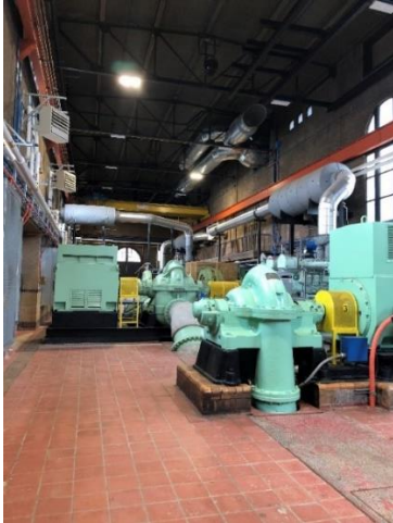
Pumping Station interior
