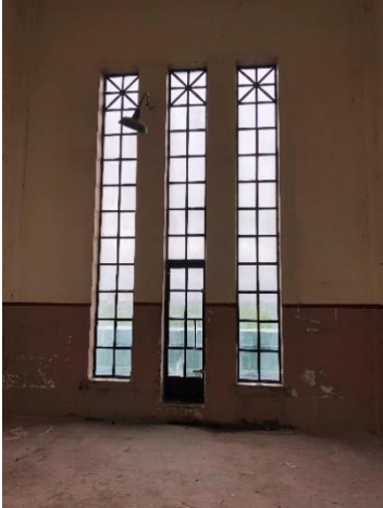
View from inside the Chemical Building Tower, showing the square window pattern also found in the earlier Pumping Station
