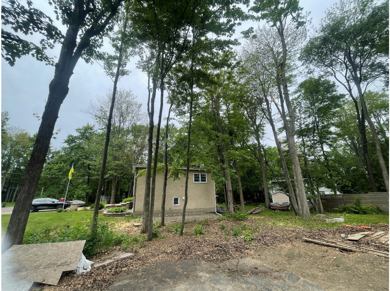
Figure 1: Picture showing area of asphalt where the new addition will be going, and the trees in the background. Picture taken from the centre of the property facing west
