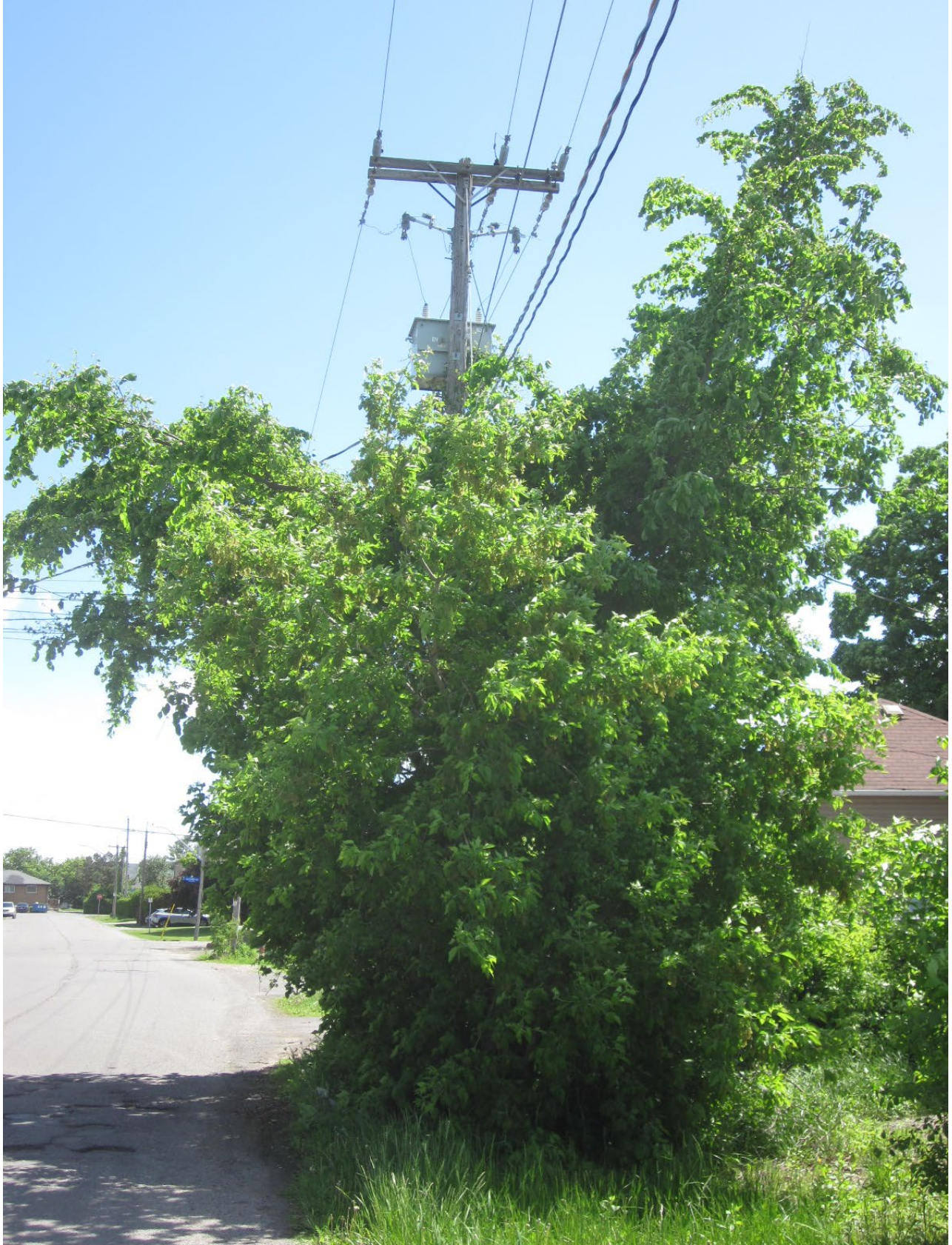
Picture 1. Tree #1, city white elm at 1353 Gosset Street.
