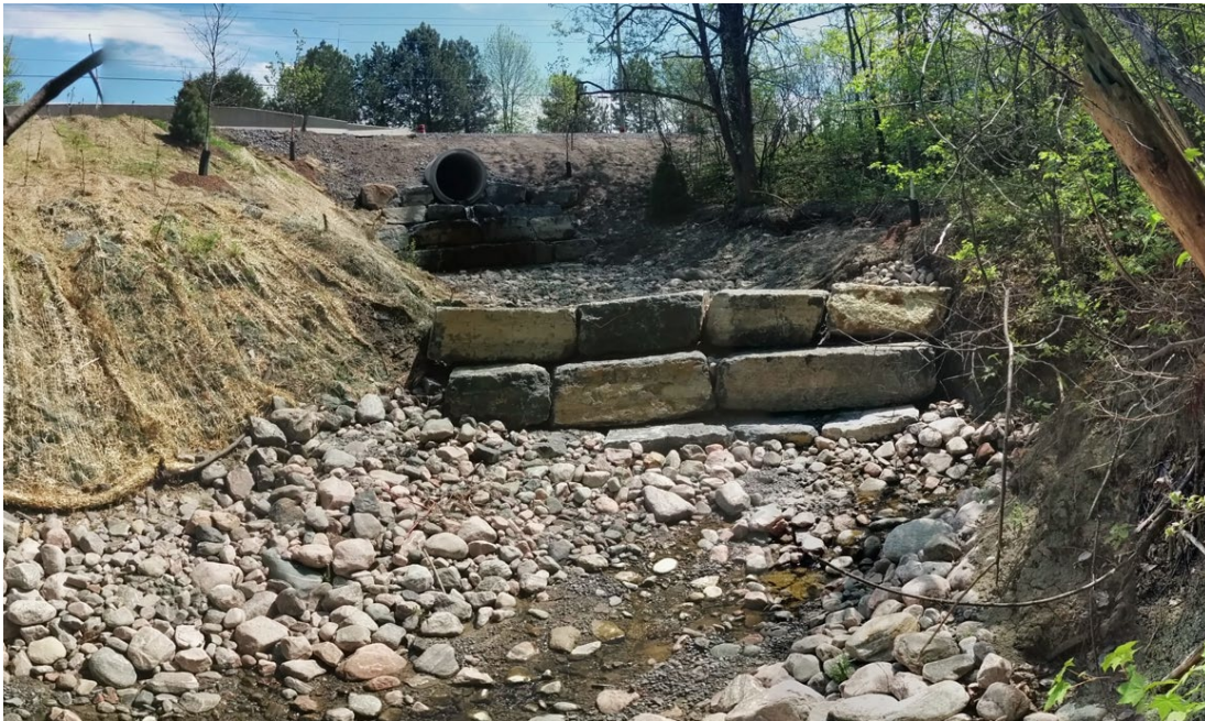
Figure 5.7. Creek Control Structures, Courtesy Coldwater Consulting
