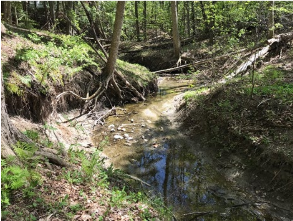
Figure 3.9. Eroded banks and the roots of an established tree have been exposed
