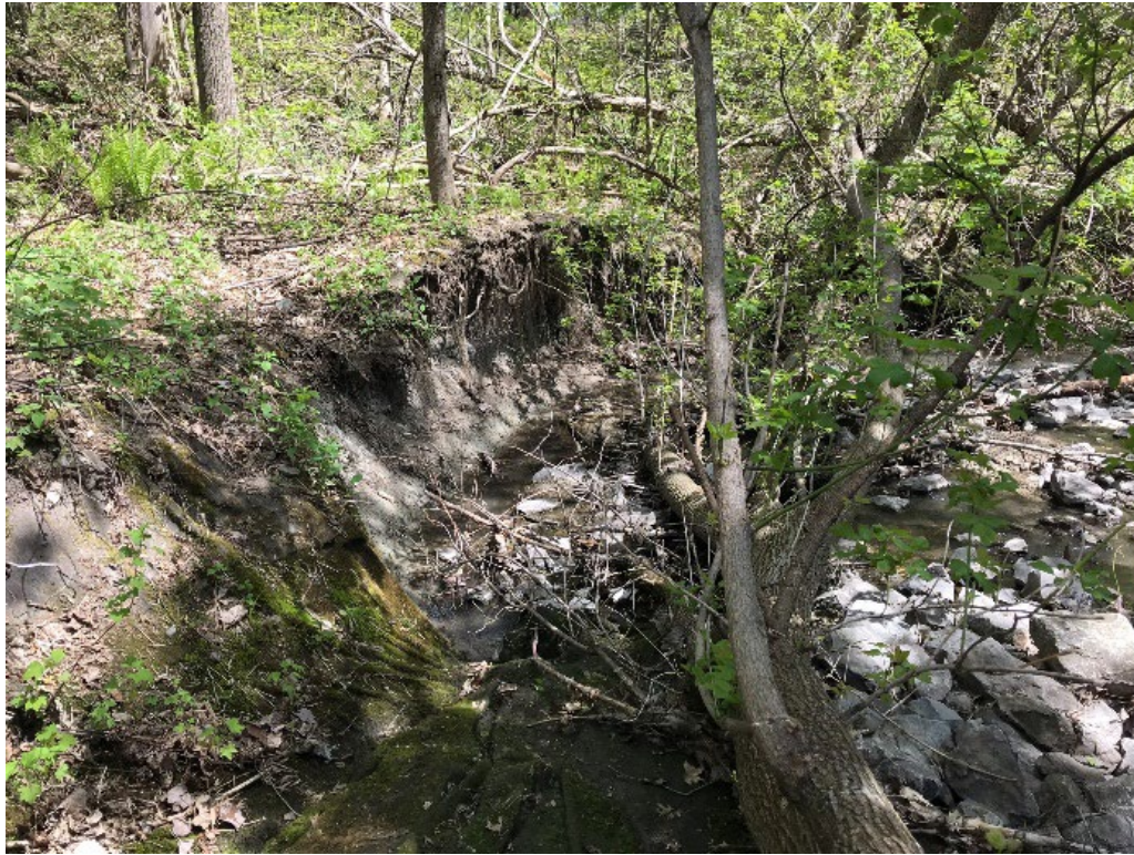
Figure 3.7. The left bank is eroded, located in the upper reach of the channel
