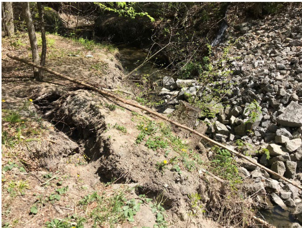
Figure 3.8. Failure of the left bank opposite a rip rap protected slope
