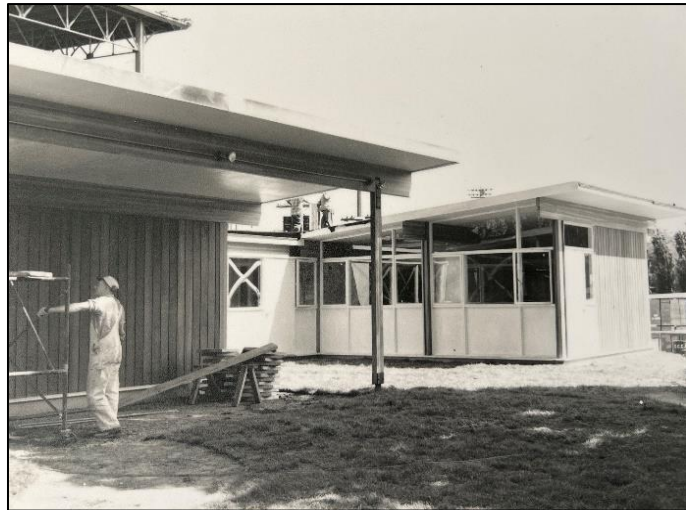
The 1958 lottery home under construction at the display site at Lansdowne Park before being moved to 8 Robert Kemp Street. Source: Current property owner.
