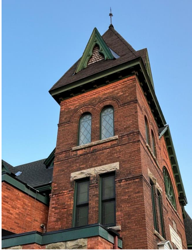
Coloured and leaded glass, and wooden detailing on the church's north tower roof. City of Ottawa, 2024.
