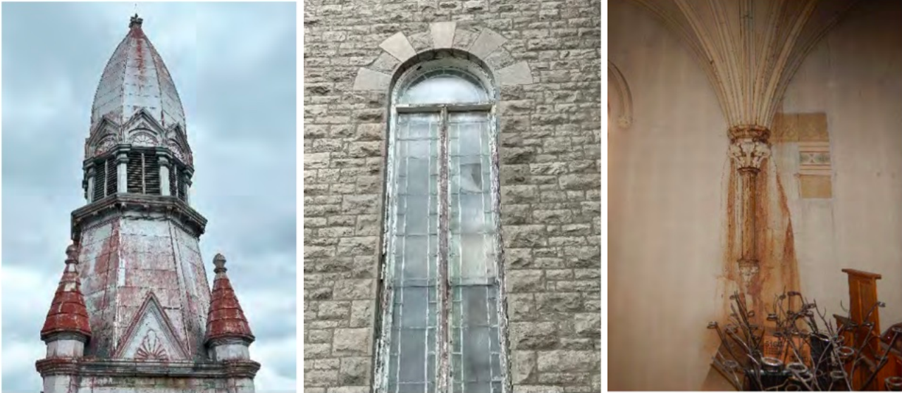
Figures 3,4,5: Selected images from St Brigid’s Building Condition Report showing deterioration. RMA+SH Architects/John Cooke & Assoc Structural Engineers (2023)
