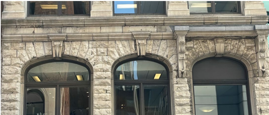
First storey showing carved stone keystones and cornice brackets, as well as rusticated stone cladding. City of Ottawa, 2024.
