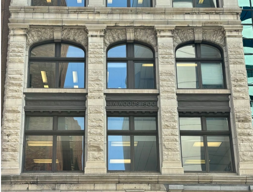
Second and third storey window openings featuring inscribed spandrel panel. City of Ottawa , 2024.
