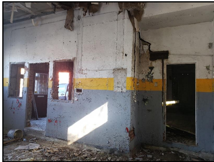
Interior wall with major crack/displacement at door openings
