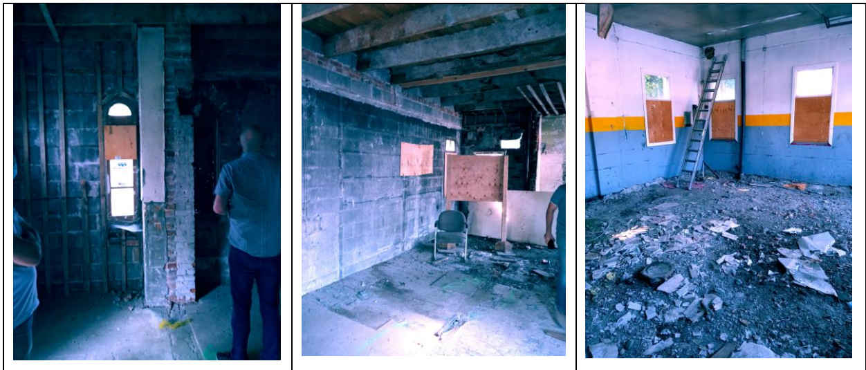
Figure 6: Interior views illustrating the condition, with the interior stripped down to the block walls.
