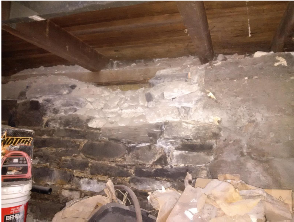
Photo Three – Dry Rot on Wood Framing
