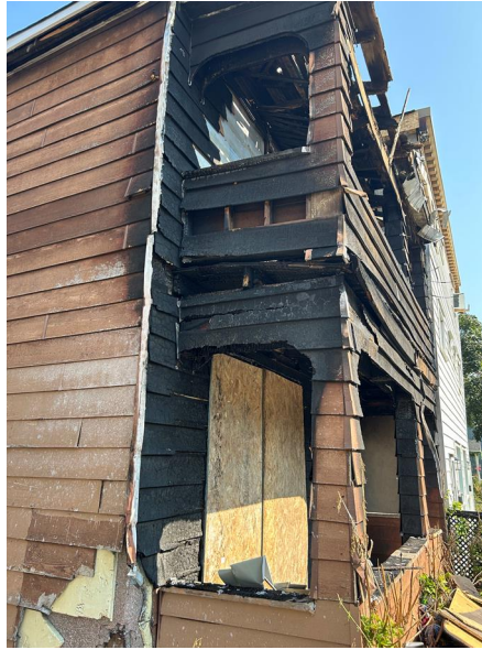
Photo Eight Fire Damage
