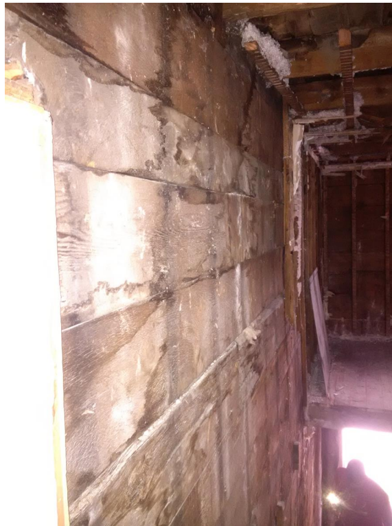
Photo Seven – Out of Plumb Wall/Water Infiltration
