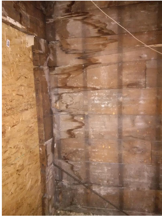
Photo One – Moisture Penetration
