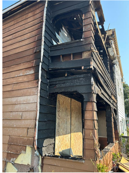
Photo Eight Fire Damage
