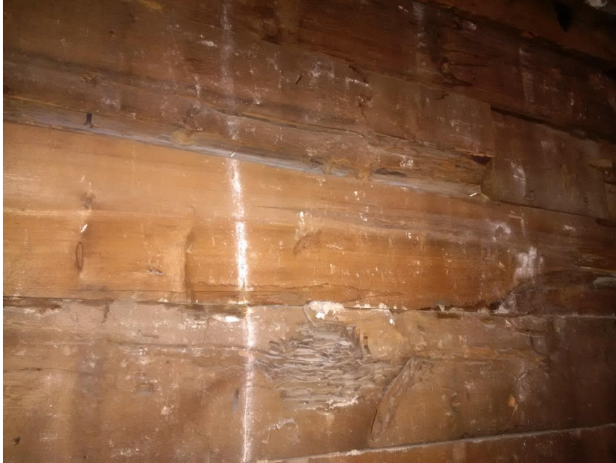
Photo Six – Carpenter Ant Damage
