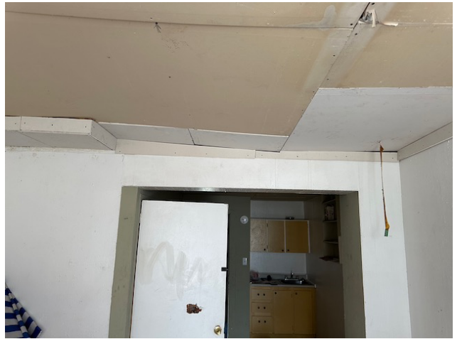
Photo 3 – Sagging Floor Joists Above (227/229)
