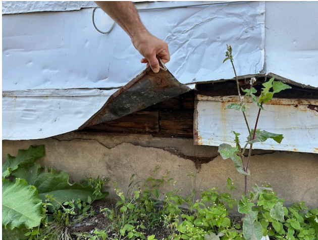
Photo 9 – Rotting of Wall Lumber (231/233)
