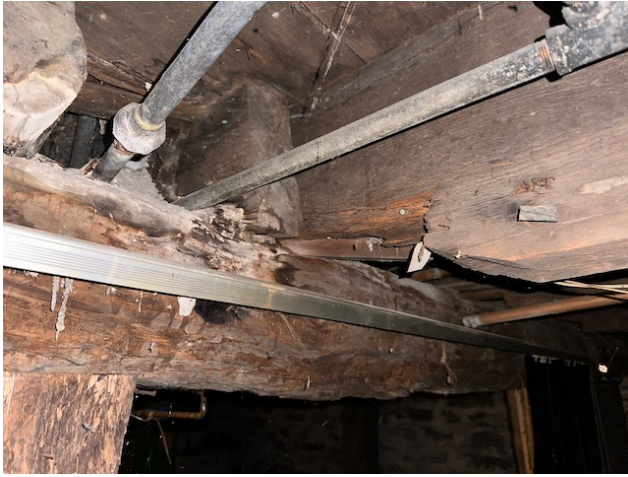
Photo 1 – Rotting Basement Joists (227/229)
