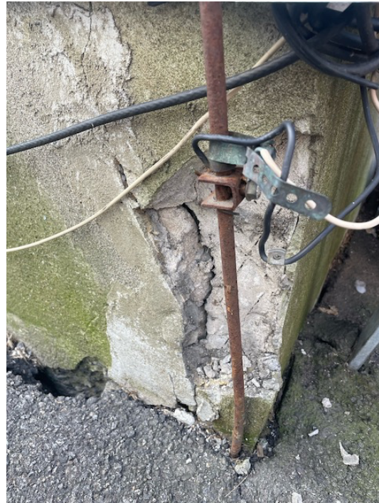
Photo 10 – Foundation Wall Cracking (231/233)
