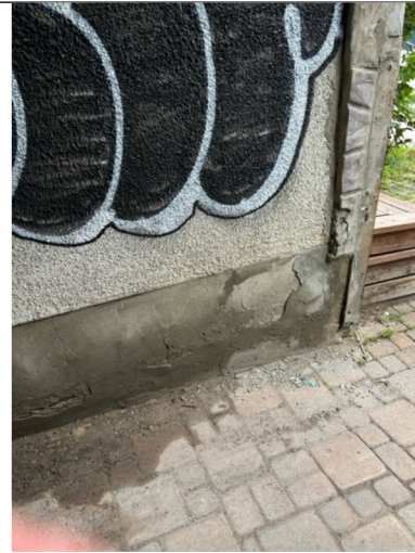
Photo 6: Cracking in back of veneer.
