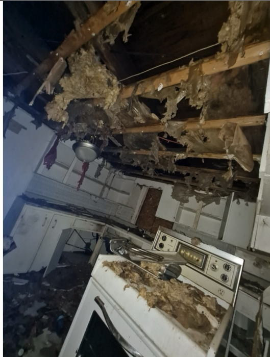
Photo 46: Ceiling and insulation have been
