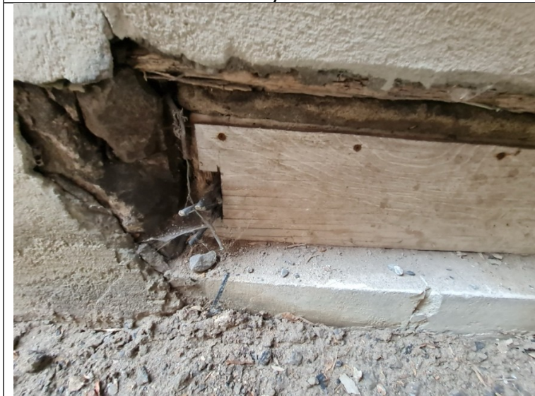
Photo 7: Foundation wall deterioration.
