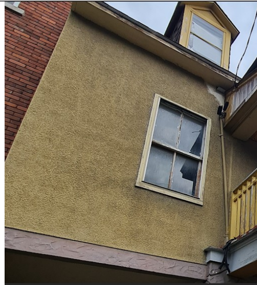
Photo 2: Front Stucco weathering & staining.
