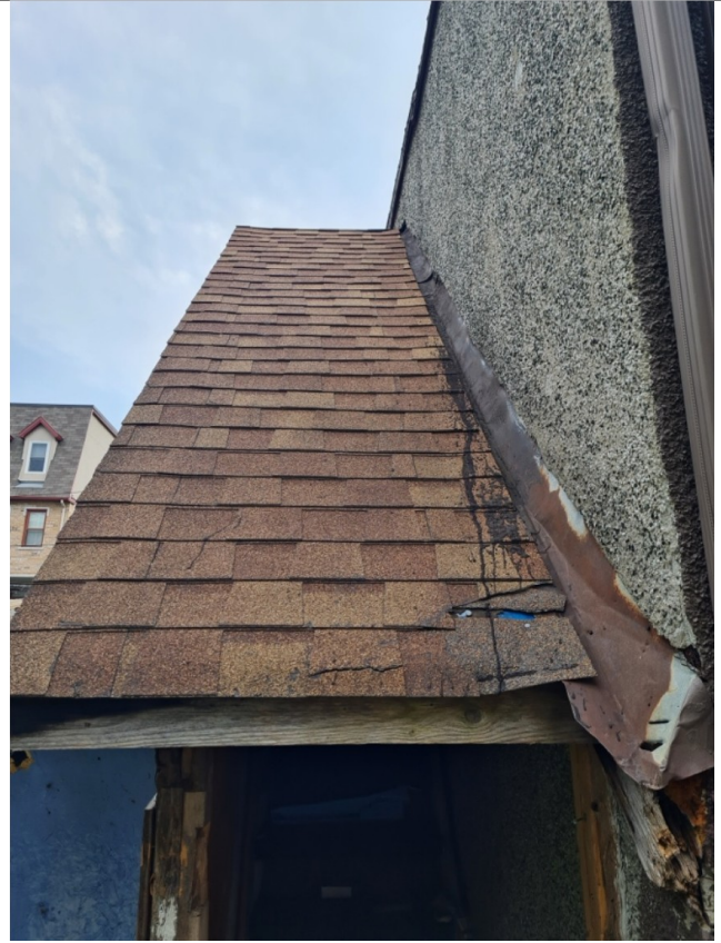
Photo 43: Poor flashing detail, corroding away.
