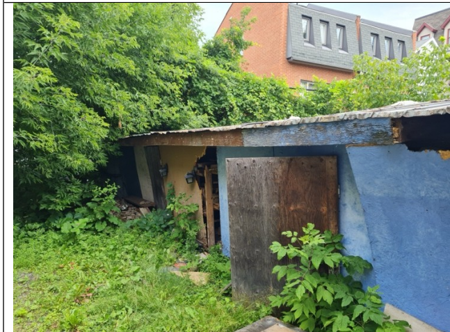
Photo 32: Shed is visibly settling and leaning.
