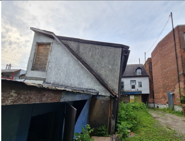
Photo 36: Addition wall leaning dramatically. Unstable structure in state of active collapse.
