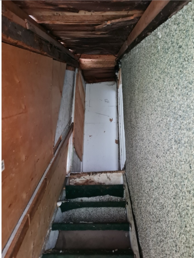
Photo 42: Timber appears weathered. Staircase is slanted.
