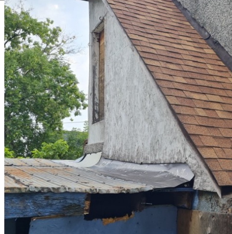
Photo 35: Corrosion of roof sheathing.
