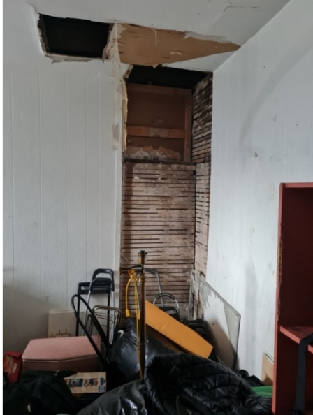
Photo 20: Exposed lath and a hole in the ceiling.
