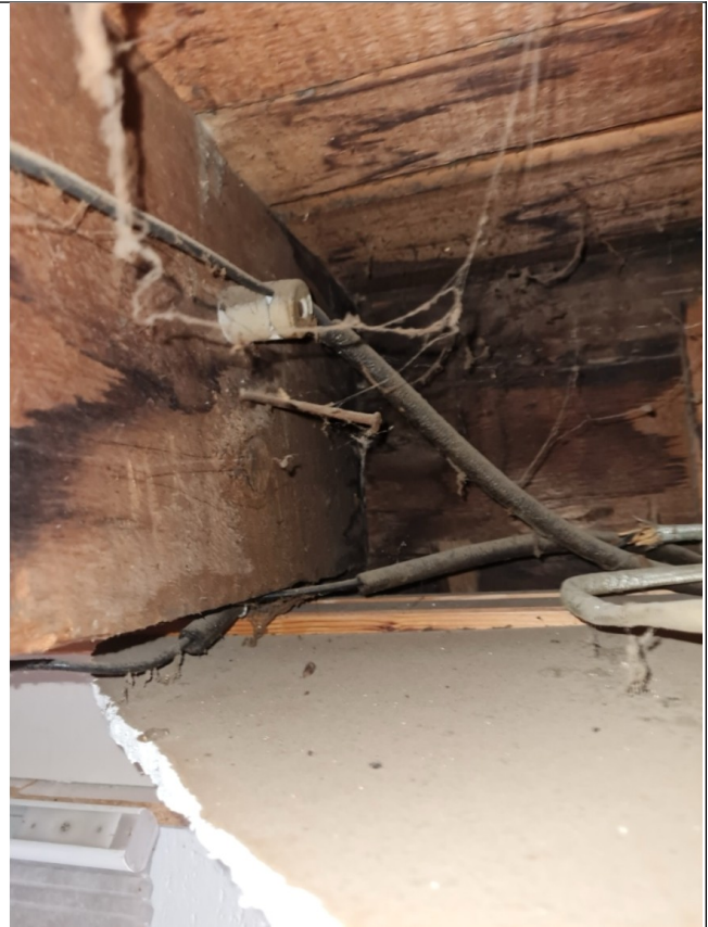
Photo 19: Dark stained joists and rim board in the second floor plenum at the front (South) wall of the building.
