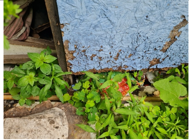
Photo 31: Shed lacks a foundation, bearing on water damaged areas. The paint is peeling, indicative of weathering of the wood.
