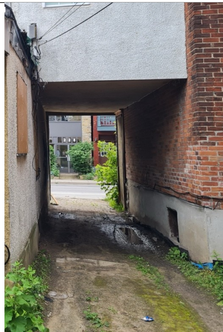
Photo 4: Laneway covering is slanted.
