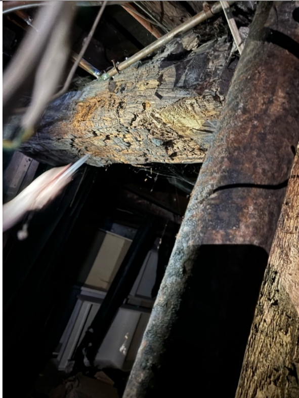
Photo 16: Severe deterioration of beam due to rot.
