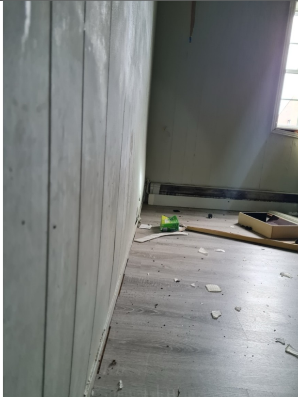
Photo 22: Interior wall bulge and sloped floor above laneway below.
