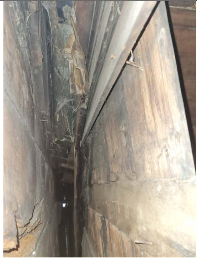
Photo 25: Inside of wall showing signs of decay along both structures. Daylight observed on all sides.
