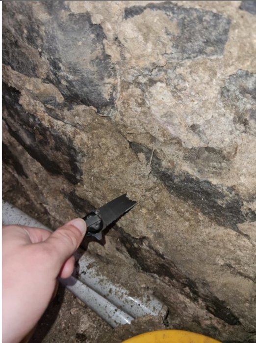
Photo 10: Weak mortar. Field Knife penetrates easily.
