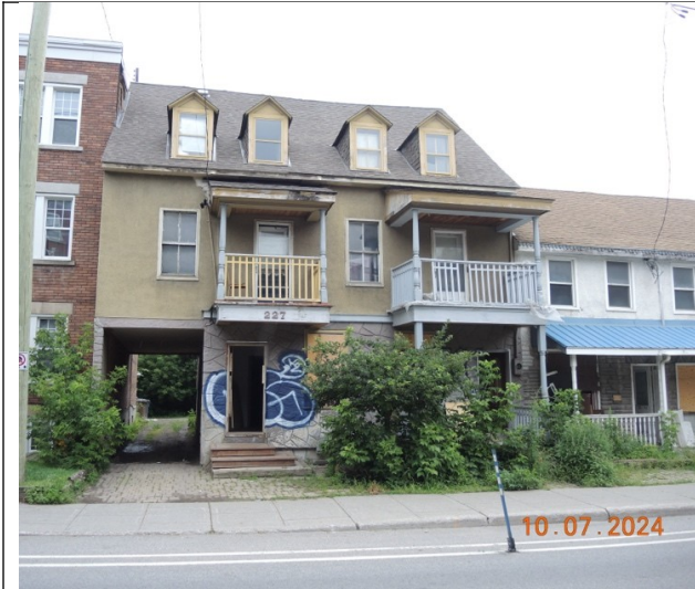
Photo 1: Paint peeling and weathering of wooden elements.
