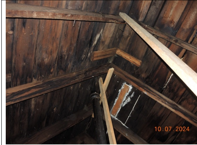
Photo 26: Dark staining in roof by plumbing stack. Prior local repair noted.
