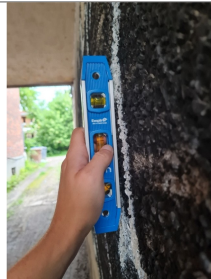
Photo 8: Laneway wall plumbness.
