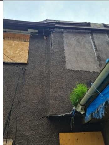
Photo 37: Stucco cracking and shifting visible on addition.
