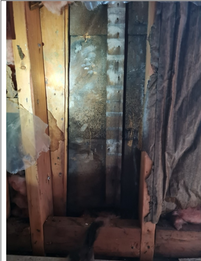
Photo 18: Exposed exterior wall showing signs of water damage on first floor at the front (South) wall of the building.
