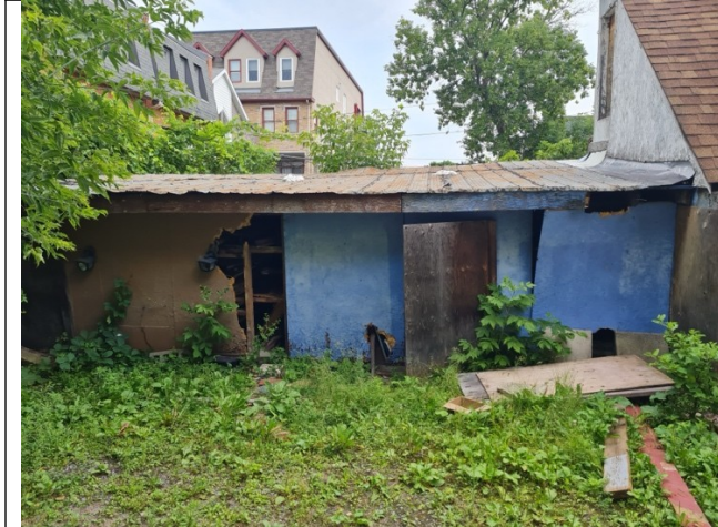
Photo 30: Certain pieces of wooden wall are broken/missing. Shed is leaning, roof slope is curved.
