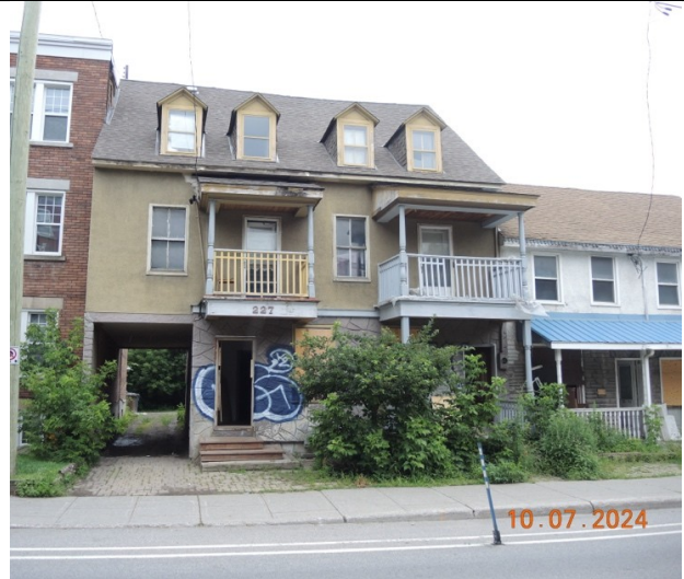
Photo 27: Roof line shows signs of sagging near the middle of the roof.
