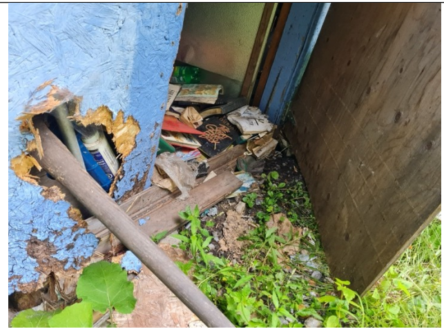
Photo 33: Visible damage to exterior walls of the shed.
