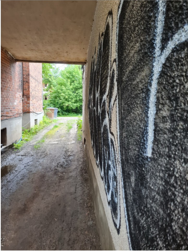
Photo 9: Bulging of laneway wall.
