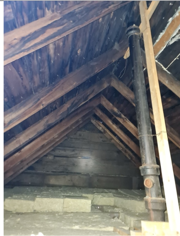
Photo 29: East gable end wall in attic.
