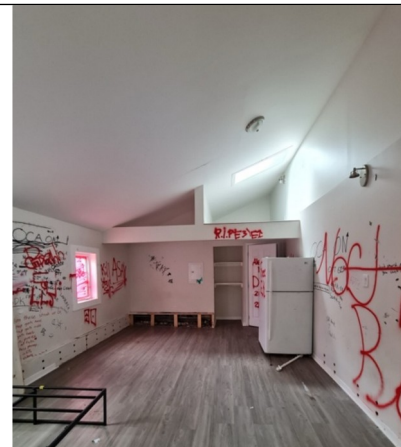
Photo 21: Small bulge in drywall.
