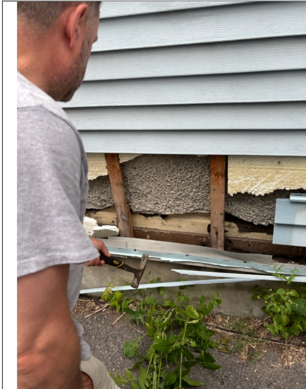
Photo 4: Siding has been applied on top of existing stucco and original wood siding.
