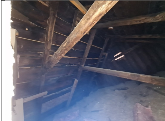
Photo 22: Roof structural elements showing signs of decay and moisture. Daylight observed from inside the attic.
