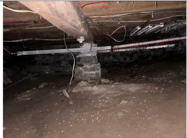
Photo 9: Deterioration of masonry pier.
