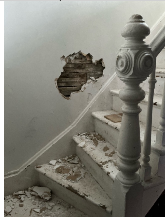
Photo 14: Exposed Lath showing signs of moisture damage.
