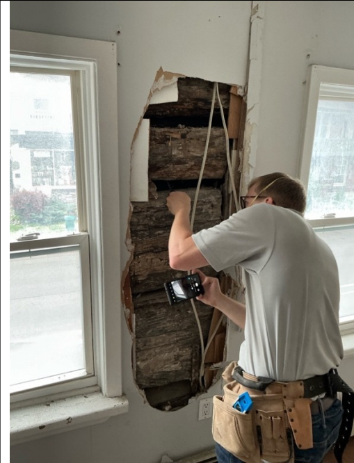
Photo 12: Rot in exterior South wall on second storey.
