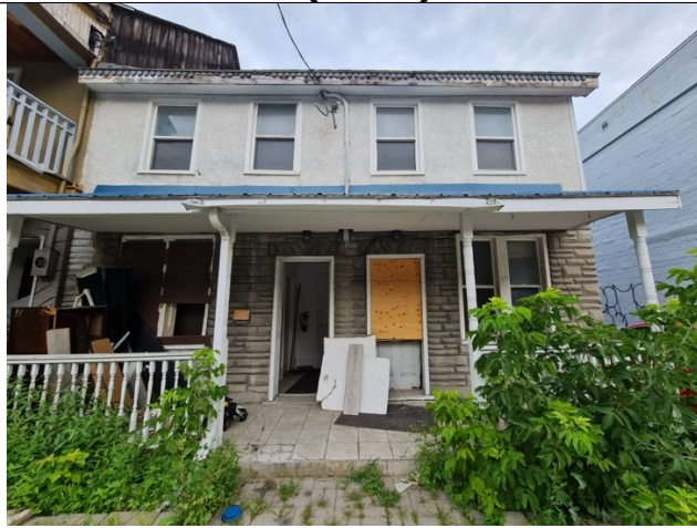
Photo 1: Porch roof no longer appears level.
