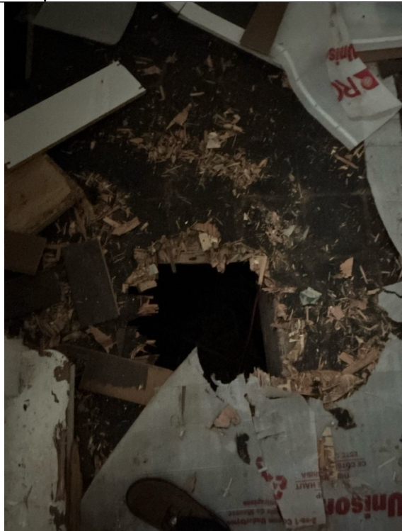
Photo 15: Hole in floor down to crawlspace. Rot is present.
