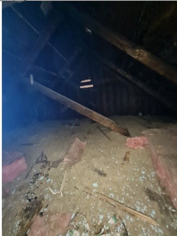
Photo 24: Rafter-tie is disconnected from rafter. End where previously connected has dark staining.
