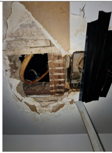
Photo 17: Hole in ceiling. Showing signs of water damage.
