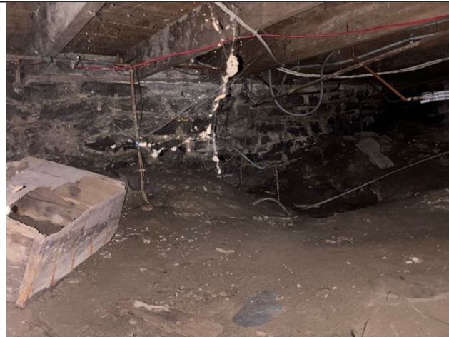
Photo 8: Water staining on joists and wet foundation wall.
