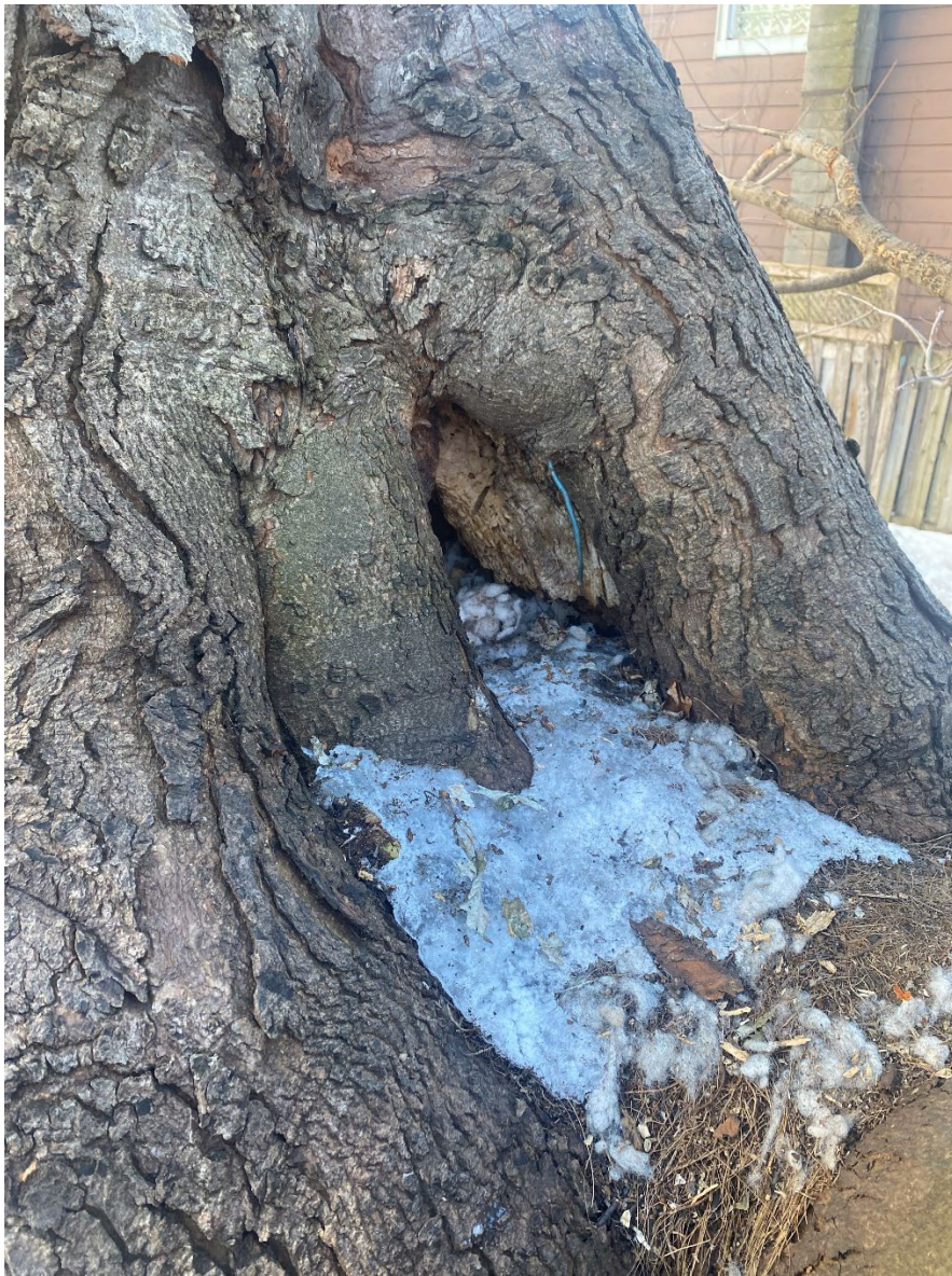
Figure 4: Decay in the main junction of the large branch leaning over the subject property
