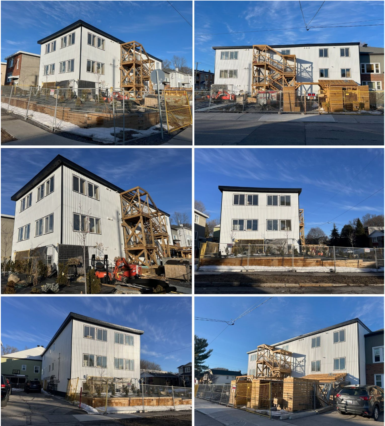
Figure 18: Site photos taken March 17th, 2025. Temporary wooden structures for construction to be removed.
