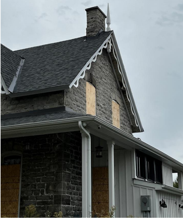
Fire damage under eaves, City of Ottawa, 2025
