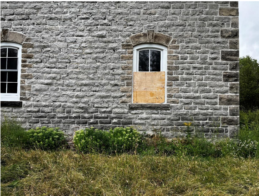
Fire damage at side windows, discoloration above basement level, City of Ottawa, 2025
