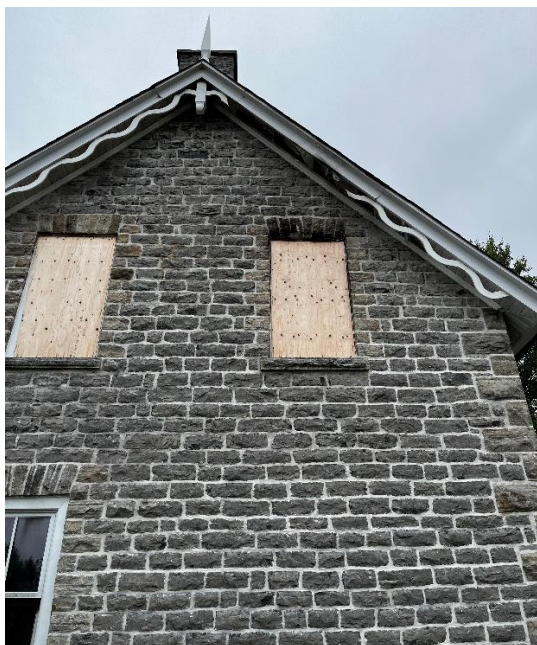
Fire damage at rear second storey windows, City of Ottawa, 2025
