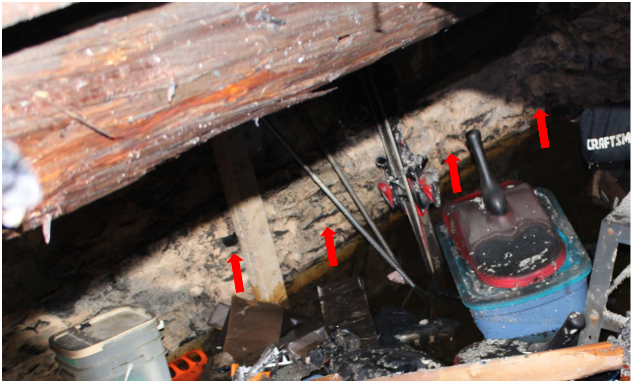
Photograph 06 – South Foundation Wall – Taken by Pario on April 14, 2025. – Degraded Lime Mortar (Red Arrows).
