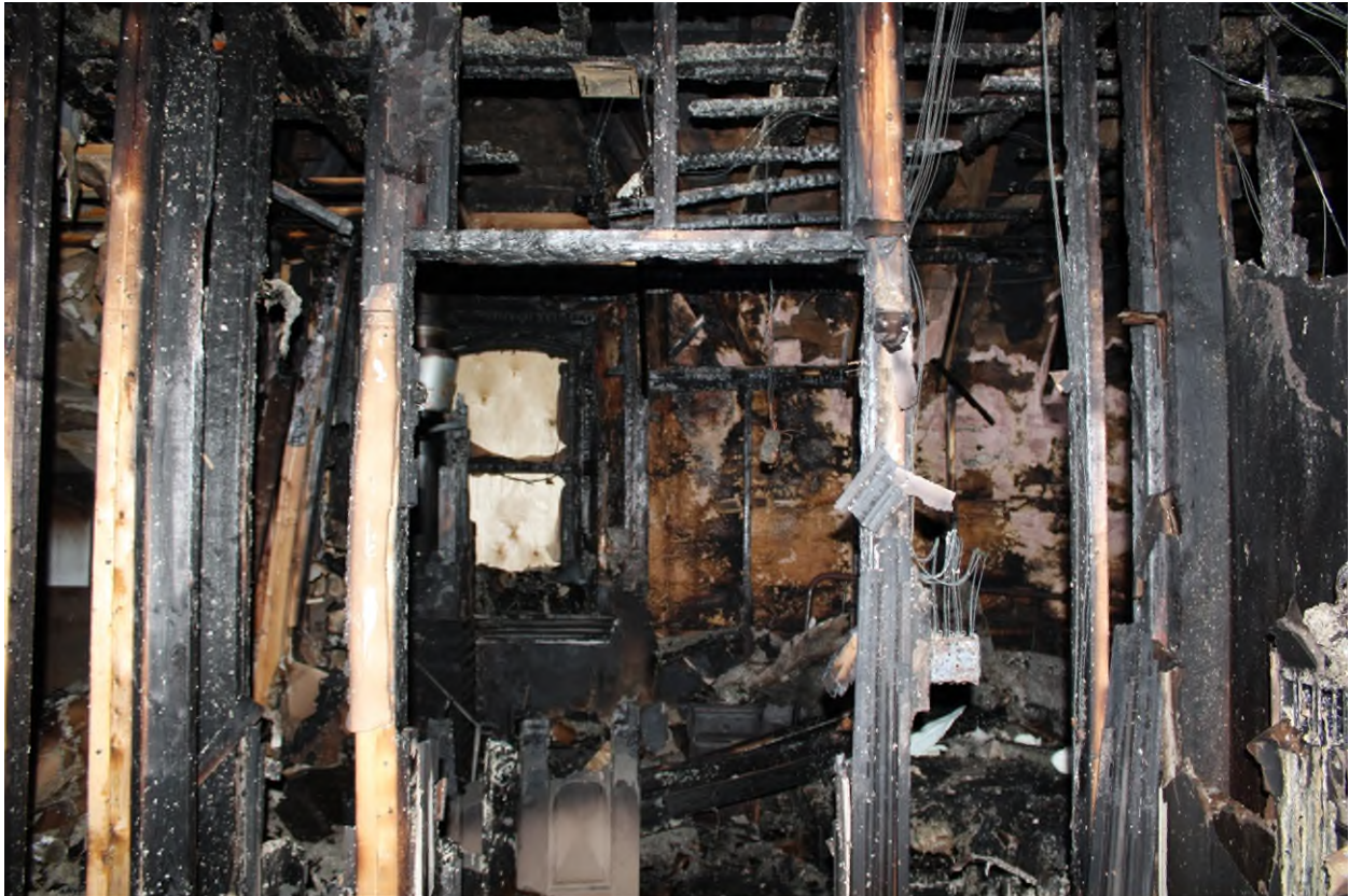
Photograph 14 – View Looking at Fire Damaged Wall Assemblies (Second Floor) – Taken by Pario on April 14, 2025
