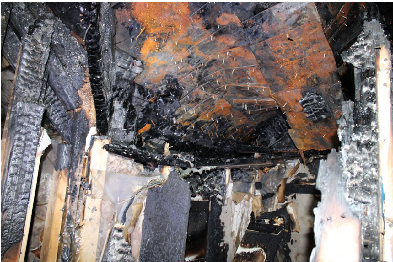
Photograph 12 – View Looking at Fire Damaged Roof Assembly (Second Floor) – Taken by Pario on April 14, 2025.
