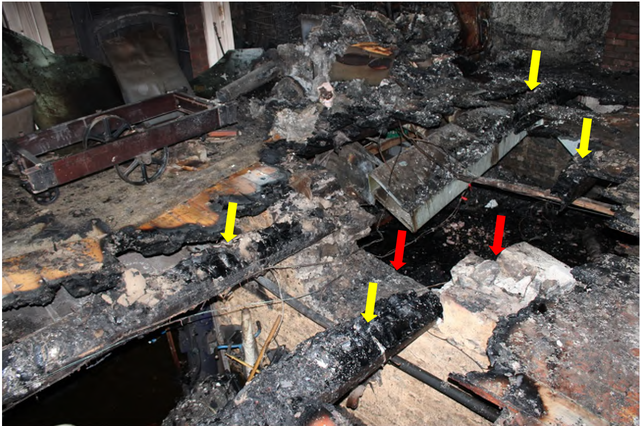
Photograph 05 – Main Floor West Side – Taken by Pario on April 14, 2025. – Damaged Stone & Mortar Foundation (Red Arrows) – Damaged Timber Floor Beams (Yellow Arrows).
