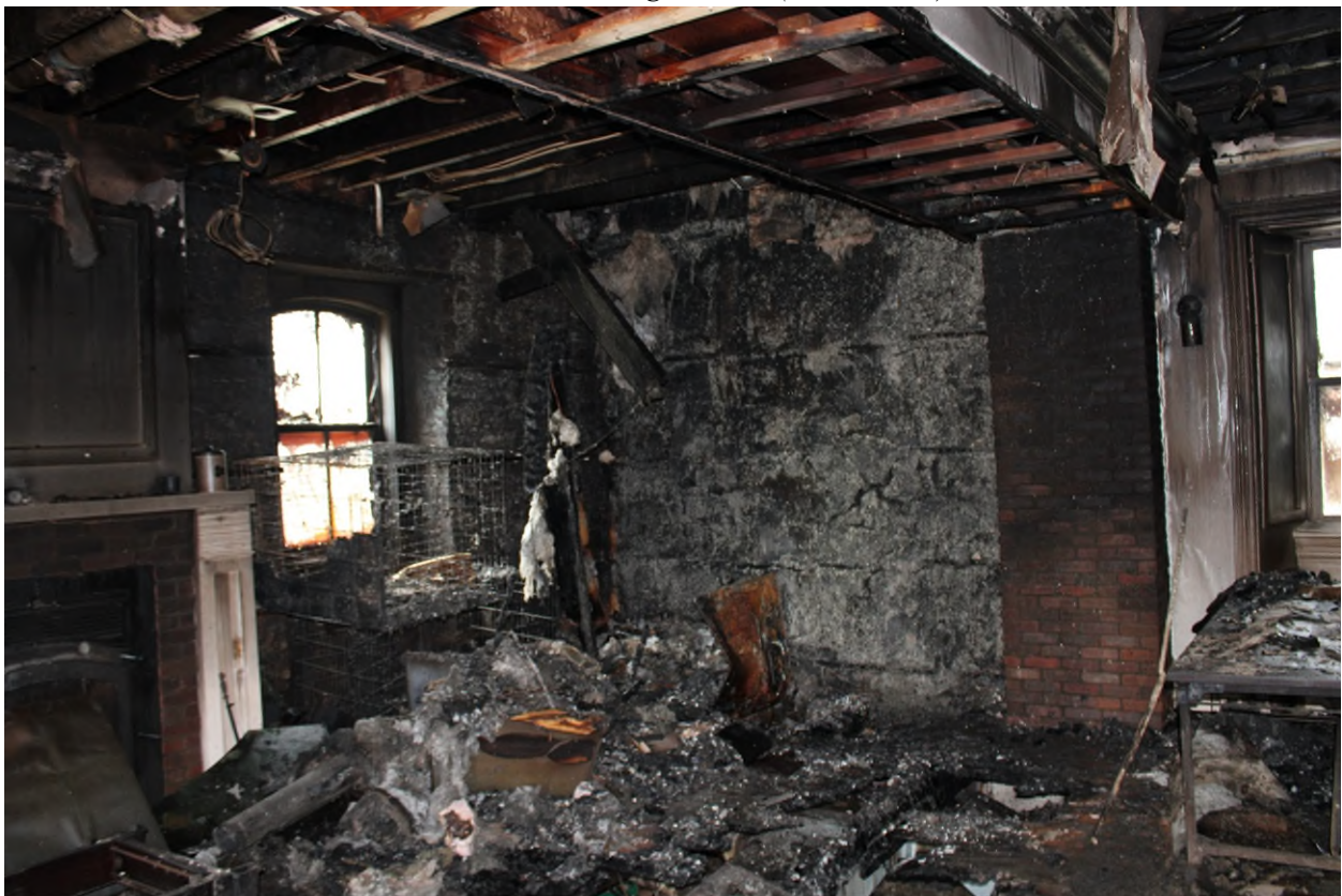
Photograph 08 – View Looking Northwest at Fire Damages (Main Floor) – Taken by Pario on April 14, 2025.
