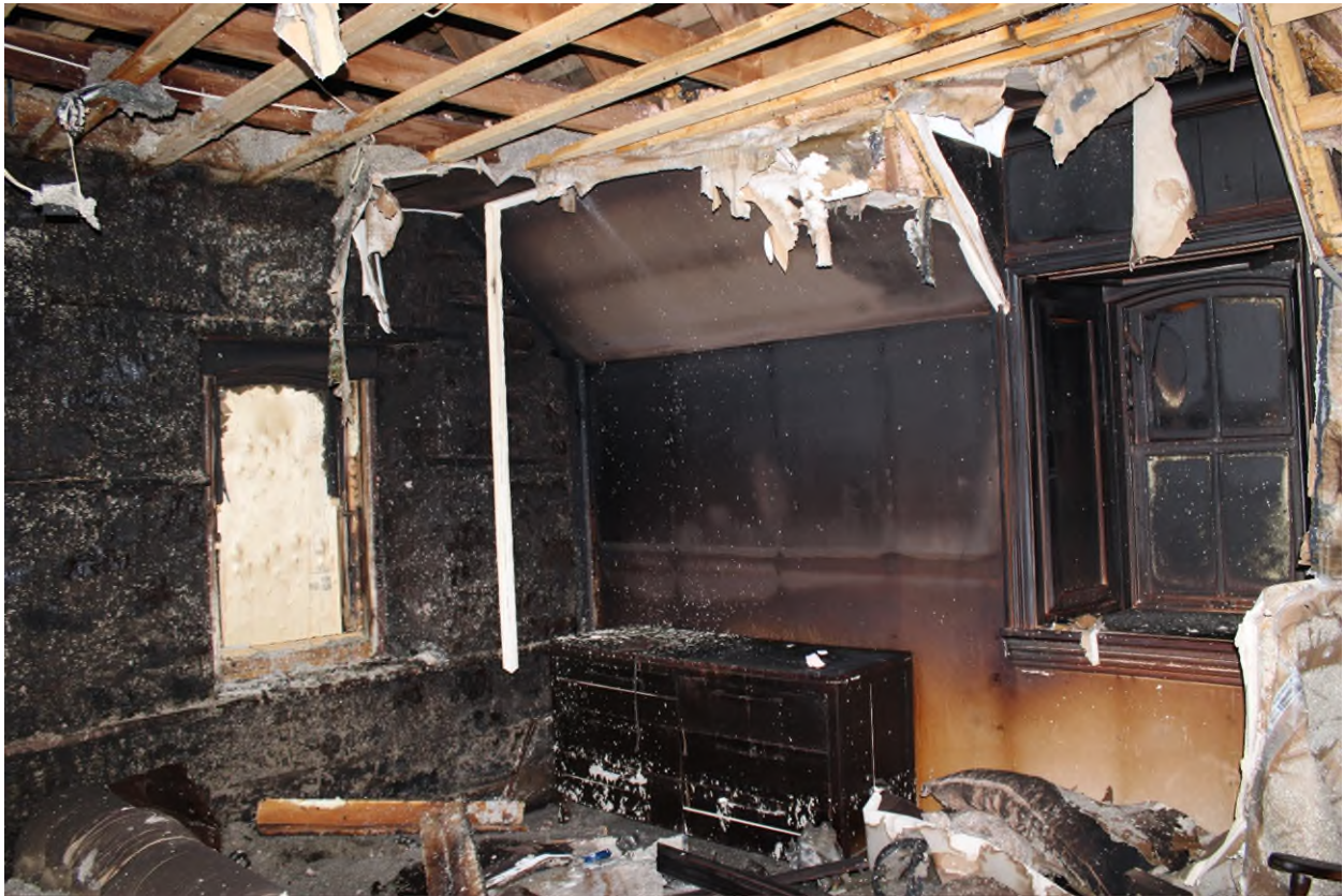
Photograph 11 – View Looking at Fire Damages (Second Floor) – Taken by Pario on April 14, 2025.
