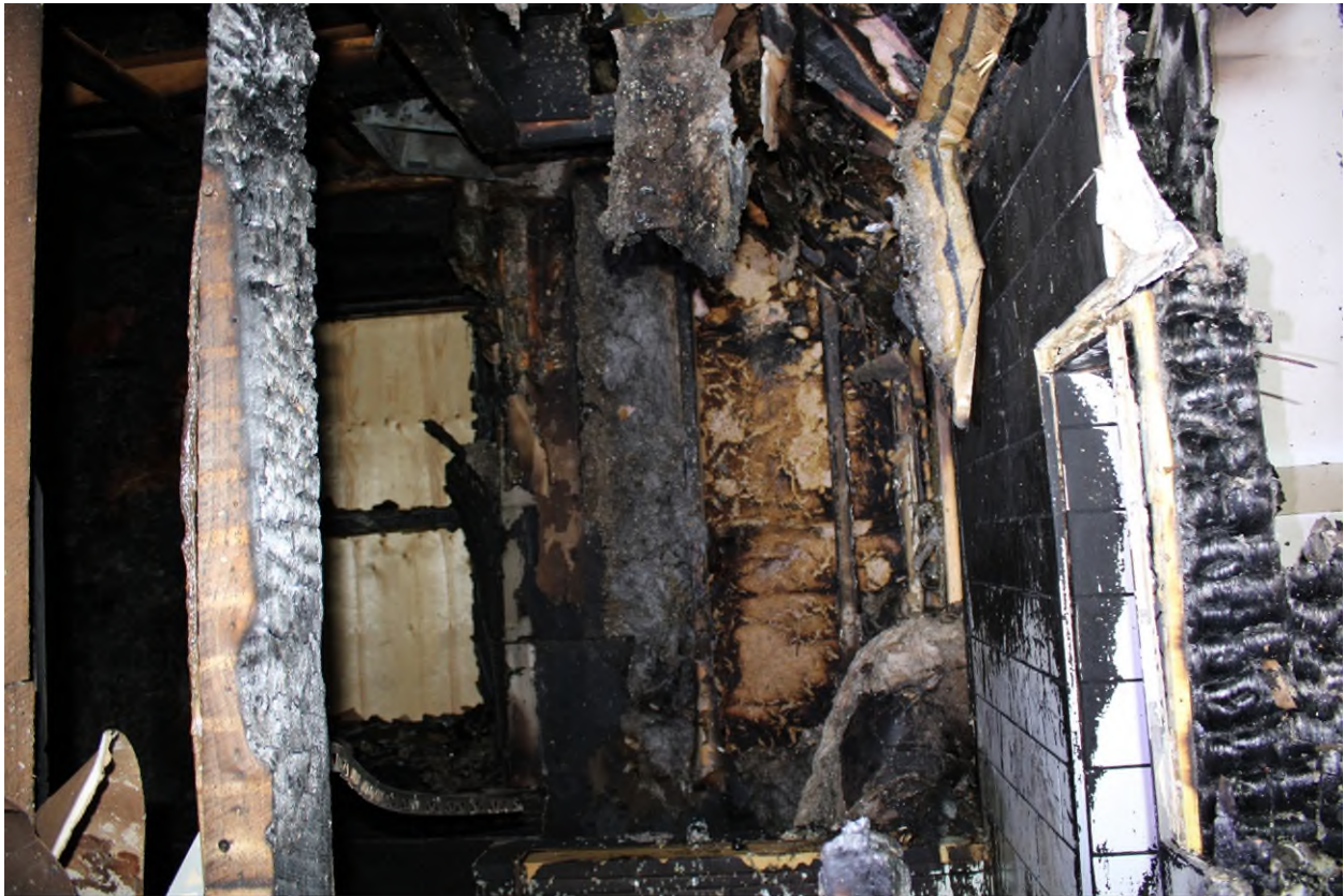
Photograph 13 – View Looking at Fire Damaged Wall Assemblies (Second Floor) – Taken by Pario on April 14, 2025.
