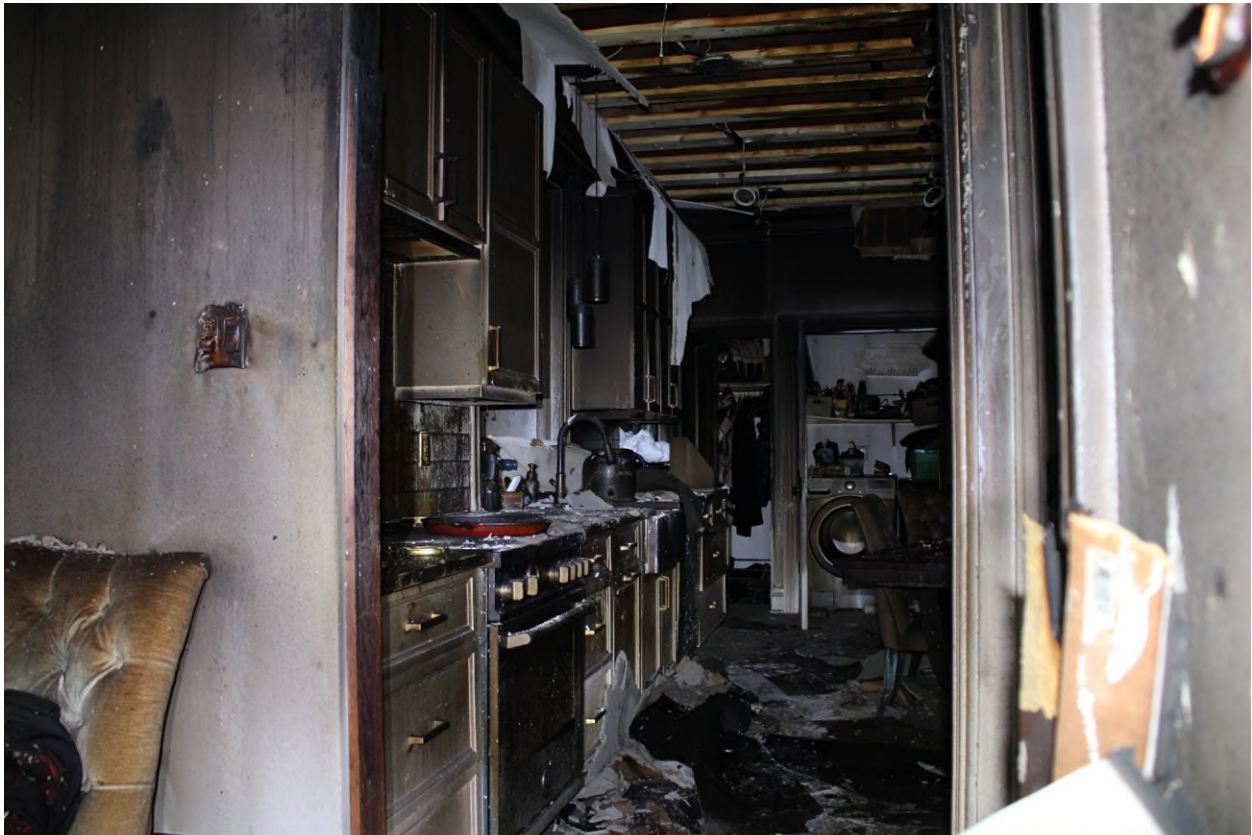
Photograph 09 - View Looking East at Fire Damages (Main Floor) – Taken by Pario on April 14, 2025.
