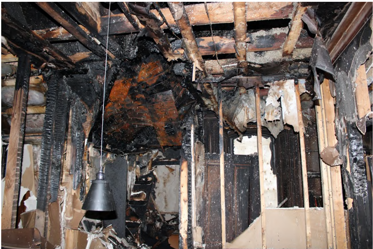
Photograph 10 - View Looking at Fire Damages (Second Floor) – Taken by Pario on April 14, 2025.
